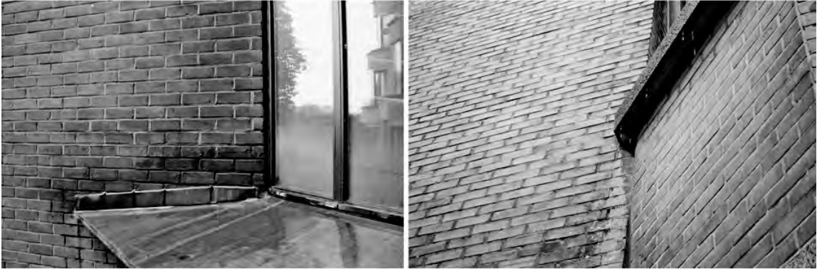
Figure 16.8 Rainwater runoff and missing sill step below the window frames
