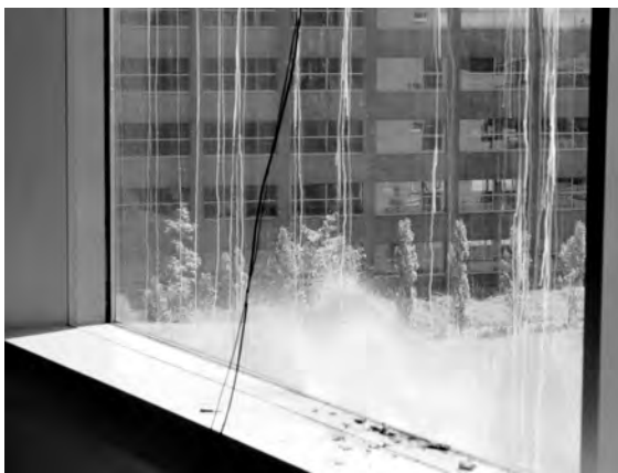
Figure 16.9 Dripping water and runoff along the inside face of the windows
