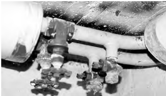
Figure 11.4 Uninsulated isolation valves
