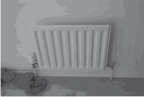
Figure 5.5 Radiator in a low-energy home
