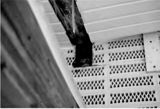
Figure 16.3 Swimming pool: Wooden roof girder collapsed by fungal attack
