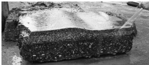
Figure 14. Forensics on rutted SMA pavement on US-231.
