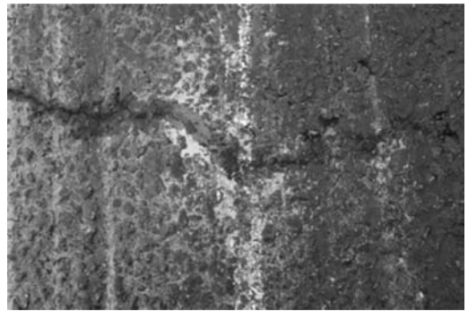
Figure 5. Close-up view of transverse crack on rubberized asphalt.
