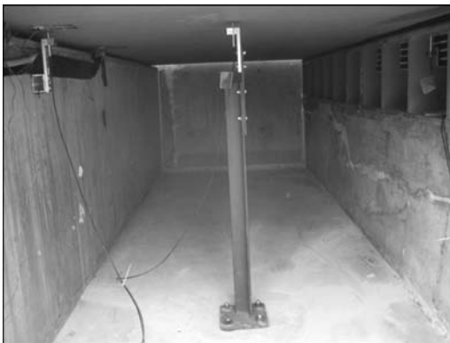
Figure 9. General view of instruments under the joint.
