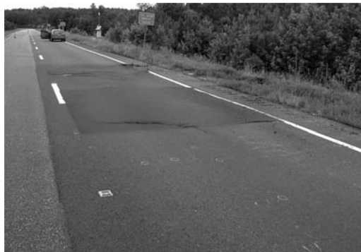
Figure 9. Photo of failed conventional rehabilitation
