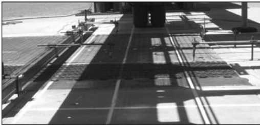
Figure 8. General view of instruments on top of joint.
