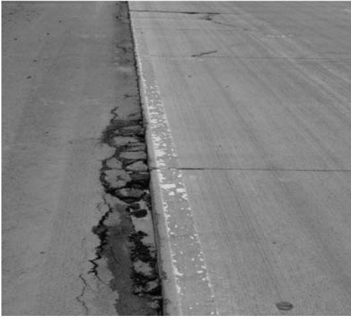
Figure 6. Standing water in deteriorated shoulder of Cell 513.
