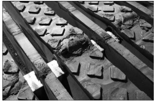
Figure 25a. Close-up view of damage to Trelleborg unit.
