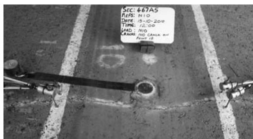
Figure 11. Shrinkage crack at Station 12 prior to trafficking.
