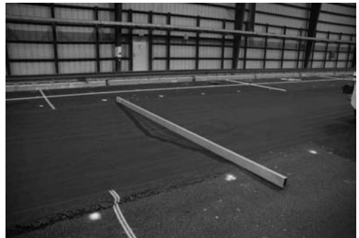
Figure 4. Pavement failure in the east end of the MRC rubblized test section.
