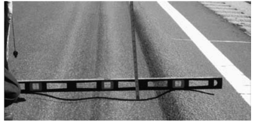
Figure 3. Significant rutting in test section with low QC air voids.
