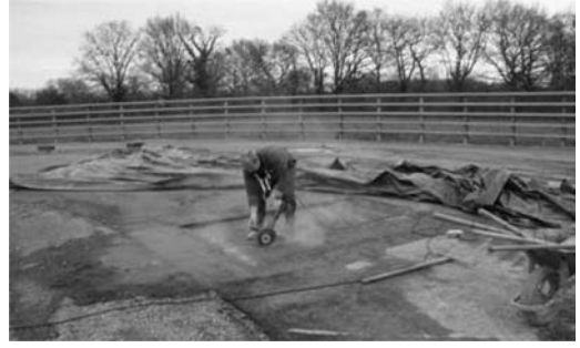
Figure 4. Sawing of a transverse vertical crack inside the fiber reinforced cement concrete layer.
