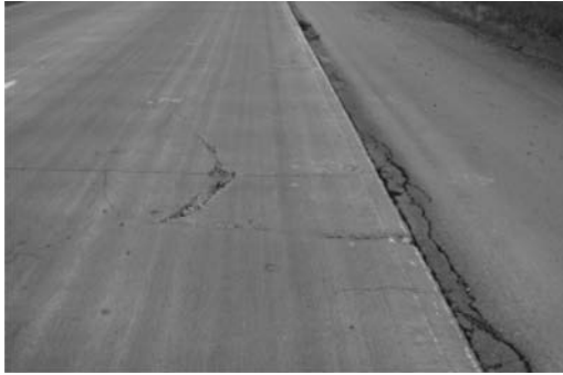
Figure 3. Cracking in area of embedded sensors in Cell 513. Note condition of adjacent shoulder.
