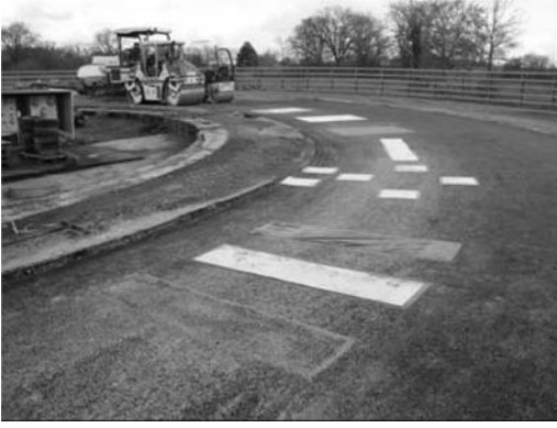
Figure 2. Interface defects before wearing course construction.
