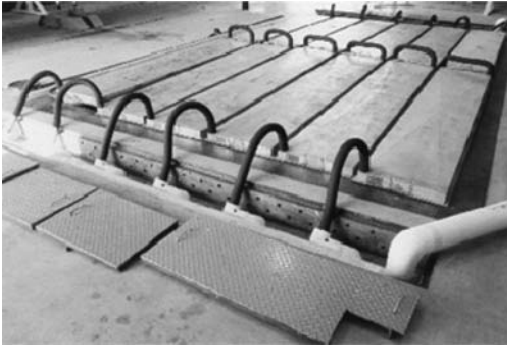
Figure 6. Surface heat exchangers.
