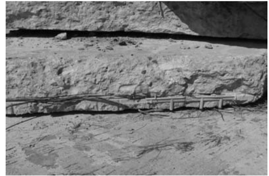
Figure 5. Embedded sensor wires and supports along crack in Cell 513.
