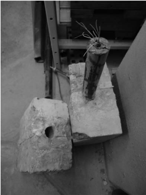
Figure 21. Dowel bar removed from the joint socket.
