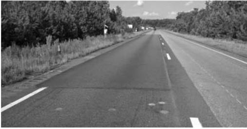
Figure 10. High polymer rehabilitation after traffic surpassed original failure.
