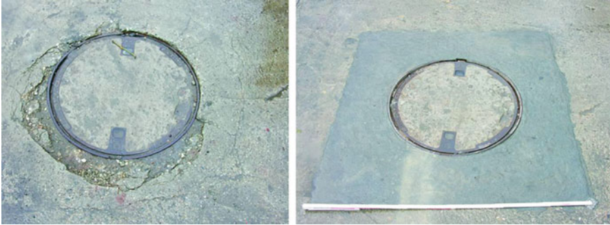
Fig. 3.25 Concrete surface in the vicinity of a sewer before repair ( left ) and 4.5 month after repair ( right ) [19]
