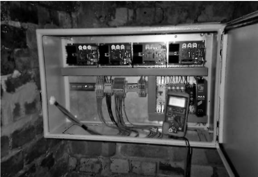
Figure 11.2 A simple manual impressed current cathodic protection power supply with four zones adjusted by the potentiostats at the top of the cabinet.
