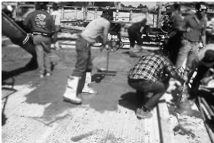
Figure 5.1 Early application of a mesh and overlay anode system on a U.S. bridge deck.
