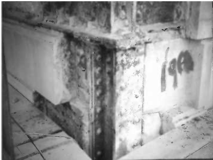
Figure 2.12 Typical corrosion of steel framing from twentieth century.
