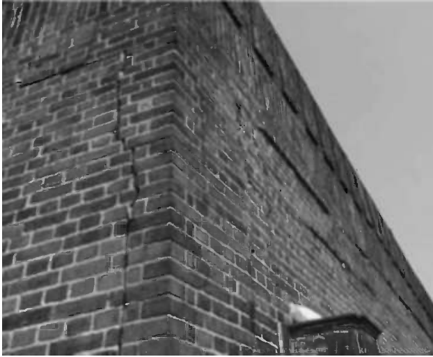
Figure 8.1 Vertical cracking caused by corrosion of the steel frame columns on a large, 1930s built brick building.
