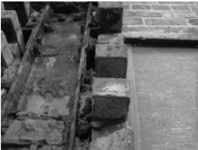
Figure 2.15 Damage to a vertical brick column due to corrosion and expansion of the steel frame.
