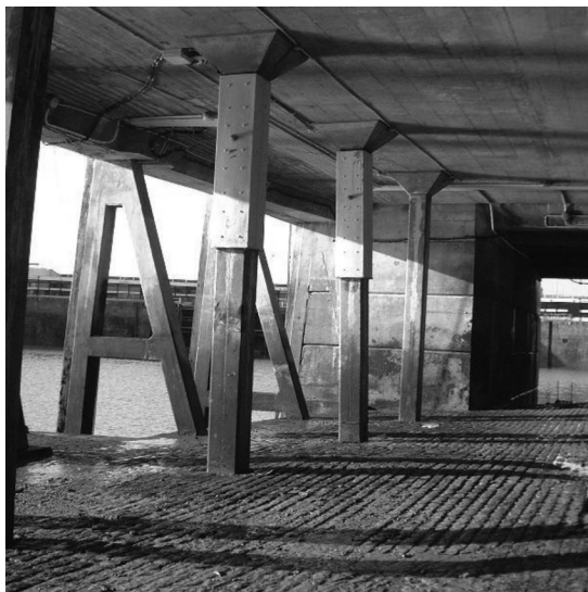
Figure 5.4 A jacketed zinc galvanic anode system applied to columns on a jetty in the Channel Islands, United Kingdom.
