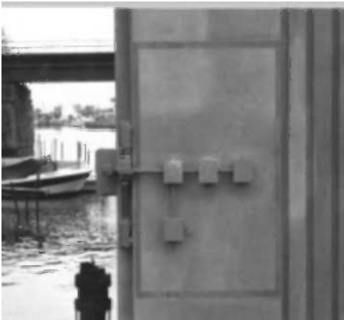
Figure 11.11 A window for current and reference electrode potential monitoring in a Corrospray™ Al-Zn-In thermal sprayed anode system on a marine bridge. (From Daily, S. F. and Green, W., Galvanic cathodic protection of reinforced and pre-stressed concrete using CORROSPRAY™ a thermally sprayed aluminium alloy, Corrpro technical Library paper CP-51. 2007.)
