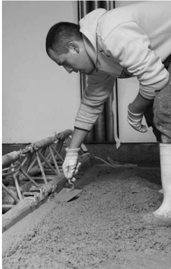
Figure 12.10 Casting of the PCC onto the floors to embed the anode mesh.
