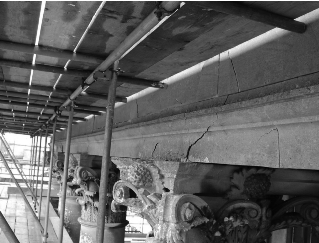
Figure 2.3 Typical damage to the original stonework of the architrave at Dodington House caused by water ingress and corrosion of embedded cramps.
