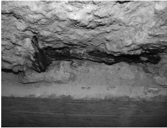
Figure 12.18 Corrosion of pre-stressing wires in precast beam.
