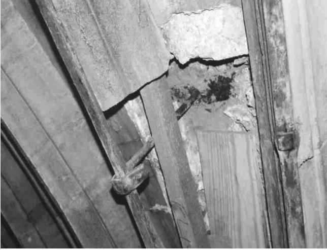
Figure 2.5 Damage to the fourteenth-century fan vault at Sherborne Abbey due to corrosion of the wrought iron reinforcements.
