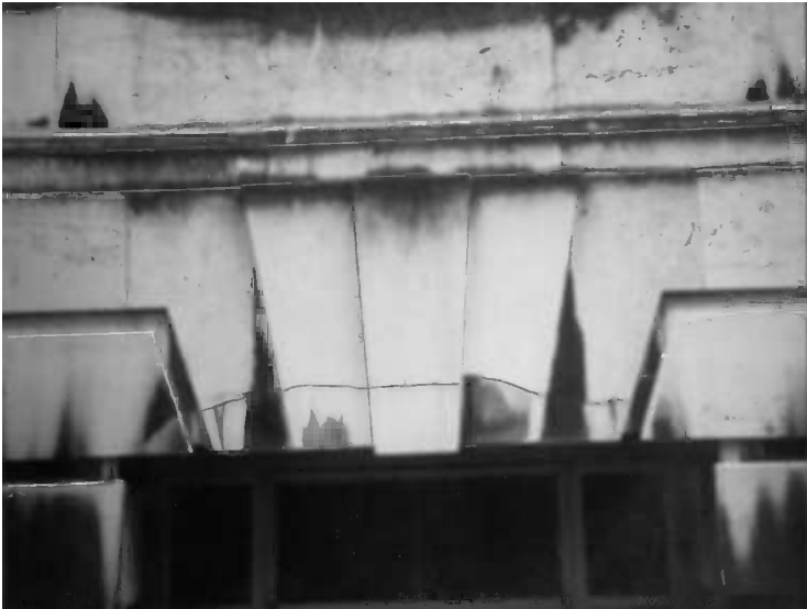
Figure 2.10 Practical example of the damage to steel framed construction as illustrated in Figure 2.9.
