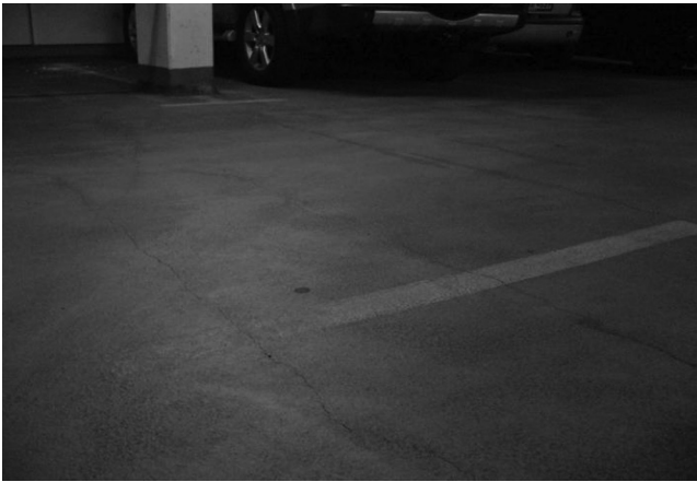
Figure 12.3 Cracks on the floor slabs in the car park.
