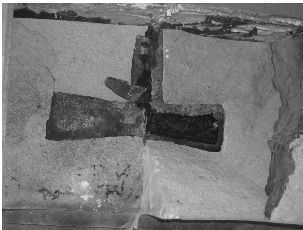
Figure 2.1 Cramp with incomplete leaded surround at Dodington House.
