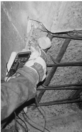
Figure 5.6 A galvanic anode in a patch repair to provide local protection around the repair and prevent the ‘incipient anode’ effect of corrosion around a repair.
