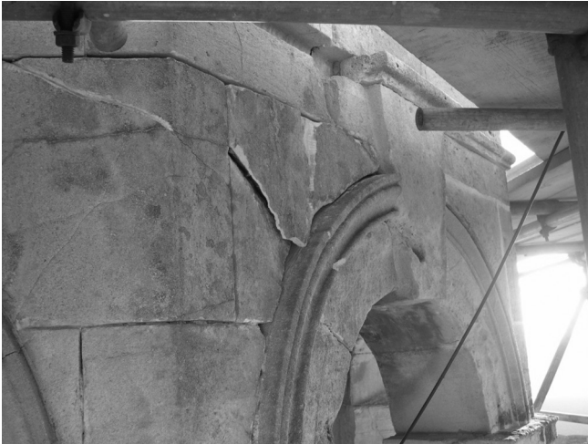
Figure 2.4 Damage to stonework at Great Witley church, Worcester, due to corroding cramps.
