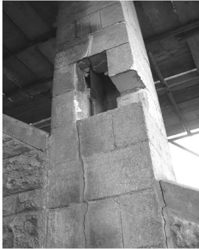
Figure 2.14 Cracking of the vertical pillars to a cricket pavilion at Downside Abbey and School, Somerset.
