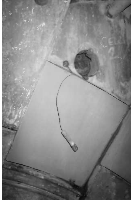
Figure 8.3 Damaged stones have been replaced before the cathodic protection contractor arriving on-site. A core hole is therefore required to make a connection to the steel and to install a reference electrode.
