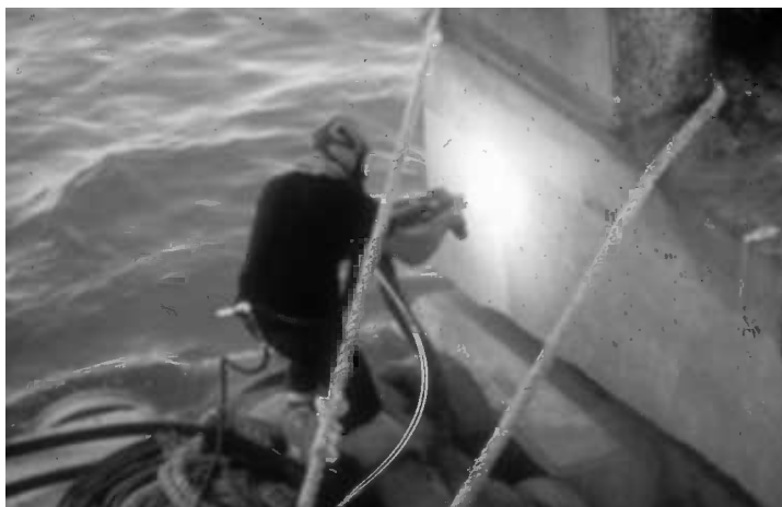
Figure 5.5 Thermal-sprayed zinc being applied to a bridge substructure in the Florida Keys in the 1990s.
