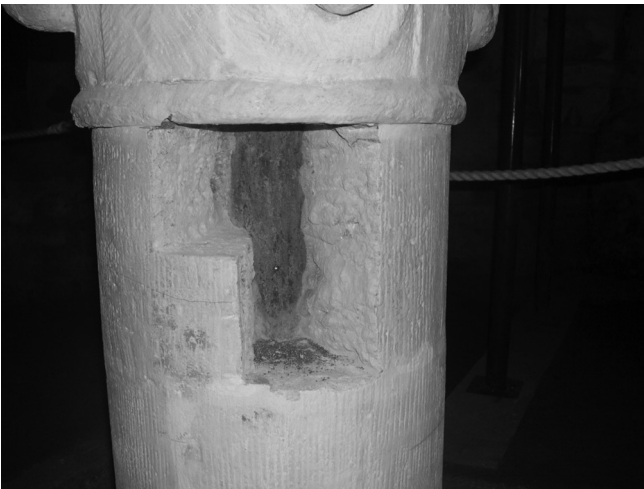
Figure 2.6 Damage to the eleventh-century Saxon stones in the vault at Gloucester Cathedral due to corrosion of the internal steel cores, which had been installed in the twentieth century.
