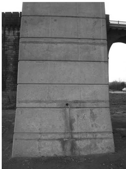
Figure 12.16 Egress of excess moisture.
