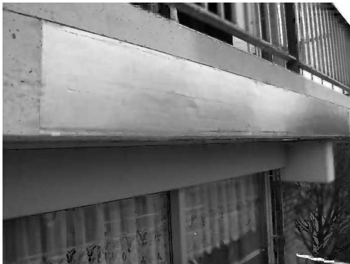
Figure 5.7 Zinc hydrogel adhesive galvanic anode applied to a balcony fascia before the application of a protective/sealing coat.
