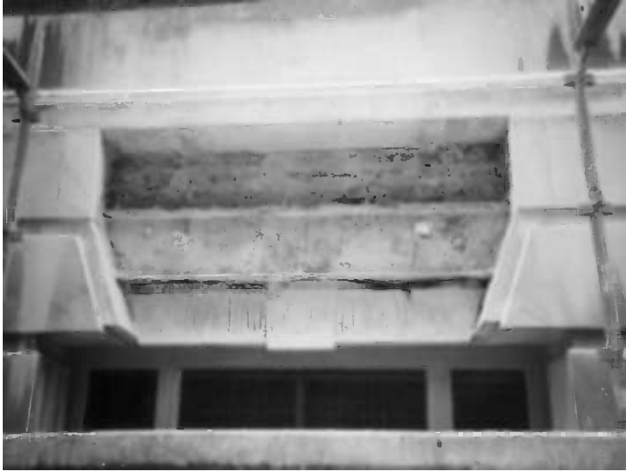
Figure 2.11 Opening up the steel framed construction to reveal the corroding steel beam.
