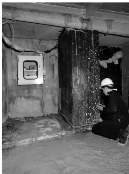
Figure 5.2 A conductive coating anode applied in an industrial plant in Australia in the 1990s.
