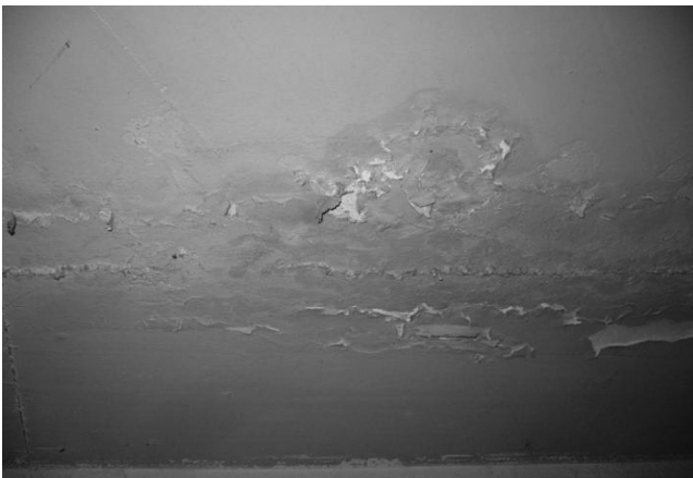
Figure 12.4 Damages and signs of moisture on the ceiling above first basement floor.
