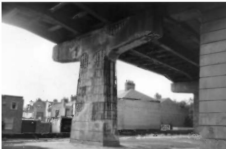
Figure 12.15 Deteriorated approach viaduct pier.
