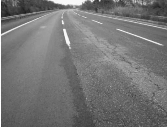
Figure 15.5 Reflective cracking initiated over an old paving joint in a flexible pavement.
