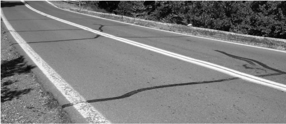
Figure 15.8 Shrinkage cracking, block patterned.
