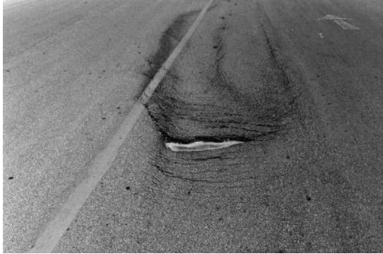
Figure 15.7 Slippage cracking. (From Asphalt Institute, Asphalt in Pavement Preservation and Maintenance , Manual Series No. 16 [MS-16], 4th Edition, Lexington, US: Asphalt Institute, 2009. With permission.)
