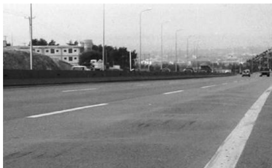
Figure 15.16 Corrugations and shoving.
