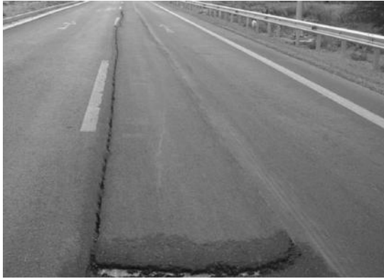
Figure 15.11 Slippage of asphalt overlay over a geotextile.
