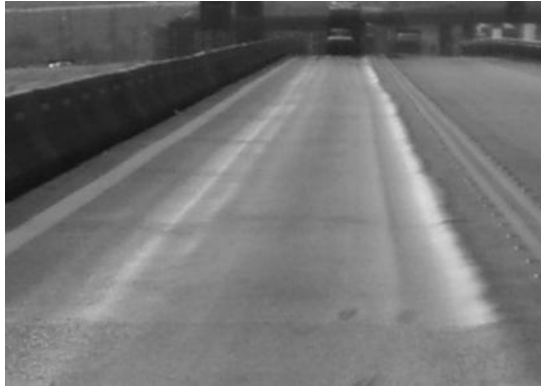
Figure 15.14 Typical rutting quite often formed very early, as shown schematically in Figure 15.12b.
