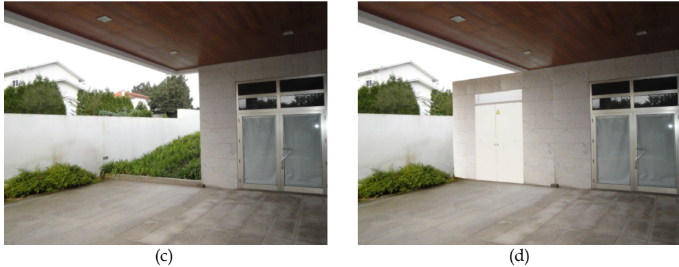
Fig. 12. Landscape integration of transformer stations in relation to structures (a) transformer station built-in a wall; (b) transformer station attached to an existing construction; (c) and (d) transformer station built by extending an existing building.
