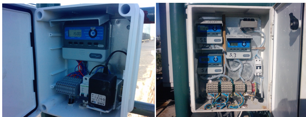
Fig. 3. Control unit panel having 8 Station used in landscape irrigation Systems
