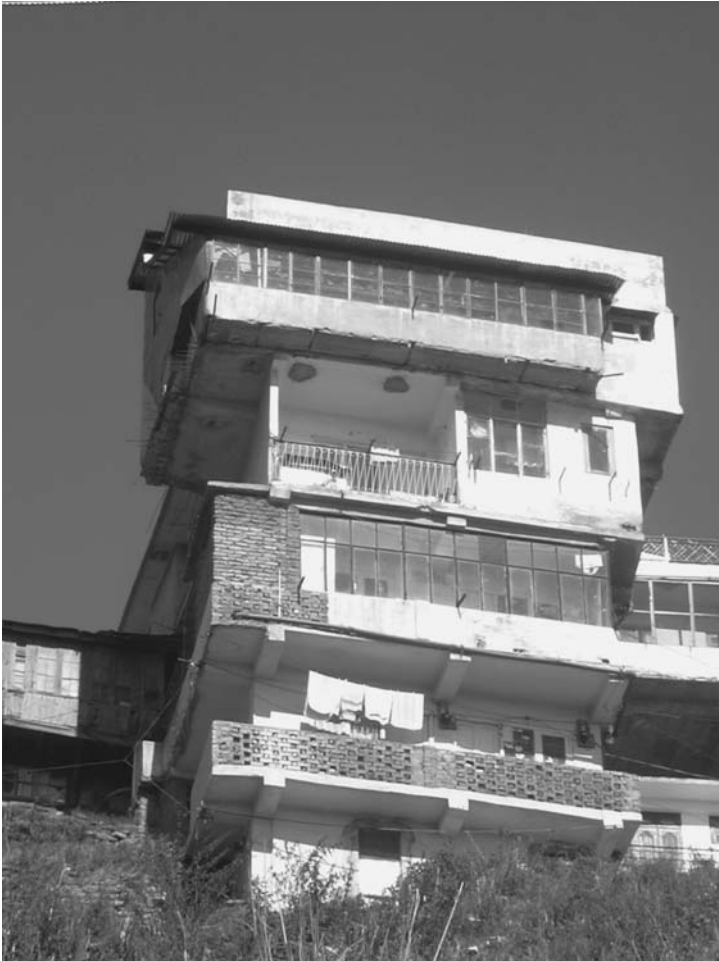
Fig. 2. Poor Building Condition: Issues of Design and Construction Quality.
