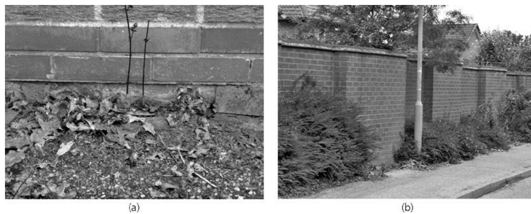
Figure 4.4. (a) Frost failure at the base of a free-standing wall, with moderately frost-resistant bricks. (b) General view of the wall, showing the castellated plan form
