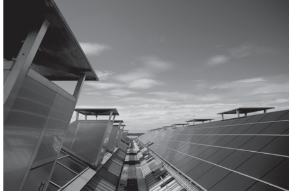
Fig. 6.7 The array of roof cowls and PVs provide shading to the rooflights
