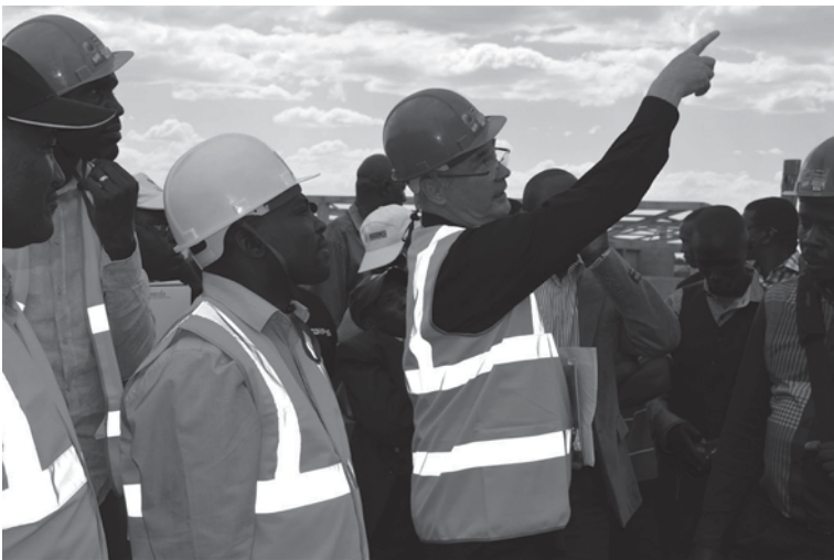
Fig. 12.21 PITCHAfrica Design Director, David Turnbull at the Waterbank Campus construction site with the Governor of Laikipia, discussing cloud formations
