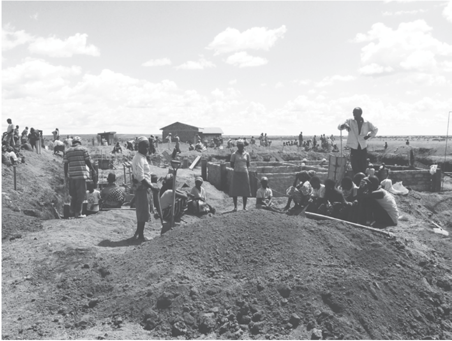
Fig. 12.9 Waterbank School, ‘harambee’ organized by the Zeitz Foundation, engaging the school community, digging the foundations
