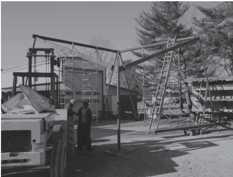
Fig. 12.5 Testing a corner assembly—with Lucien Peebles and Jane Harrison from PITCH Africa
