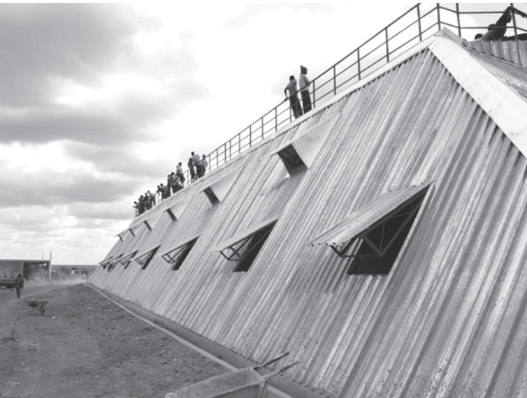
Fig. 12.15 PITCHKenya under construction. Every surface is arranged to maximize rainwater harvesting yields
