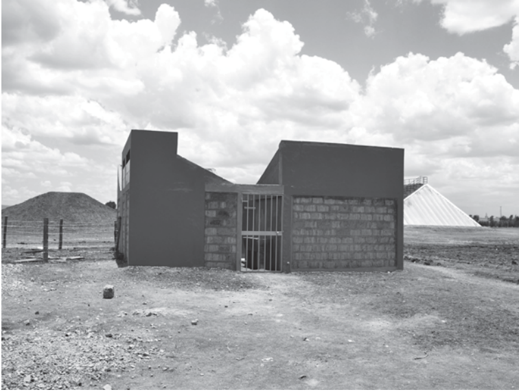
Fig. 12.18 Waterbank Campus Latrines: four blocks in a compact arrangement including open air courts for drying laundry
