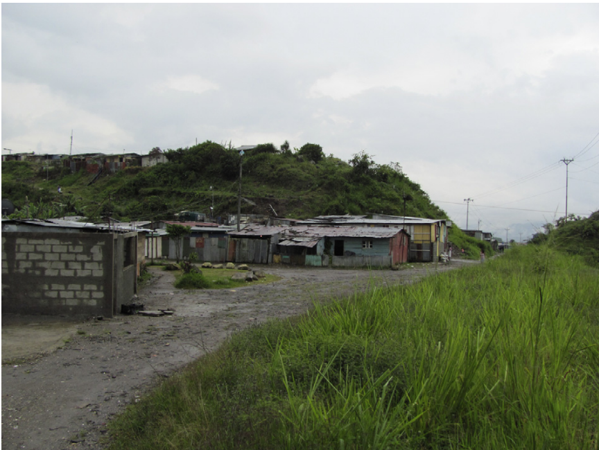
Vulnerable Houses in Illegal Dique Area, Cartago City, Costa Rica. Source: Authors.
