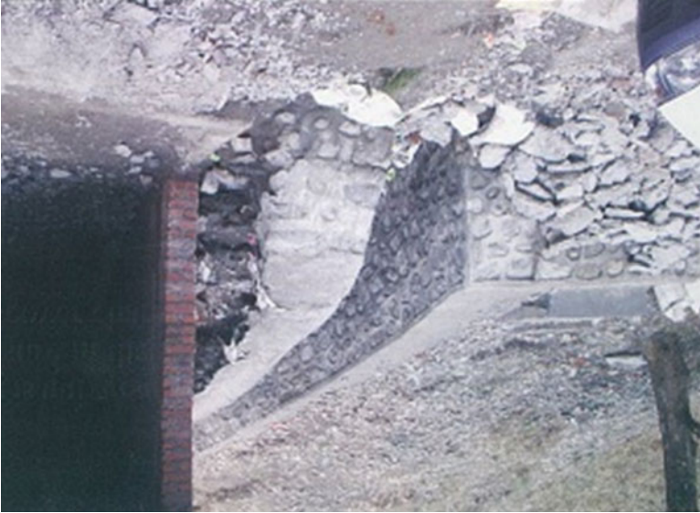
Fig. 13.6 Blockade of drainage by construction (DMMC 2011)
