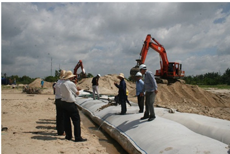
Fig. 19.6 A Stabiplage construction in Loc An, Long Dien district (Source: Department of Technology and Science)
