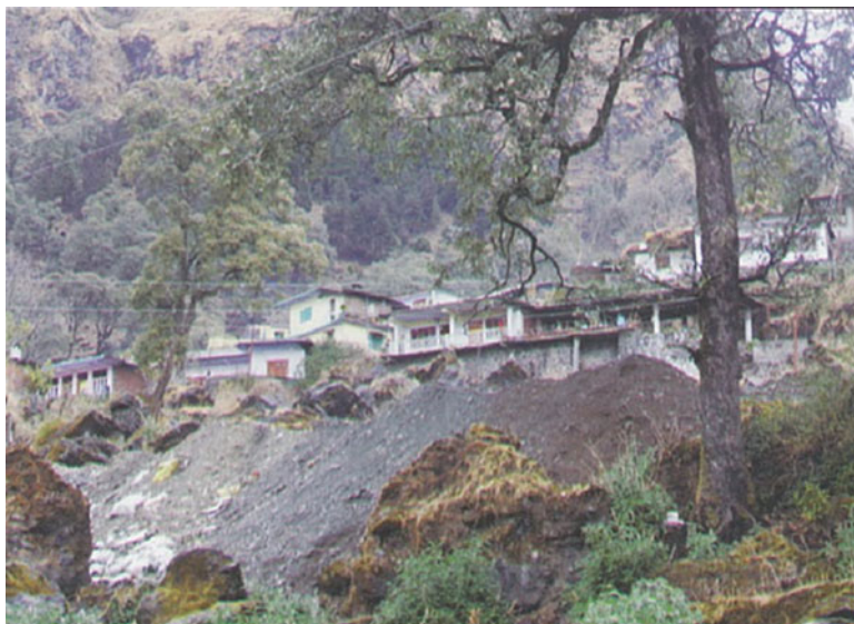
Fig. 13.5 View of indiscriminate disposal of excavated material along the hill slope (DMMC 2011)
