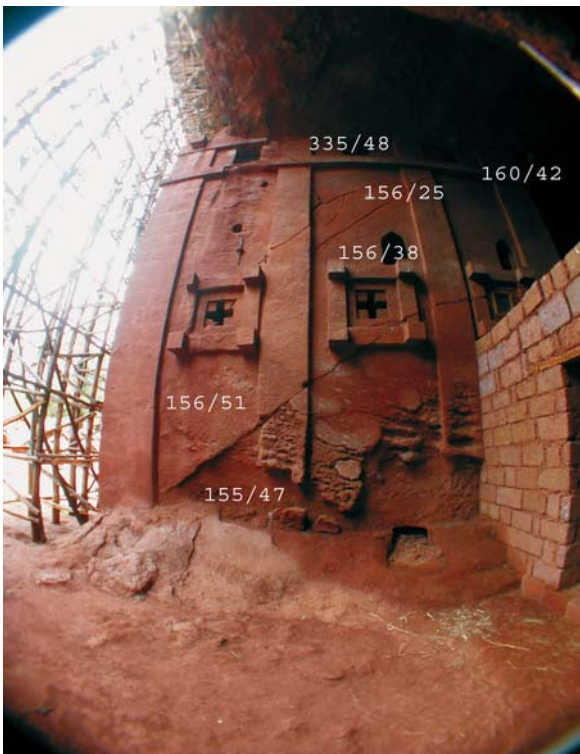
Fig. 26.8. The discontinuities detected on the lateral wall of Bet Aba Libanos; data refers to dip direction and dip
