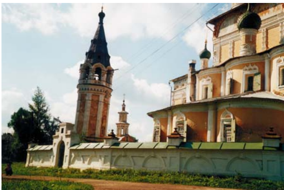
Fig. 46.6. The Resurrection Cathedral (seventeenth century, the town of Tutaev). Wall deformation and tilting of the bell tower
