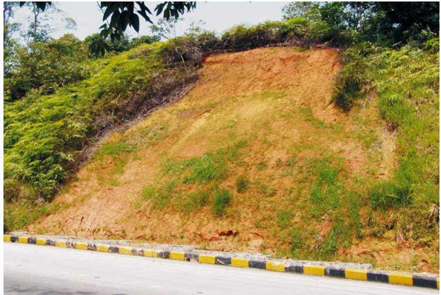
Fig. 24.6. Soil erosion feature at Fraser Hill
