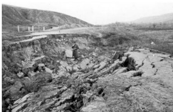
Fig. 3 Slumping and lateral spreading of the road, in Balintesti, near the Vrancea County, after the 1940 earthquake [4]
