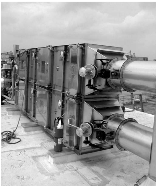
Fig. 34-5 Redundant bag-in/bag-out HEPA filters.
