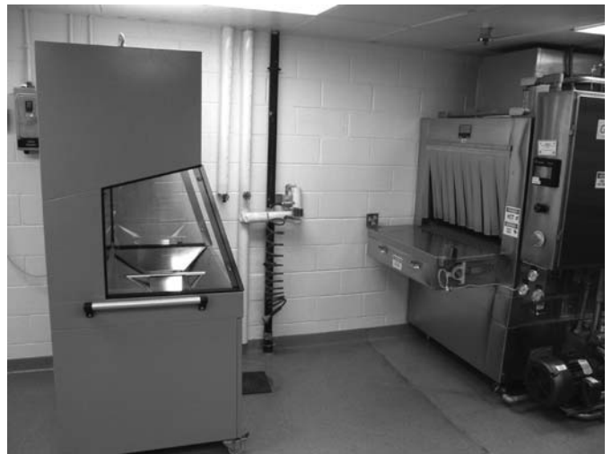
Fig. 31-9 Bedding dumping stations.
