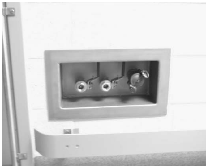
Fig. 25-7 Port for fumigant gas injection.
