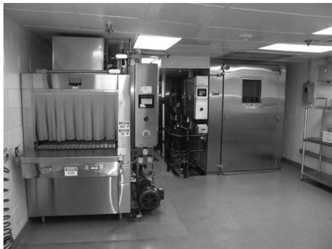
Fig. 31-2 Tunnel and rack-washers.
