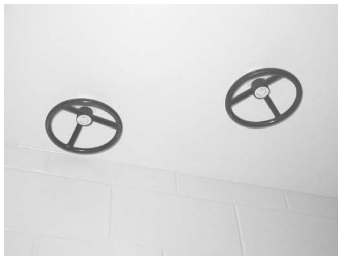
Fig. 25-6 Remote air supply/exhaust damper controls.
