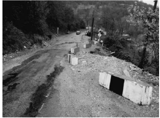
Figure 3. Landslide deformation of the motorway Lazarevskoe – Kirova, km 2 + 800.
