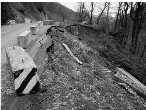
Figure 2. Landslide deformation of the motorway Makopse – Nadjigo, km 5 + 300.
