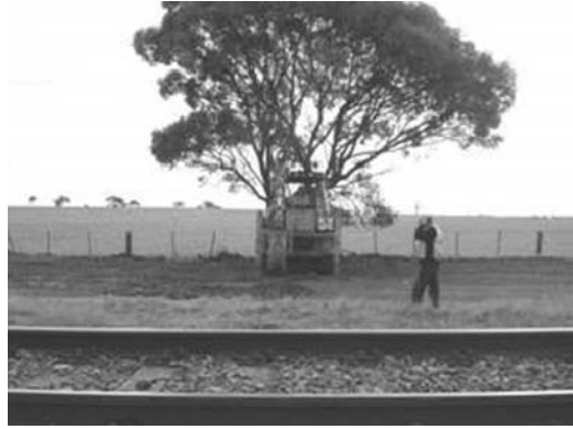
Figure 4. Excavation around a black box tree in western Victoria, Australia for validation of the developed model based on field observations.
