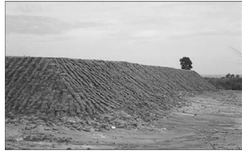
Figure 16. The protection of erosion failure.
