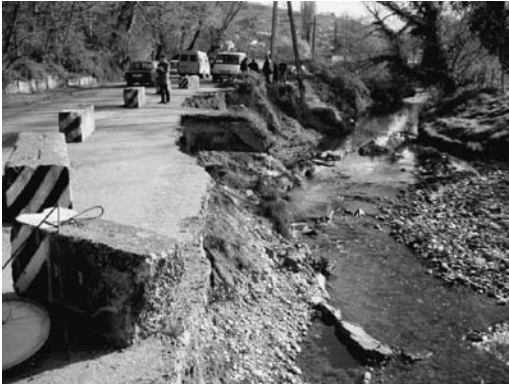
Figure 1. Destroyed site of the motorway Veseloe – Nignyaya Shilovka, km 3 + 690.
