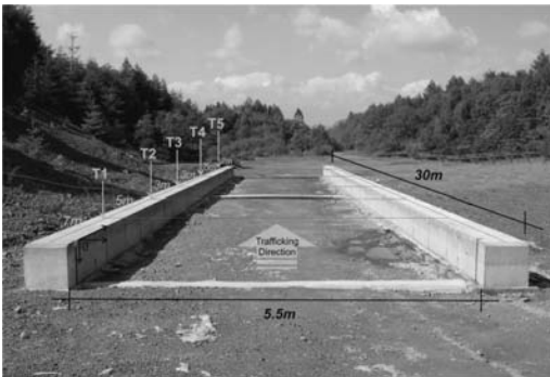
Figure 1. Ringour Testing Facility before construction of the test section with major dimensions indicated and sections chainage.
