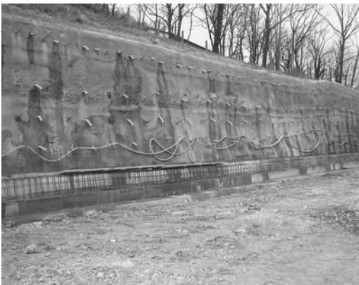
Figure 2. The photo of the cut with applied primary support system, drainage and strip footing.
