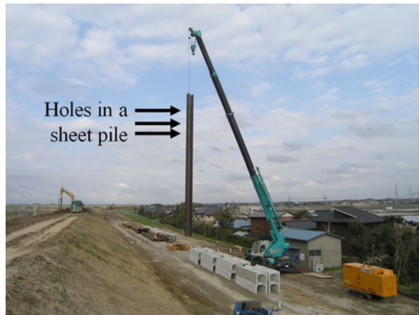
Fig. 6.20 Reconstruction of land side of Tone River levee at Sakae by installing sheet pile walls with holes
