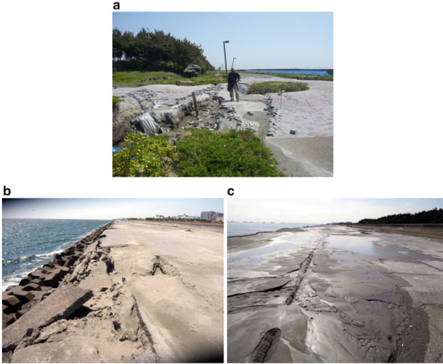
Fig. 4.24 Lateral spreading towards the sea behind the cemetery park at Hinode-8, Urayasu. (a) A depression of the ground inland of the seawall – a view to the east. (b) Damage at the edge of the apron – a view to the west. (c) Sand gushing from a seam of pavement over the apron in front of the seawall – a view to the west
