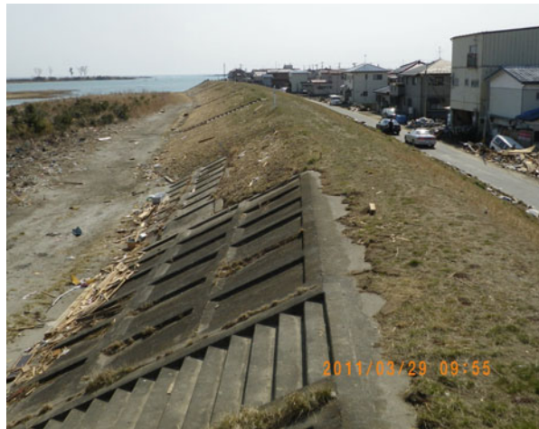
Fig. 6.11 Appearance of the Yuriage Levee of Natori River after the tsunami attack
