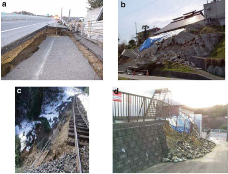
Fig. 12.7 Damage to non-reinforced soil structure during great East Japan earthquake. (a) Subsidence of highway embankment (East Nippon Expressway Company, 2011). (b) Collapse of retaining wall on local road (JC-IGS Technical Committee, 2011). (c) Collapse of retaining wall on railway track (East Japan Railway Company, 2011). (d) Collapse of retaining wall at housing site (Koseki et al. 2011)
