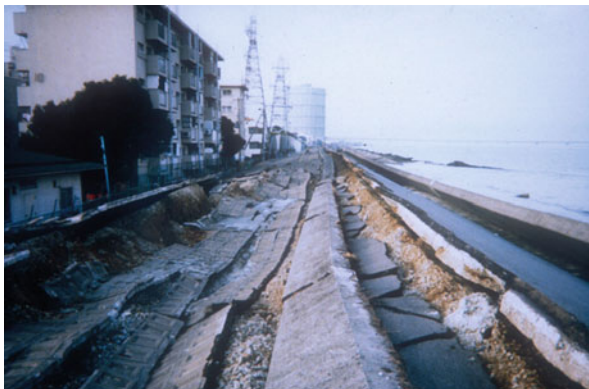
Fig. 6.1 Distorted shape of Yodo River levee after 1995 Kobe earthquake
