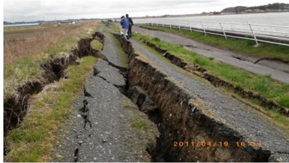
Fig. 6.6 Significant distortion of the Hinuma levee at Shimo-Ishizaki
