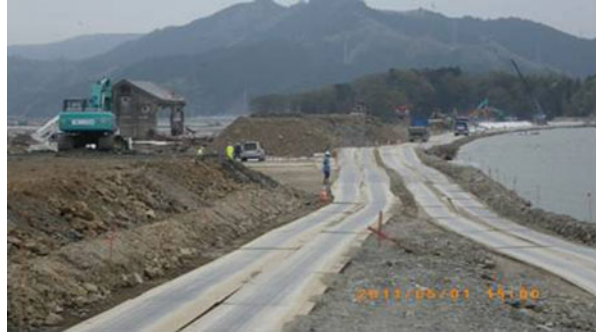
Fig. 6.10 Kitakami River Levee at Kamaya under restoration after total destruction by the tsunami attack
