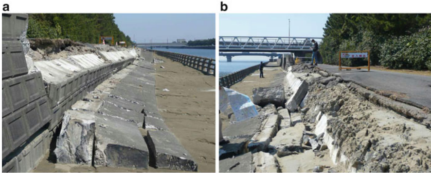
Fig. 4.32 Failure of the walkway wall on the north of the Hanami River. (a) Collapse of the wall north of The Hanami River – viewed from the west. (b) Collapse of the wall north of the Hanami River – viewed from the east to the sea
