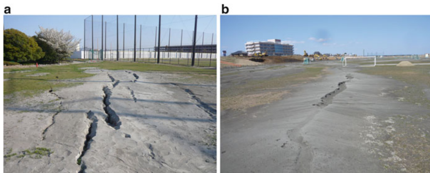
Fig. 4.35 Linear fissures in wide flat ground. (a) Cracks at Sports Park at Urayasu. (b) Cracks on the elevated bed of the Tone River
