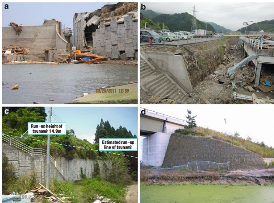
Fig. 12.11 Performance of reinforced soil wall against seismic motion and tsunami action. (a) Case 8: ultimate limit state. (b) Case 9: serviceability limit state. (c) Case 10: no damage. (d) Case 11: no damage (a and c: by courtesy of Dr. Otani: Hirose Co.; b and d: JC-IGS Technical Committee (Dr. Hironaka))
