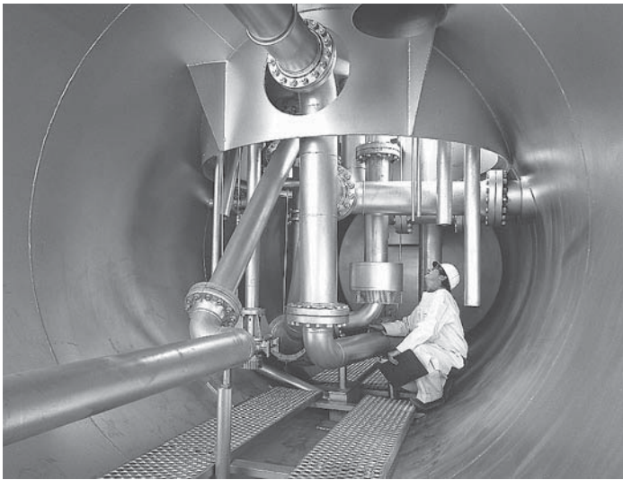
FIGURE 21.6 Piping is a basic part of steam generation power plants. Courtesy Washington Public Power Supply System
