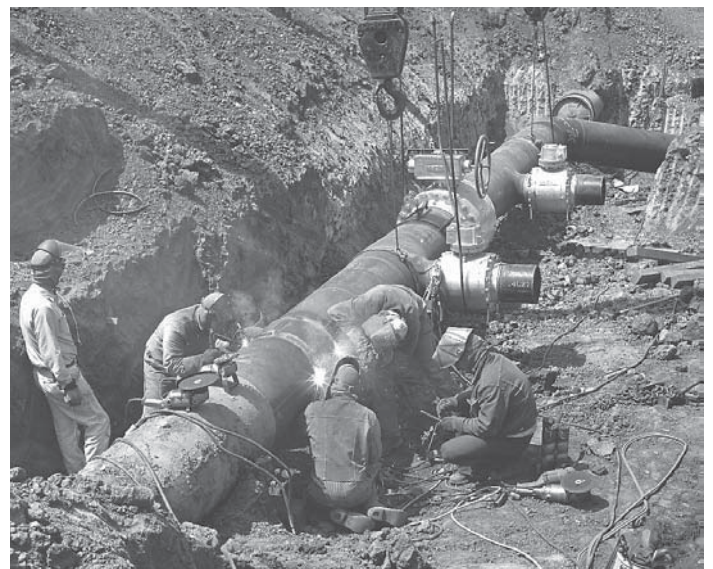
FIGURE 21.4 Underground piping supplies natural gas for homes and industries. Courtesy Pacific Gas & Electric
