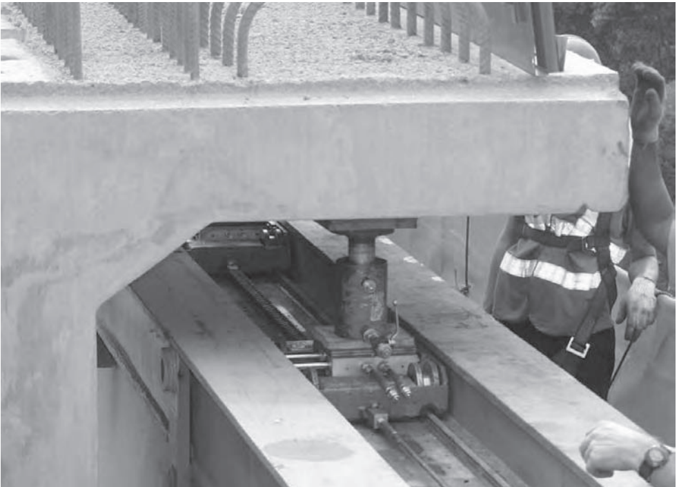
Figure 15.10 West Rail, Hong Kong: detail of sledges (Photo: VSL, www.vsl.com )
