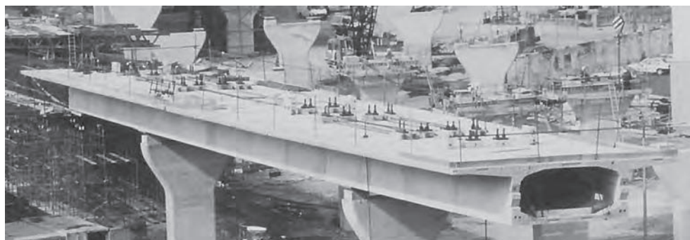
Figure 15.25 Belfast Cross Harbour Bridges: spans erected on temporary stressing alone (Photo: Graham-Farrans JV/Esler Crawford)
