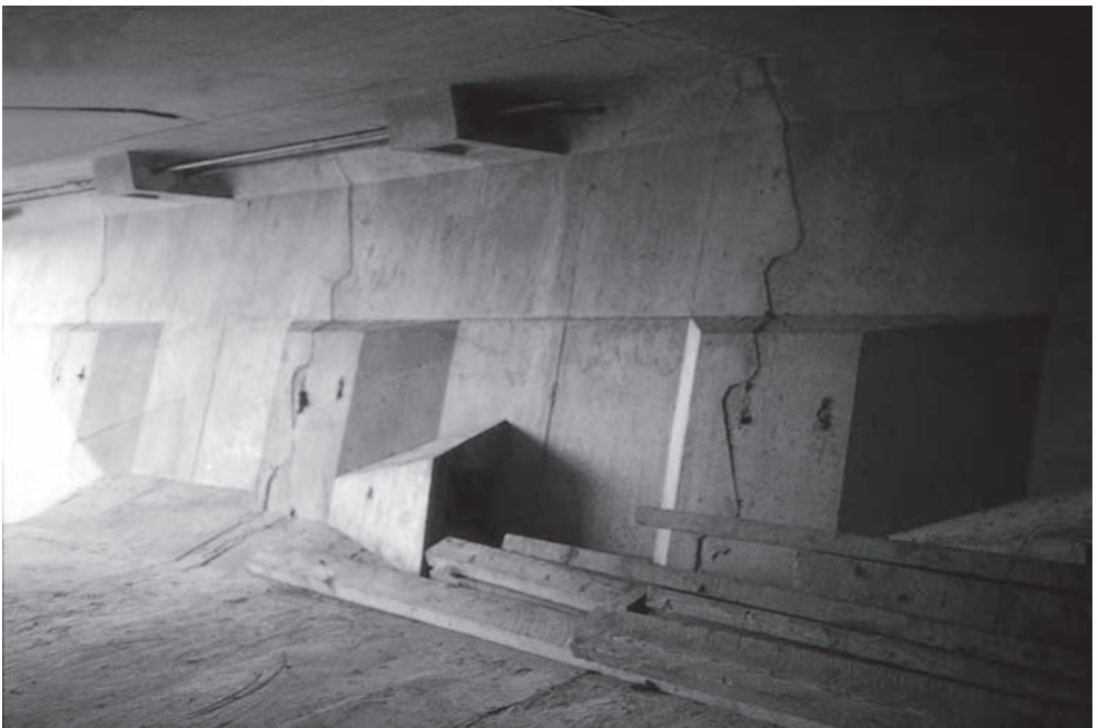
Figure 15.21 East Moors Viaduct: interior of box showing temporary stressing bars, web thickenings for face anchors and blisters for Stage 2 cables (Photo: Robert Benaim)
