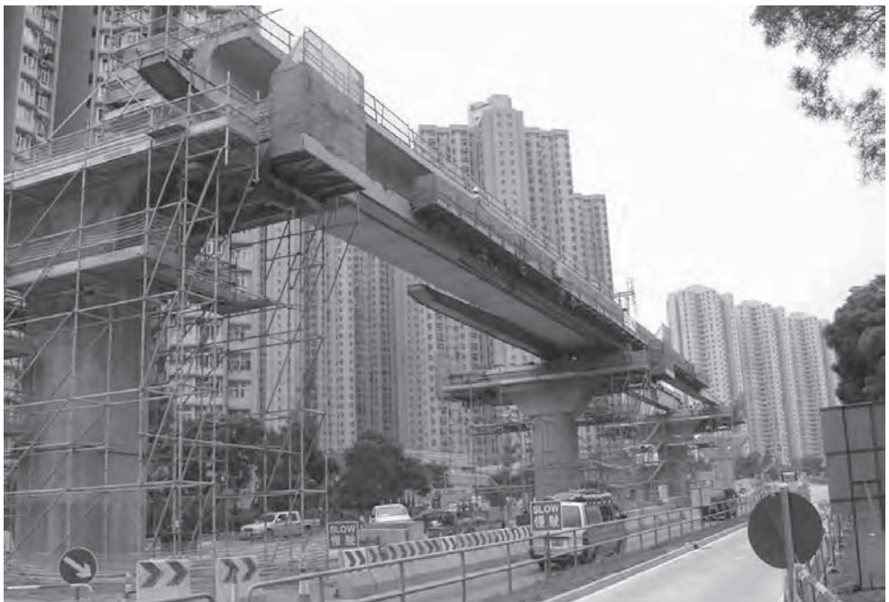
Figure 15.7 East Rail Gantry (Photo: VSL, www.vsl.com )
