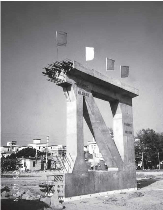
Figure 9.36 Trial panel of truss (Photo: Engineer Leo K.K. Leung, Executive Director of Hopewell Highway Infrastructure Ltd (Hong Kong Stock Code: 737))
