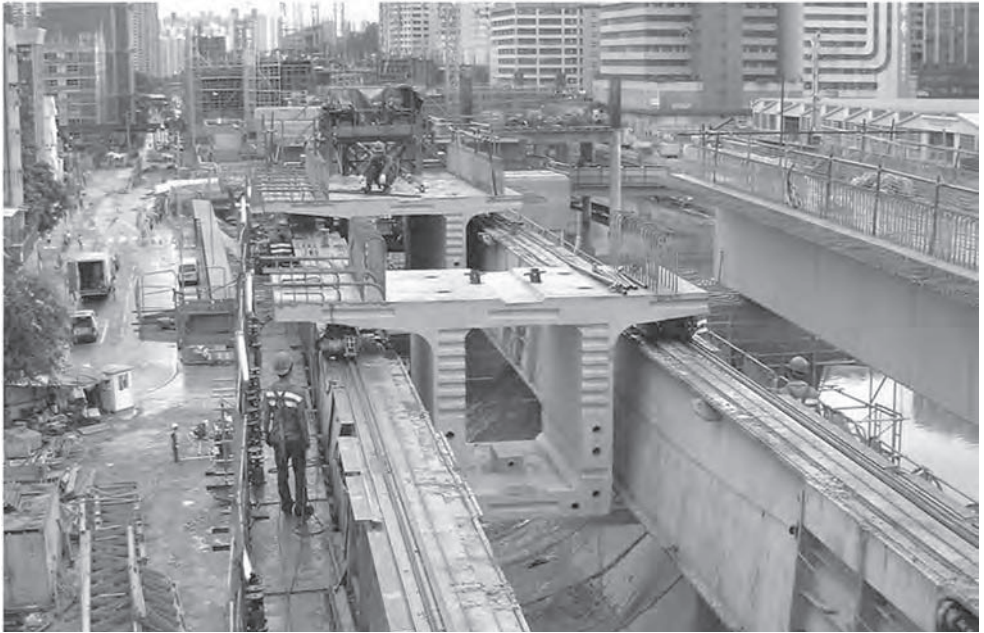
Figure 15.9 West Rail, Hong Kong: detail of gantry (Photo: VSL, www.vsl.com )
