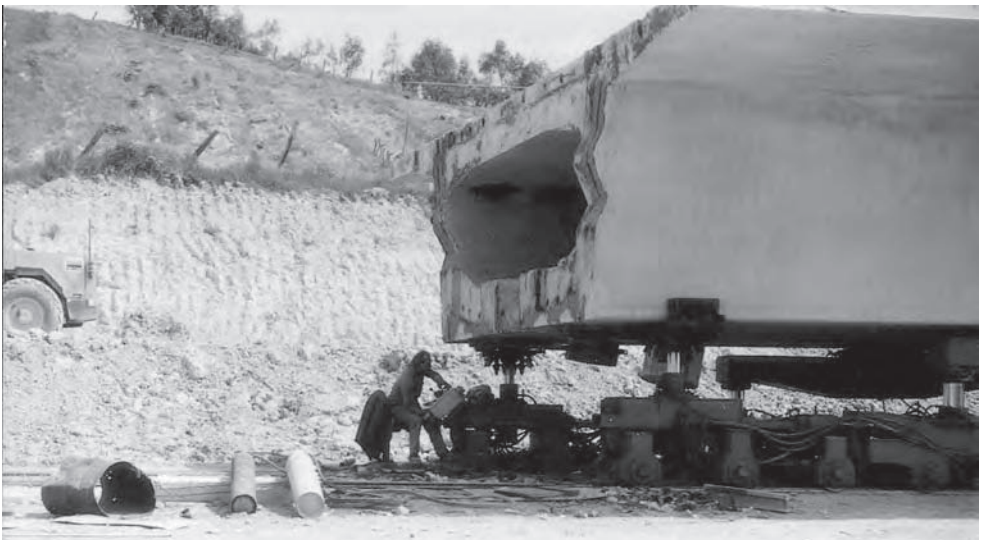
Figure 15.46 Poggio Iberna Viaduct, Italy: deck unit on its transporter (Photo: David Benaim)
