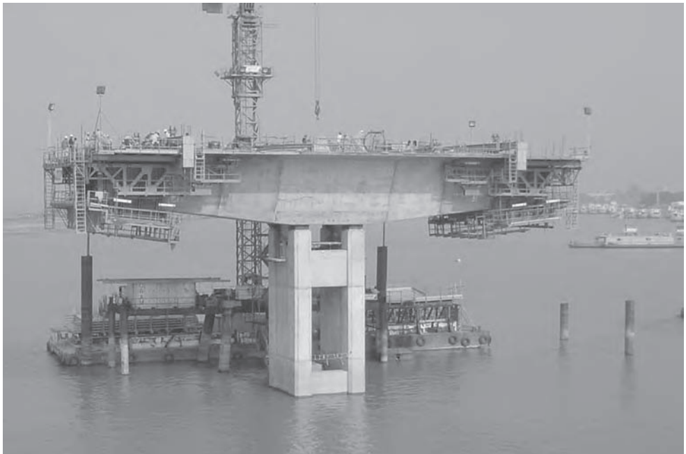
Figure 15.16 Bhairab Bridge, Bangladesh: underslung falsework travellers (Photo: Roads and Highways Department, Government of Bangladesh and Edmund Nuttall)
