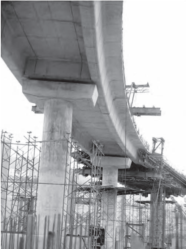
Figure 12.8 Contract 308 of the HKMTR, Tai Ho Viaduct: twin rib deck with pier diaphragms (Photo: Robert Benaim)
