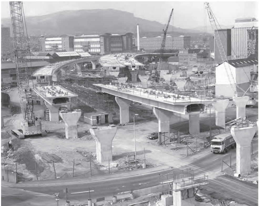
Figure 15.29 Belfast Cross Harbour Bridges: the flexibility of crane erection (Photo: Graham-Farrans JV/Esler Crawford)
