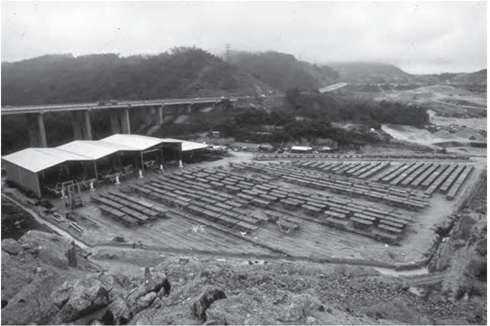
Figure 14.16 STAR: casting factory and storage (Photo: Benaim)
