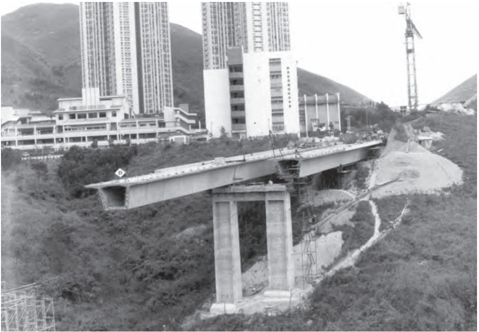
Figure 15.44 Liu To Bridge, Hong Kong (Photo: Dragages et Travaux Publics, Hong Kong)
