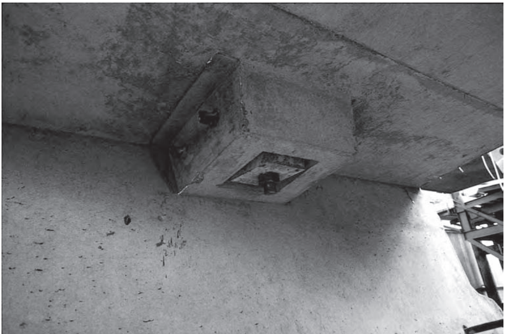
Figure 14.14 East Moors Viaduct: temporary stressing blister doubling as lifting point (Photo: Benaim)
