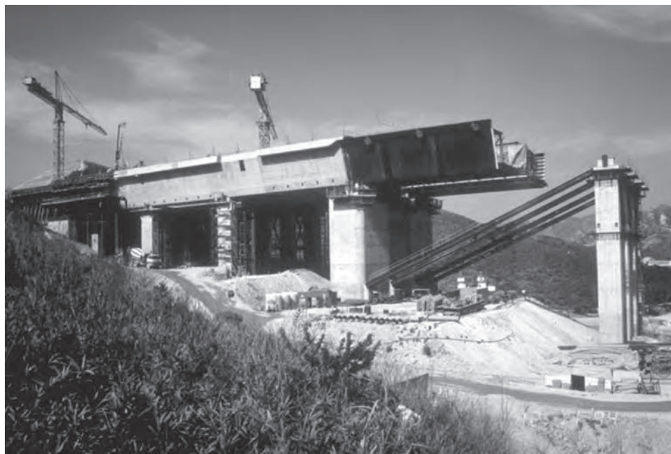
Figure 15.42 Kap Shui Mun Bridge, Hong Kong: launching of approach span (Photo: Benaim)
