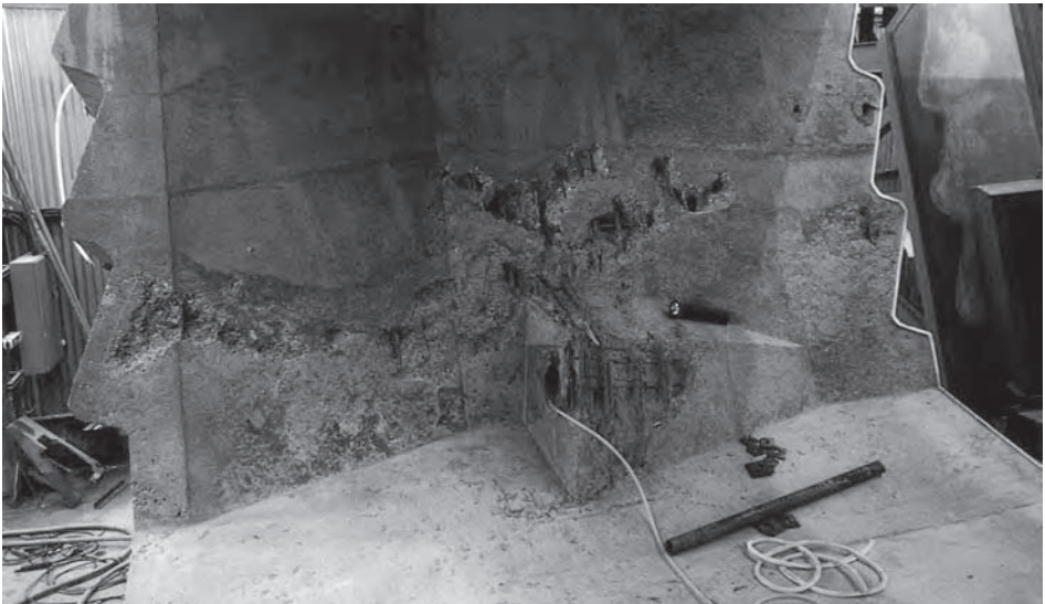
Figure 9.25b East Moors Viaduct: failed pour for trial segment (Photo: Benaim)
