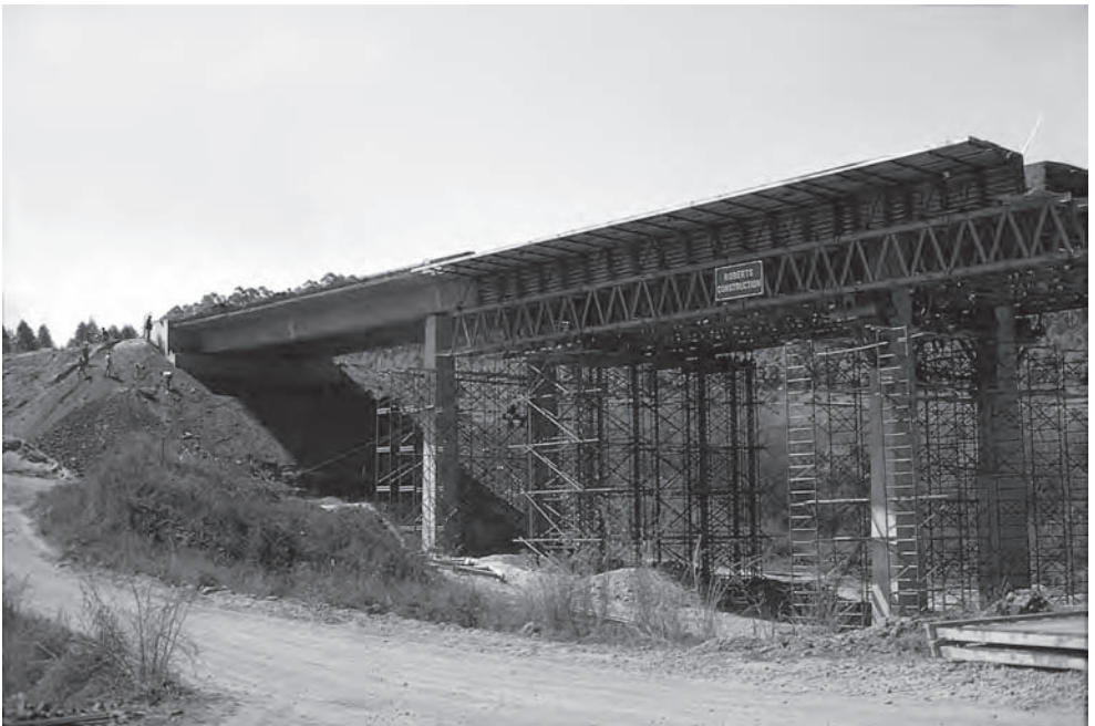
Figure 12.16 Doornhoek Bridge: typical falsework for span-by-span construction of short bridge (Photo: Arup)
