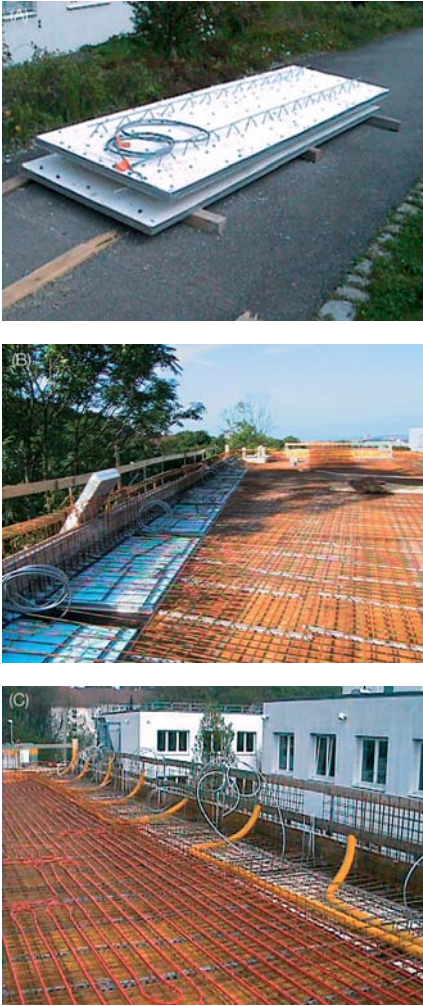
Figure 2.20 (A) The edge strip heating elements placed in the formwork. (B) Technical installation in the reinforced concrete floor prior to pouring. (C) Heating, cooling, and ventilation pipes are integrated into the reinforcement. (© Dietmar Strauß, Besigheim, Germany, and © Martin Duckek, Ulm, Germany)
