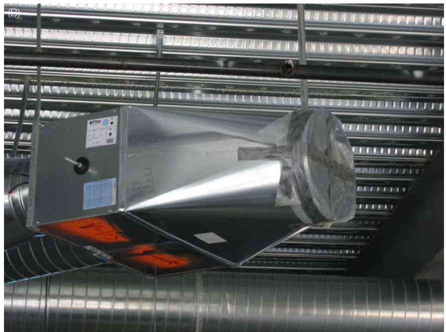
Figure 13.3 (A) Ductwork should be protected during storage and prior to installation. (B) Openings should be sealed during the installation process to prevent contamination. (Photographs courtesy of DPR Construction, Inc.)
