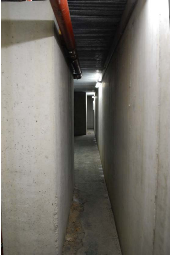
Figure 7.10 After entering the building through the outside air intake grilles, air flows through the earth canal, which cools the air via ground contact in summer and heats it in winter.
