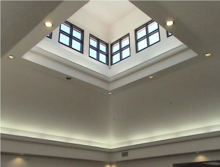
Figure 12.2 (A) A clerestory conducts diffuse light into a lobby below at St. Johns River State College in St. Augustine, Florida. (D. Stephany)
