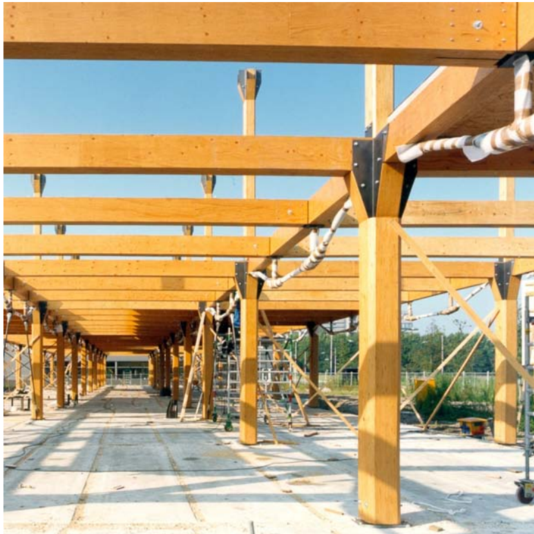
Figure 11.11 (B) The columns and beams, shown during construction. (J. M. Post, XX Architecten)
