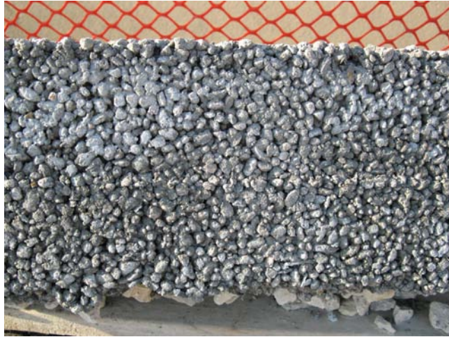
Figure 10.16 (L) Pervious pavement is made from concrete or asphalt, with coarse aggregates that create air voids, allowing water to pass through the system. (Source: City of Fairway, Kansas)
