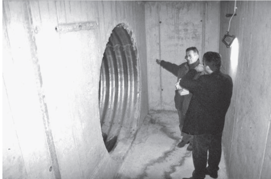
Figure 9.24 Ground-coupled system showing an air intake tube, 1.8 meters (6 feet) in diameter, under a Mercedes showroom in Stuttgart, Germany. The galvanized steel tube, which is 100 meters (325 feet) long, heats cold air via ground contact in winter and cools hot air in summer. The tube is located in a zone under the building where the temperature is a constant 60°F (16°C).
