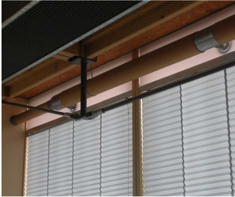
Figure 11.11 (E) Cardboard ductwork is inexpensive, resourceful, and recyclable and will be close to the end of its life expectancy by the time the XX Office Building is ready for deconstruction. (D. Stephany)
