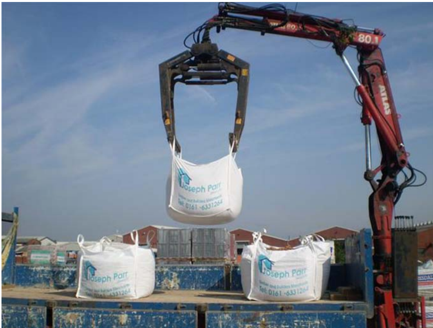
Figure 13.5 A crane moving bulk materials in large, reusable heavy-duty bulk bags from a truck for use in construction. (Photograph courtesy of Custom Packaging Products)
