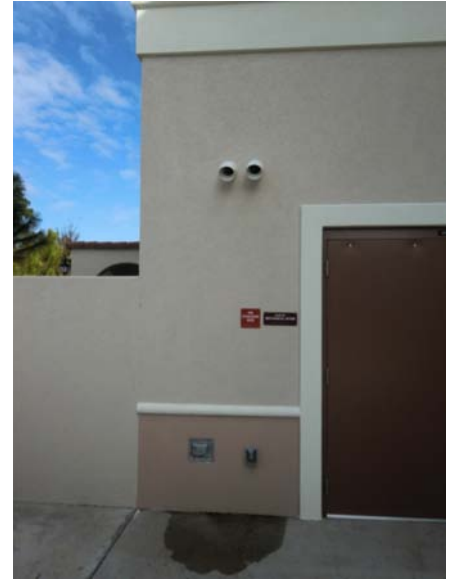
Figure 13.10 The CxA identified boiler exhaust condensation and dripping onto an exterior outlet and proposed the relocation of the electrical outlet to prevent future corrosion as well as increase safety. (Photograph courtesy of John Chyz, Cross Creek Initiative, Inc.)
