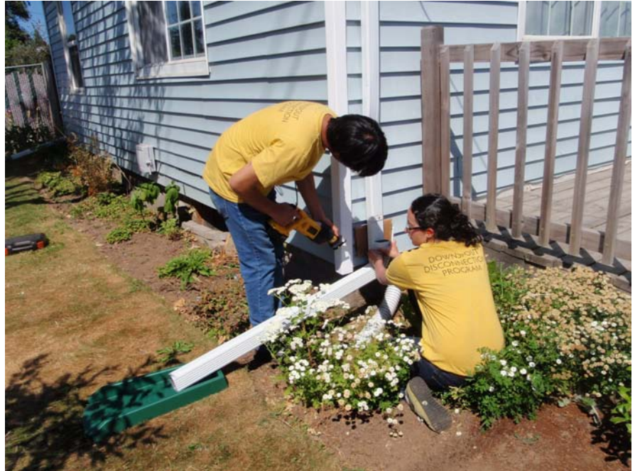
Figure 10.16 (A) Disconnecting downspouts from storm sewer systems prevents roof runoff from overloading these systems by dispersing it to vegetated areas. (Source: City of Gresham, Oregon)
