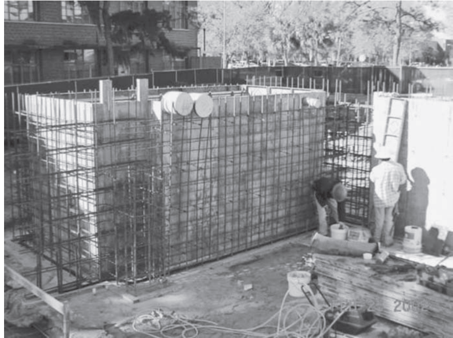
Figure 10.9 The rainwater harvesting system for Rinker Hall at the University of Florida in Gainesville has a cast-in-place cistern (shown here under construction) located under the south stairwell of the building. The rainwater is used for flushing the building's toilets. (Photograph courtesy of Centex-Rooney, Inc.)
