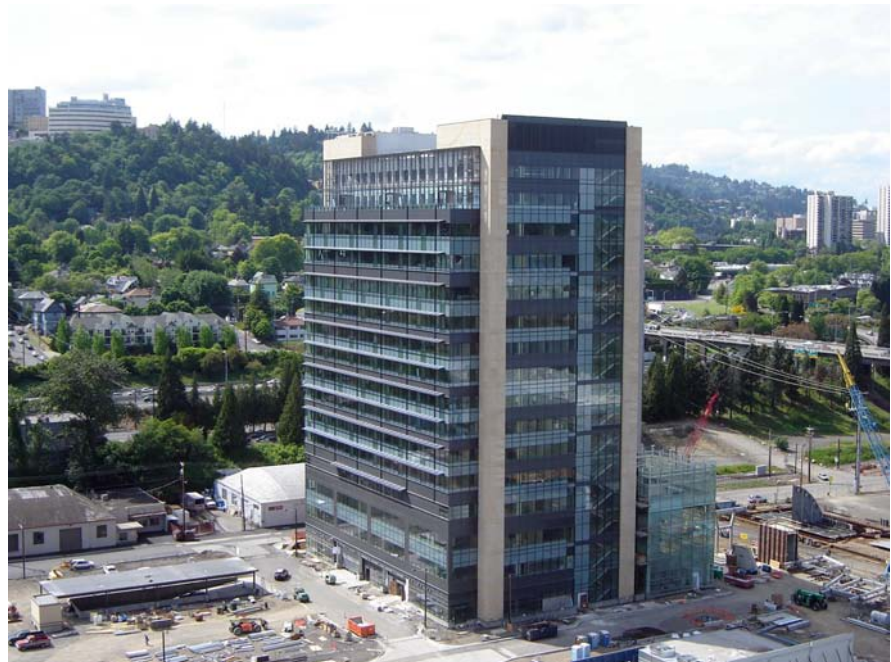
Figure 9.32 The Oregon Health and Science University's River Campus Building One, shown in the late stages of construction, is a LEED-NC 2.1 platinum certified building. (Courtesy of Interface Engineering)
