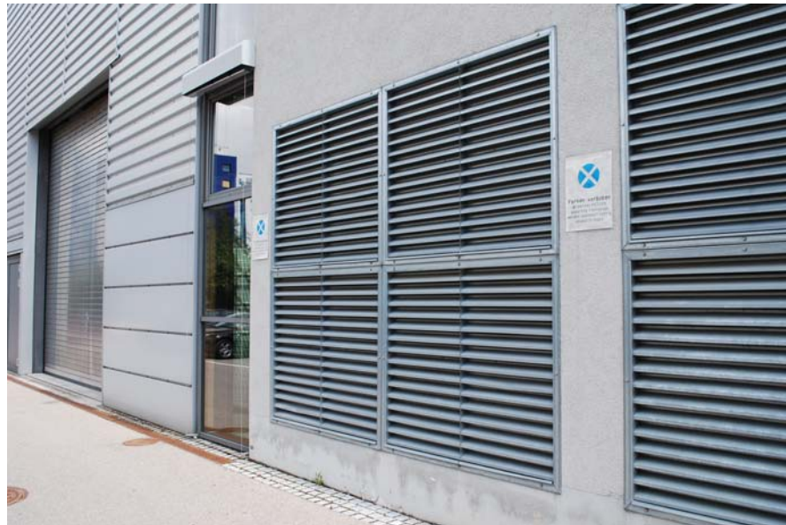
Figure 7.9 The grilles for the outside air intake for Theaterhaus are located on the side of the building. Air is induced to flow through the building by the rising warm air in the exhaust air chimney located on the top of the building.
