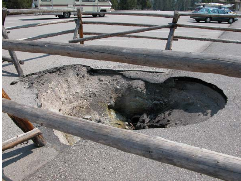
Figure 10.6 Sinkholes are an example of land subsidence due to groundwater extraction. Since groundwater serves partly as a structural component to the rock, its depletion results in voids and eventual collapse, sometimes sudden and unpredictable, creating a substantial hazard to people and infrastructure. (Photograph courtesy of Ildar Sagdejev)
