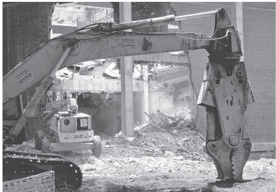
Figure 11.1 Partial demolition of the Levin College of Law library at the University of Florida in Gainesville for a building expansion project. Truly green buildings of the future should be designed for deconstruction to maximize the reuse and recovery of building components and materials. (Photograph courtesy of M. R. Moretti)
