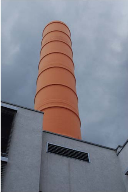
Figure 7.8 The key element of the Theaterhaus natural ventilation system is a 93-foot (30-meter) chimney, which induces airflow from outside the building, through the building interior space, to be exhausted by the stack, or chimney, effect. The chimney was a feature that was added to the building and which adds to the industrial appeal and appearance of the former steelworks building.
