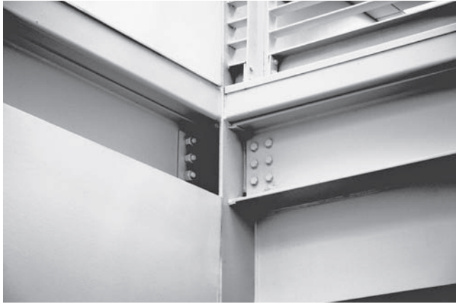
Figure 11.10 One of the innovations in the design of Rinker Hall at the University of Florida in Gainesville was to include DfD as a design criterion. One of the design features is the use of bolted, exposed steel connections to permit their ready removal. (Photograph courtesy of M. R. Moretti)
