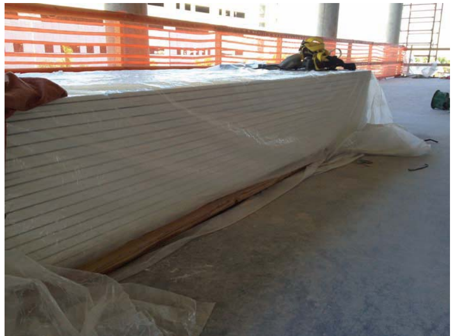
Figure 13.6 Construction products and materials such as the gypsum board shown here should be kept dry, covered, and off the ground to prevent future mold and IAQ problems. (Photograph courtesy of DPR Construction, Inc.)
