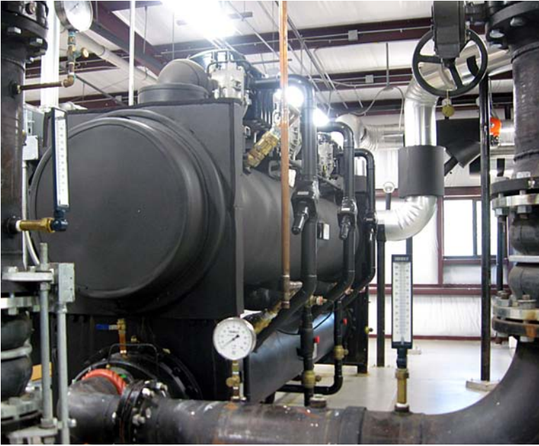
Figure 6.5 A high-efficiency Smardt centrifugal chiller was installed to replace the outdated unit, providing cooling for the entire St. Johns River State College. The chiller is designed to meet future needs as the campus continues to expand. (Photograph courtesy of Glen Roberts, St. Johns River State College)
