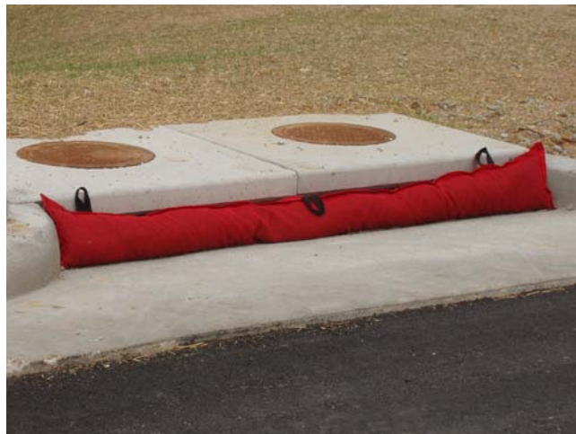
Figure 13.1 Storm drain inlet protection implementation on a newly constructed site. This type of device must be continuously monitored during construction operations to ensure it is functioning properly. (Don Thieman, CPESC, ASP Enterprises)
