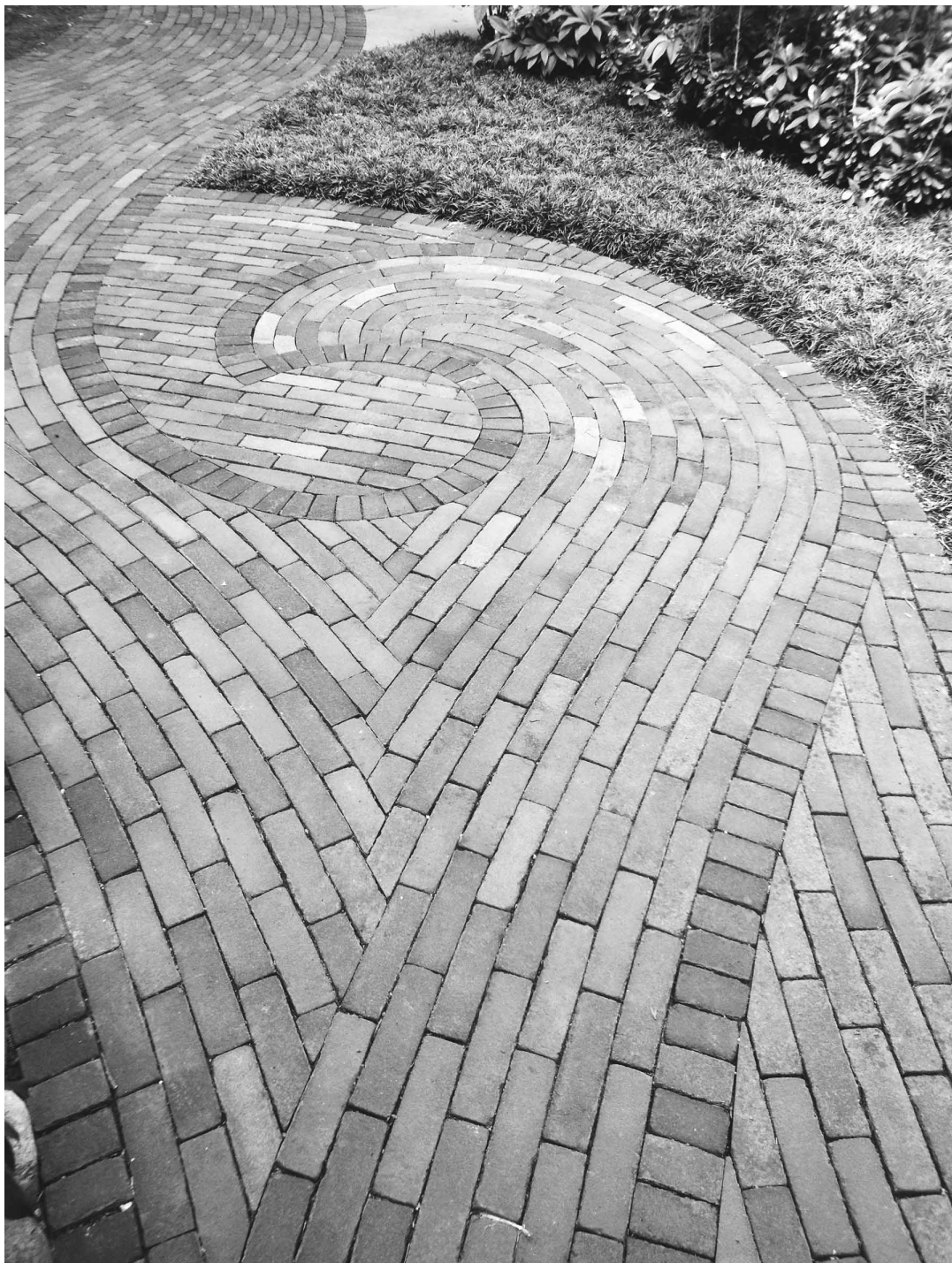
FIGURE 20. ONDINE GARDEN, DUMBARTON OAKS, WASHINGTON, D.C. (2008). JOHN POND AND NATHANIEL TRENT, MASONS. (Courtesy Magenta Livengood.) Hard-fired brick pavers were dry-laid in an intricate pattern following the elegant design of Beatrix Ferrand in this historic garden. About 10 percent of the bricks were cut by hand during installation.
