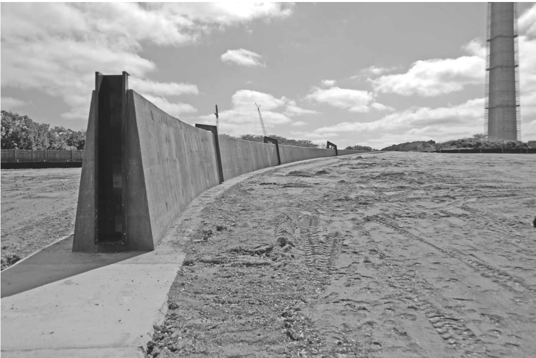
FIGURE 63. POTOMAC PARK LEVEE, WASHINGTON, D.C. (2012—UNDER CONSTRUCTION). OLIN, PHILADELPHIA AND LOS ANGELES. (Courtesy Magenta Livengood.) This levee complies with new post-Katrina FEMA 100-year flood-control requirements. Along with the earth berms and stone-clad concrete walls, 17th Street can be blocked with a post-and-panel system that can be installed with 24 hours’ notice. These measures will prevent rising waters from the Potomac River from flooding the Federal Triangle and other critical areas in the district.
