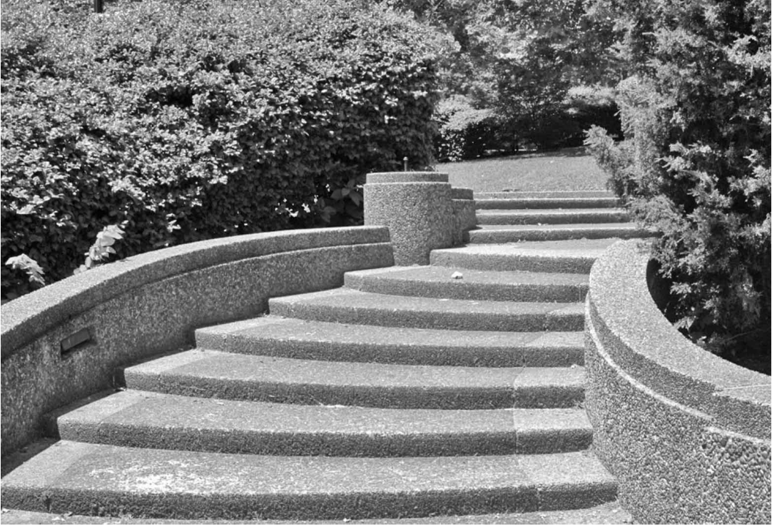
FIGURE 1. MERIDIAN HILL PARK, WASHINGTON, D.C. (1915–1936). JOHN J. EARLEY, ROSSLYN, VIRGINIA. (Courtesy Magenta Livengood.) The innovative and patented cast-in-place and pre-cast concrete techniques used mixes with stone pebble aggregate that were sorted by color and size. The result was intended to have a similar appearance as cut stone panels, railings and ornament, but it cost less. The stairs flow down the hill in a way that is well suited to the material of concrete. In 1994, this park was the first in the country to be recognized as a National Historic Landmark.
