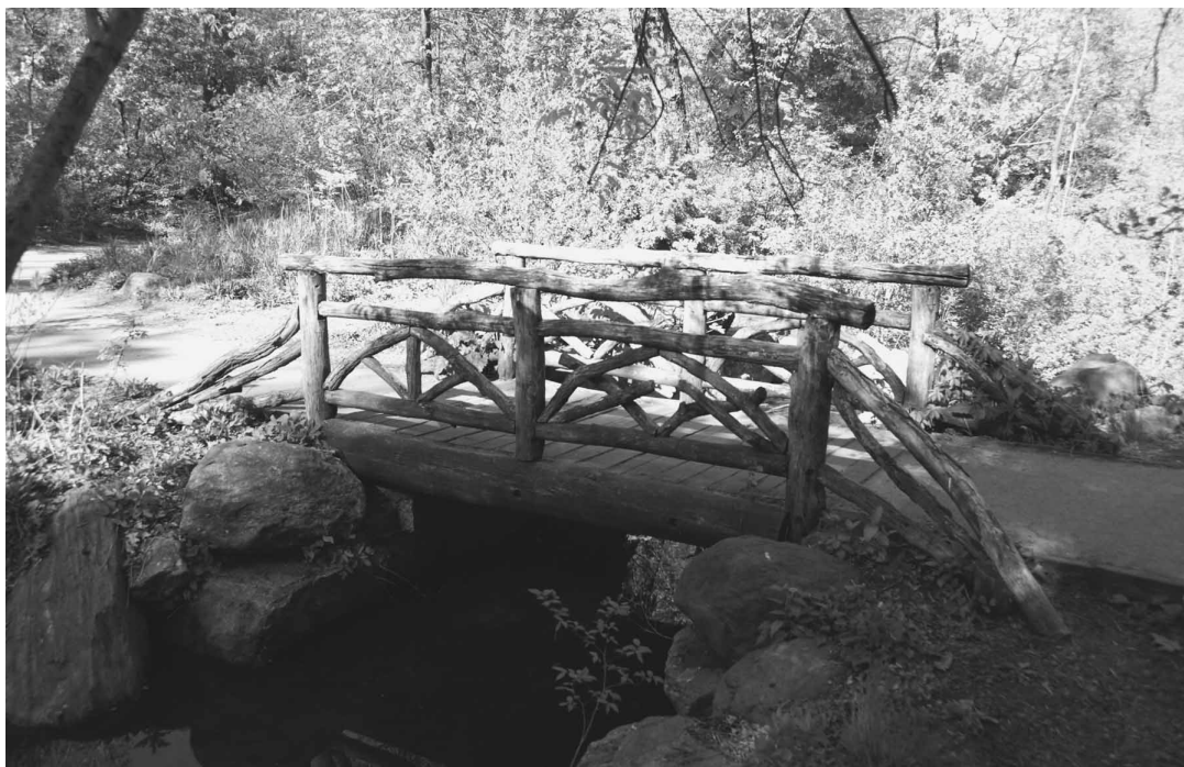
FIGURE 56. RUSTIC BRIDGE, CENTRAL PARK, NEW YORK CITY (OPENED IN 1859, REBUILT AS NEEDED). (Courtesy Magenta Livengood.) Rough wood logs from fallen trees salvaged in the park are used for repairing or replacing rustic structures. They are found in the wilder areas and support a feeling of being in the country.
