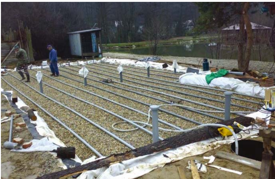
Figure 4-46. Distribution of wastewater across the surface of VF bed at Bojna, Slovakia. Photo by Milan Raffesberg, with permission.
