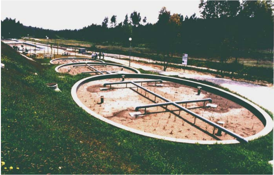
Figure 4-45. Wastewater distribution at vertical flow constructed wetland which is a part of the treatment system for landfill leachate near Leiria, Portugal. Photo by Jan Vymazal.
