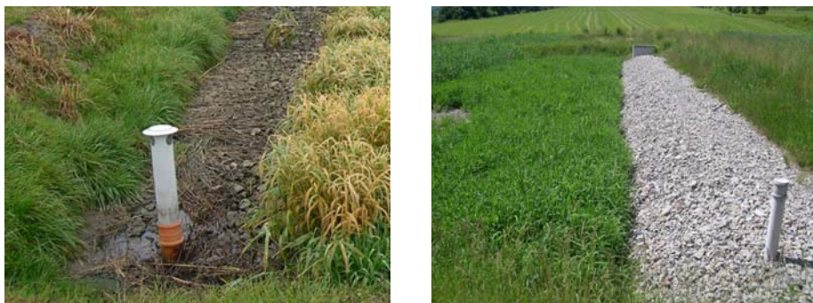
Figure 5-29. Inspection pipes at the end of inflow zone. Left: CW Čejkovice, right: Mořina, Czech Republic. Photos by Jan Vymazal.
