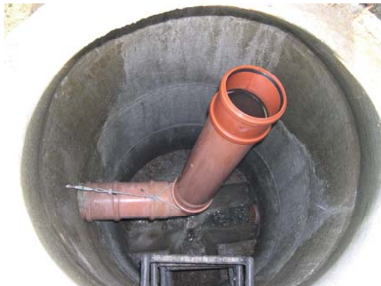
Figure 5-33. Socketted pipe at the outflow from a HF CW in Krásna Lúka, Slovakia, Photo by Jan Vymazal.
