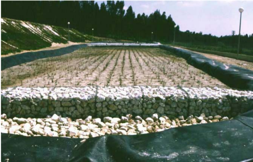
Figure 6-9. HF constructed wetland as a part of a VF-HF hybrid constructed wetlands for landfill leachate in Leiria, Portugal. Photo by Jan Vymazal.
