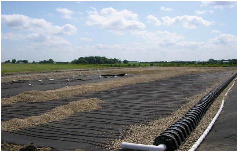
Figure 7-36. Installation of influent distribution chamber and aeration lines for HF CW at Prinsburg, Minnesota, U.S.A. Photo by Scott Wallace, with permission.
