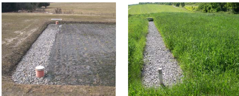
Figure 5-32. Outflow zones are leveled with the filtration bed surface. The zones are frequently equipped with inspection pipes. Left: CW Sklené, Czech Republic, right: CW Mořina, Czech Republic. Photos by Jan Vymazal.
