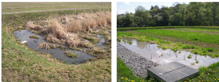
Figure 5-21. Surfacing (ponding) of wastewater in the inlet zone of HF constructed wetlands Břehov (left) and Mořina (right), Czech Republic. Photo by Lenka Kröpfelová.
