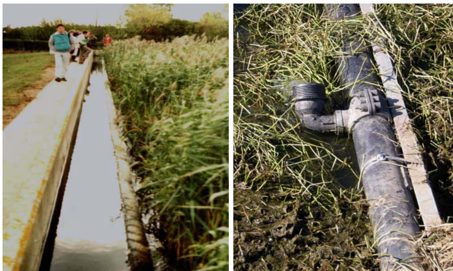
Figure 5-24. Open inflow trench in HF CW Acle, United Kingdom (left) and adjustable tees in HF CW Otorohanga, New Zealand (right). Photos by Jan Vymazal.
