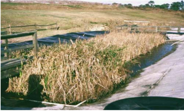
Figure 7-39. Pilot-scale (71.7 m 2 ) HF constructed wetland for landfill leachate at the New Hanover County landfill, North Carolina, U.S.A. Photo by Jan Vymazal.
