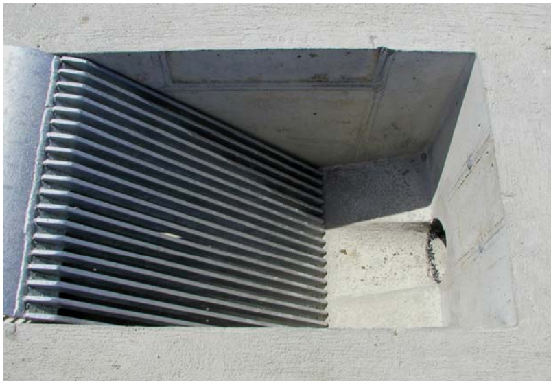
Figure 5-7. Bar screens. Constructed wetland Čejkovice, Czech Republic. Photo by Lenka Kröpfelová.
