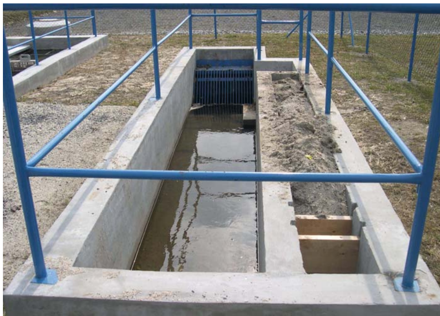
Figure 5-13. Horizontal flow grit chamber with side grit compartment. CW Sklené, Czech Republic. Photo by Lenka Kröpfelová.
