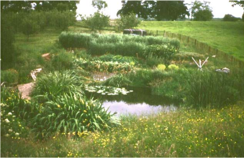
Figure 4-42. Hybrid system at Oaklands Park, UK. The first VF stage ( 6 \times 8 \text{ m}^2 ) is composed of six beds planted with Phragmites australis (top back of the picture), the second VF stage (below, 3 \times 5 \text{ m}^2 ) is composed of three beds planted with Scirpus lacustris , Iris pseudacorus and P. australis . The third HF stage ( 8 \text{ m}^2 ) is planted with I. pseudacorus and the 4 th HF stage ( 20 \text{ m}^2 ) is planted with Acorus calamus , S. lacustris , Carex elata and Sparganium erectum . Photo by Jan Vymazal.
