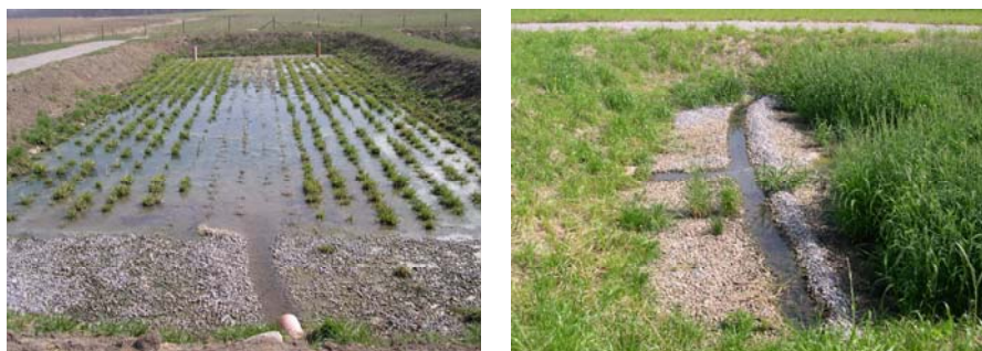
Figure 5-31. Distribution of wastewater in HF CW Břehov, Czech Republic. Left: Wastewater flows through the middle of the bed causing shortcircuiting, right: raised wall which spreads the wastewater along the whole inlet zone. Photos by Lenka Kröpfelová.
