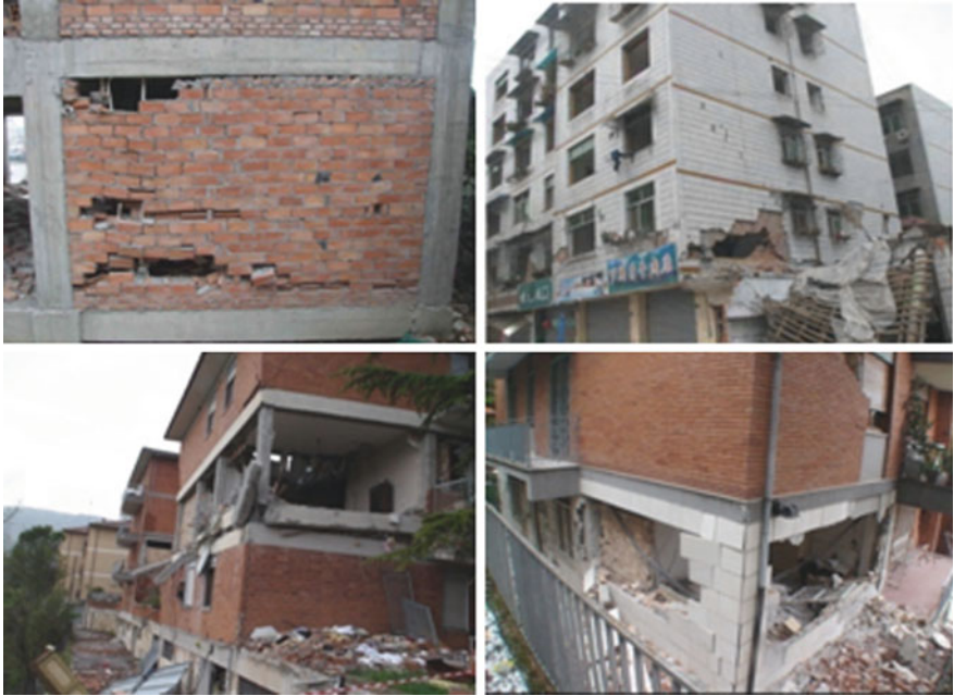
Fig. 33.1 URM infill walls damage from earthquakes in 2008 Wenchuan, China ( top ) and 2009 L'Aquila, Italy ( bottom )
