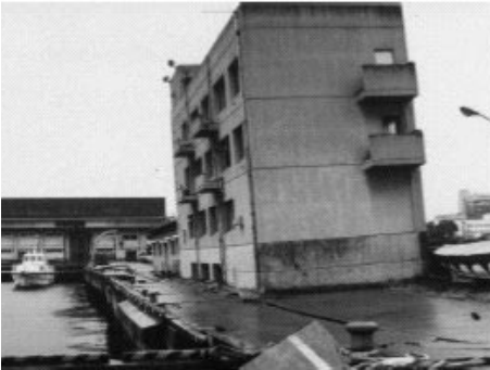
Photo 11.1. Tilted building in lateral spreading area
