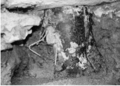
Photo 11.3. Damage to pile head
