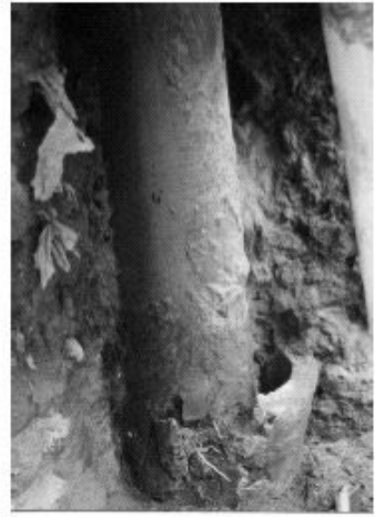
Photo 11.4. Damage to pile near ground water table
