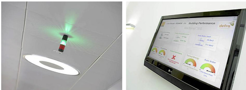
FIGURE 4.2 Traffic light system for natural ventilation (Left) and the energy performance dashboard (right). Courtesy http://www.kier.co.uk/uploaded/fileupload/Defra%20Inwick%20Case%20Study .
