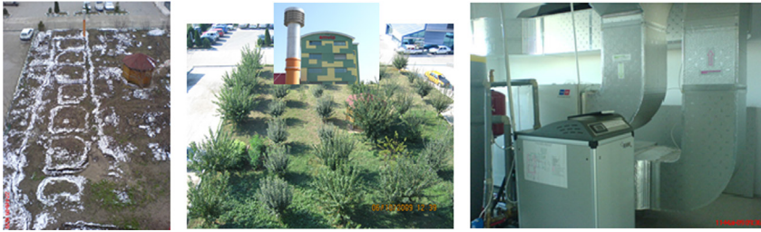
FIGURE 15.10 Earth heat exchanger, fresh air introduction pipe, controlled ventilation system with energy recovery + heat pump.
