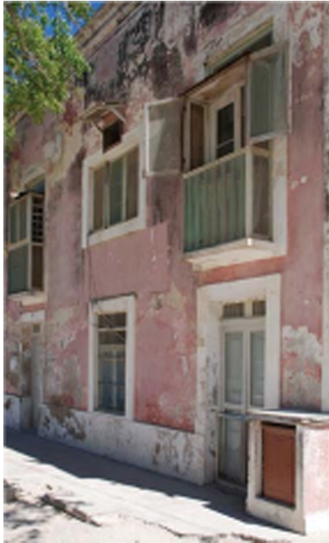
FIGURE 16.83 Use of mosquito net in an old building in Maputo, Mozambique.
