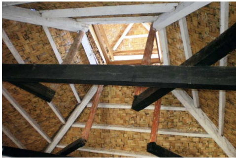
FIGURE 16.91 Interior of a stack ventilation tower in a house in Sao Vicente.
