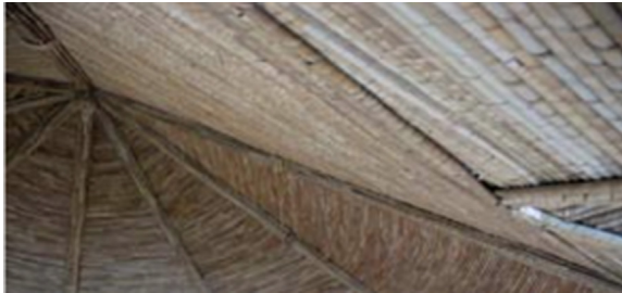
FIGURE 16.60 Internal roof insulation in a recent building, using local materials (thatch), in Guiné-Bissau (left), and Mozambique (right).
