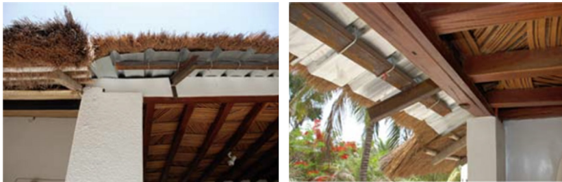
FIGURE 16.58 Roof with mixed construction system. The thatch is superimposed on the corrugated metal sheet (sub-layer): the benefits of sealing and durability conferred by the use of the metallic layer and the insulating ability of the thatch (tourism building, Guinea-Bissau).
