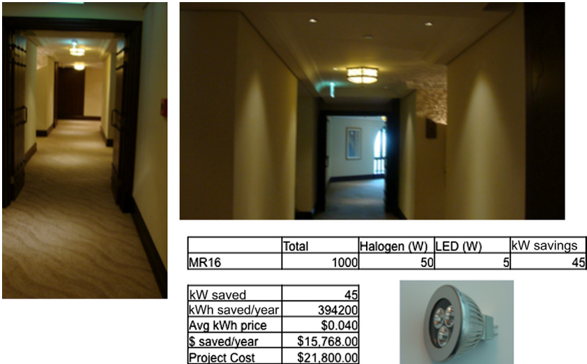
FIGURE 7.8 Pictures of the LED MR16 installed at the Shangri-la Hotel in Abu Dhabi; a summary table and a picture of the specific product used.
