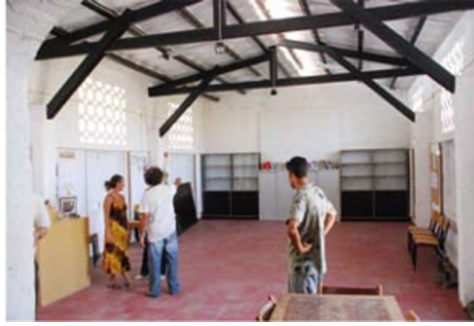
FIGURE 16.89 Building for cultural activities in Lagedos. Openings at top and opposing fronts, for cross ventilation, and opening on the roof for stack effect ventilation.
