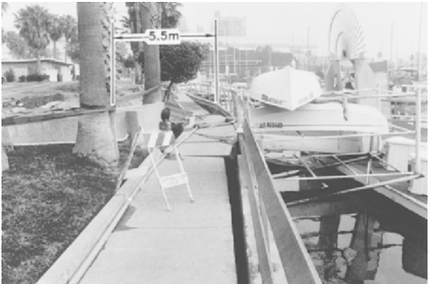
FIGURE 9.22 Damage to a marine facility caused by the California Northridge earthquake on January 17, 1994. (From Kerwin and Stone 1997; reprinted with permission from the American Society of Civil Engineers.)
