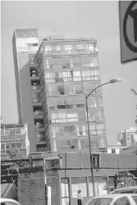
FIGURE 4.25 Building damage and tilting in Mexico City caused by the Michoacan earthquake in Mexico on September 19, 1985. (Photograph from the Steinbrugge Collection, EERC, University of California, Berkeley.)
