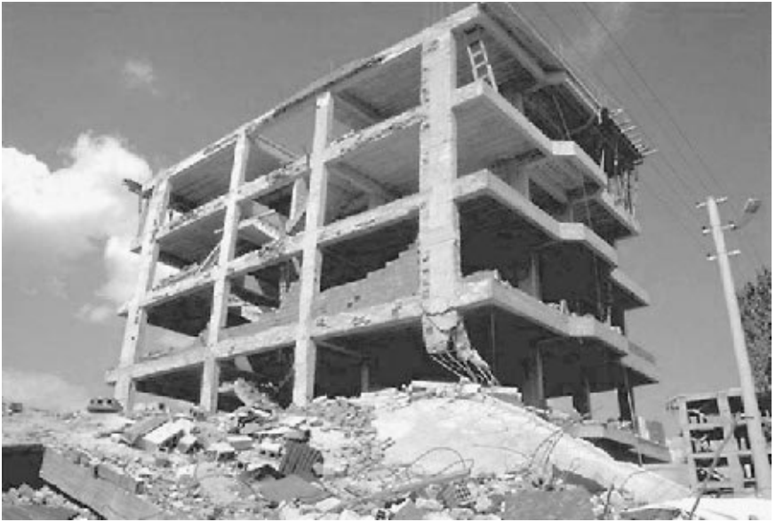
FIGURE 4.22 The building shown has lost a corner column due to the collapse of an adjacent building during the Izmit earthquake in Turkey on August 17, 1999. Note that the roof of the collapsed building now rests on the third-story corner of the standing building. (Photograph from the Izmit Collection, EERC, University of California, Berkeley.)
