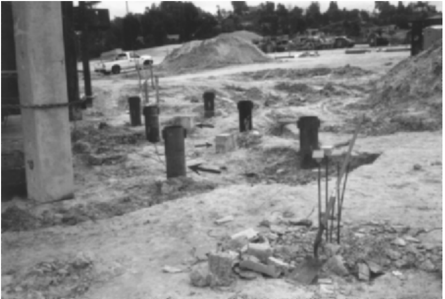
FIGURE 13.24 Pile load test. The small arrows point to the prestressed concrete piles, which will be subjected to a load test. The large arrow points to one of the six anchor piles.
