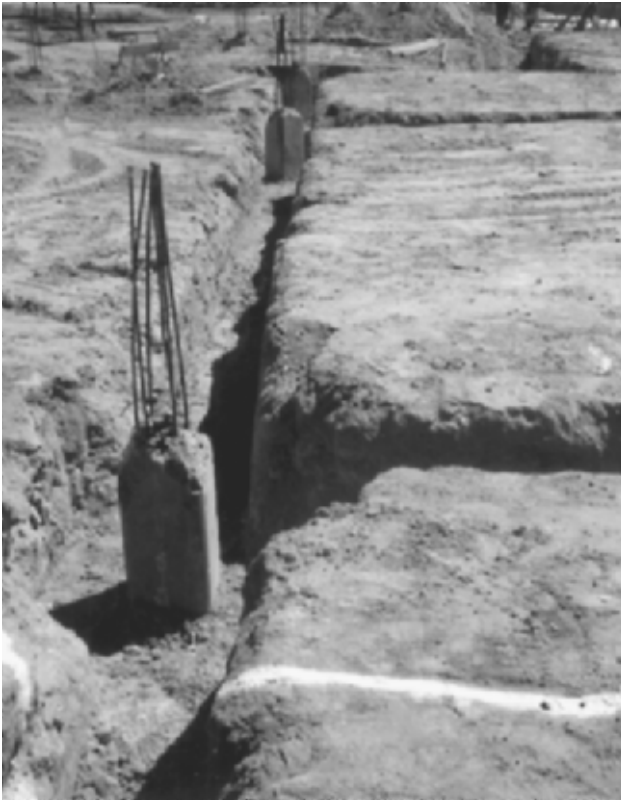
FIGURE 13.29 Prestressed concrete piles have been installed, and the excavations for the pile caps and grade beams are complete. The strands at the top of the pile will be connected to the steel reinforcement in the pile cap and grade beam.
