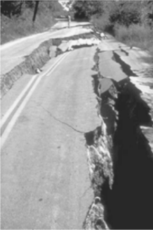
FIGURE 9.35 Earthquake damage to a two-lane road in Santa Cruz Mountains. The slope movement was caused by the Loma Prieta earthquake in California on October 17, 1989. (Photograph from the Loma Prieta Collection, EERC, University of California, Berkeley.)
