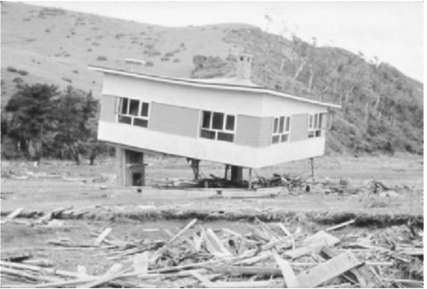
FIGURE 3.58 Tsunami damage caused by the Chile earthquake in 1960. (Photograph from the Steinbrugge Collection, EERC, University of California, Berkeley.)
