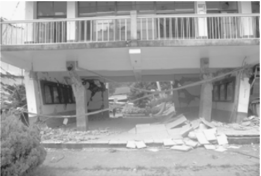
FIGURE 3.6 Portion of a building that remained standing at the Kuang Fu Elementary School. This portion of the building was directly adjacent to the surface fault rupture associated with the Chi-chi (Taiwan) Earthquake on September 21, 1999. Note in this figure that the ground was actually compressed together adjacent to the footwall side of the fault rupture. (Photograph from the Taiwan Collection, EERC, University of California, Berkeley.)
