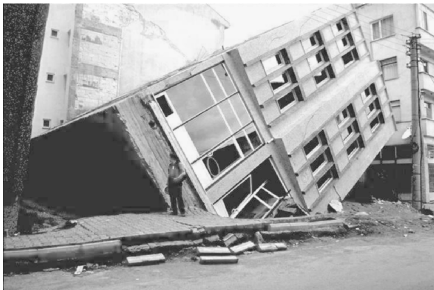
FIGURE 8.4 The building suffered a liquefaction-induced bearing capacity failure during the Izmit earthquake in Turkey on August 17, 1999. (Photograph from the Izmit Collection, EERC, University of California, Berkeley.)
