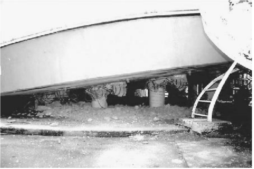
FIGURE 4.12 Overview of a collapsed gas storage tank, located at a gas storage facility near Sabanci Industrial Park, Turkey. The elevated gas storage tank collapsed during the Izmit earthquake in Turkey on August 17, 1999. (Photograph from the Izmit Collection, EERC, University of California, Berkeley.)
