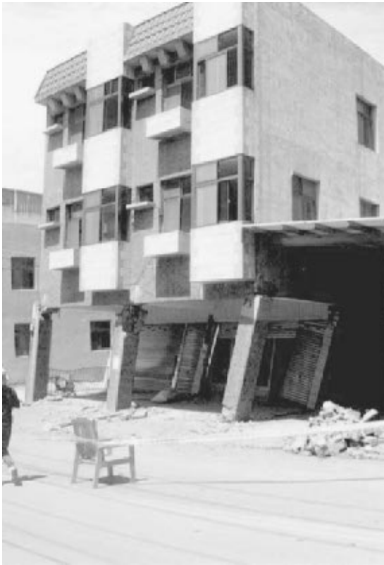
FIGURE 4.5 Damage due to a soft story at the ground floor. The damage occurred during the Chi-chi earthquake in Taiwan on September 21, 1999. (Photograph from the USGS Earthquake Hazards Program, NEIC, Denver.)
