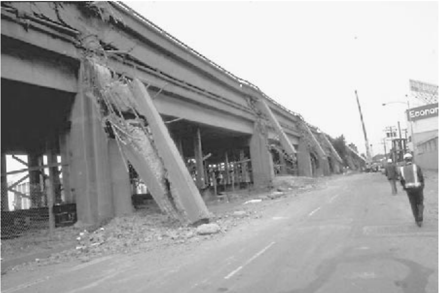
FIGURE 4.28 Close-up view of the collapse of the Cypress Street Viaduct caused by the Loma Prieta earthquake in California on October 17, 1989. (From USGS.)
