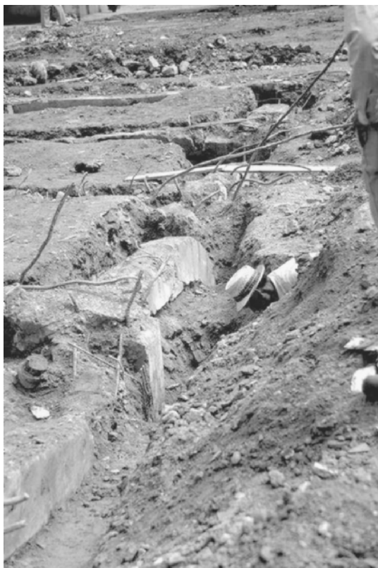
FIGURE 8.6 The building foundation shown above was constructed of individual footings that were interconnected with concrete tie beams. The building collapsed during the Caracas earthquake in Venezuela on July 29, 1967. When the foundation was exposed, it was discovered that the spread footings had punched downward into the soil. Note that the tie beam at the center of the photograph was bent and pulled downward when the footing punched into the underlying soil. (Photograph from the Steinbrugge Collection, EERC, University of California, Berkeley.)
