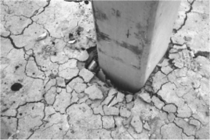
FIGURE 13.23 This prestressed concrete pile struck an underground obstruction, displaced laterally, and broke near ground surface. The arrow points to the location of the breakage.
