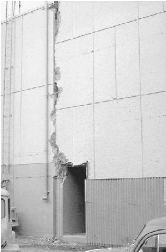
FIGURE 4.20 Pounding damage to the Anchorage-Westward Hotel caused by the Prince William Sound earthquake in Alaska on March 27, 1964. The building on the right half of the photograph is the 14-story hotel, while the building visible on the left half of the photograph is the ballroom. (Photograph from the Steinbrugge Collection, EERC, University of California, Berkeley.)
