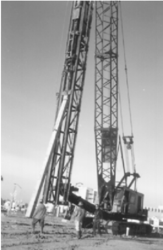
FIGURE 13.20 Pile-driving equipment. A prestressed concrete pile is in the process of being hoisted into position.
