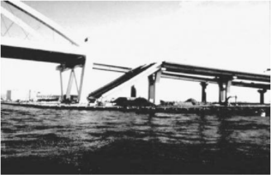
FIGURE 3.37 Collapse of a span of the Nishihomiya Bridge, apparently due to lateral retaining wall movement during the Kobe earthquake on January 17, 1995. (Photograph from the Kobe Geotechnical Collection, EERC, University of California, Berkeley.)
