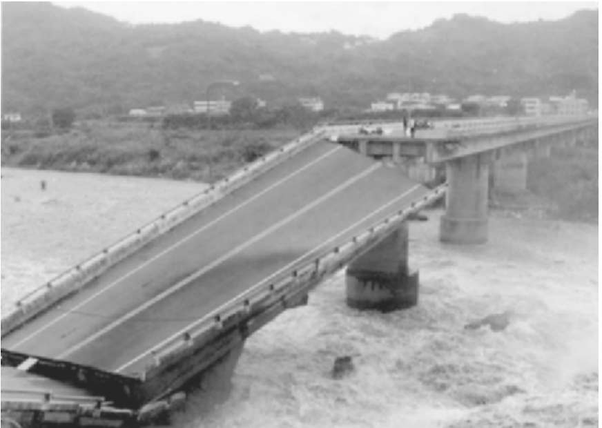
FIGURE 3.9 Collapsed bridge north of Fengyuen caused by surface fault rupture associated with the Chi-chi (Taiwan) earthquake on September 21, 1999. (Photograph from the USGS Earthquake Hazards Program, NEIC, Denver.)
