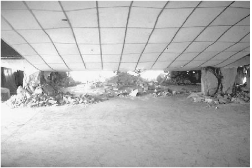
FIGURE 4.3 Torsional failure of the second story of the Hotel Terminal. The torsional failure occurred during the Gualan earthquake in Guatemala on February 4, 1976. (Photograph from the Godden Collection, EERC, University of California, Berkeley.)
