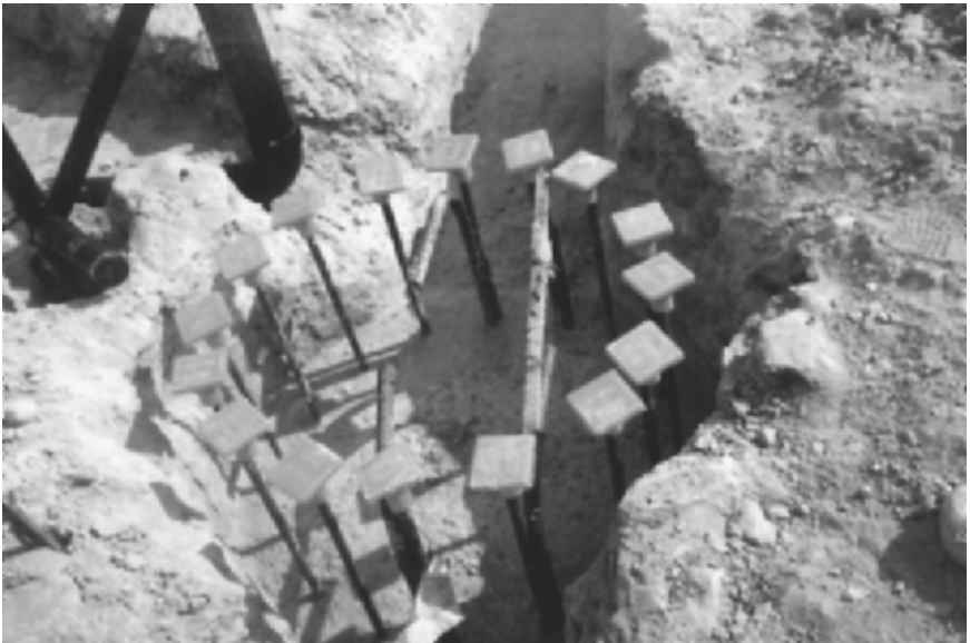
FIGURE 13.10 The pier hole has been filled with concrete. The steel reinforcement from the pier will be attached to the steel reinforcement in the grade beam.
