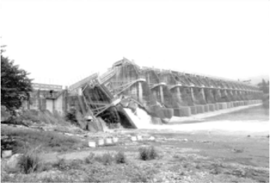
FIGURE 3.3 Overview of a dam damaged by surface fault rupture associated with the Chi-chi (Taiwan) earthquake on September 21, 1999. (Photograph from the Taiwan Collection, EERC, University of California, Berkeley.)
