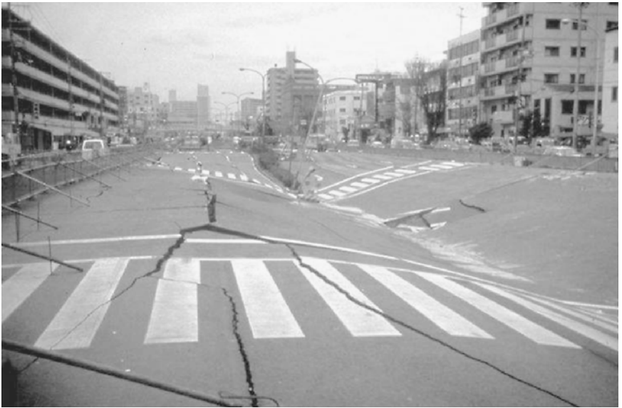
FIGURE 11.7 This picture shows street damage caused by the underlying collapse of the Daikai subway station. The January 17, 1995, Kobe earthquake (moment magnitude = 6.9) in Japan caused this damage. (Photograph from the Kobe Geotechnical Collection, EERC, University of California, Berkeley.)
