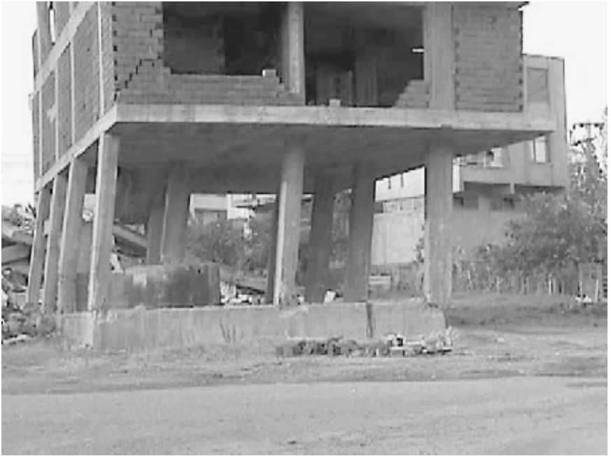
FIGURE 4.9 Damage caused by a soft story at the first-floor level. The damage occurred during the Izmit earthquake in Turkey on August 17, 1999. (Photograph by Mehmet Celebi, USGS.)
