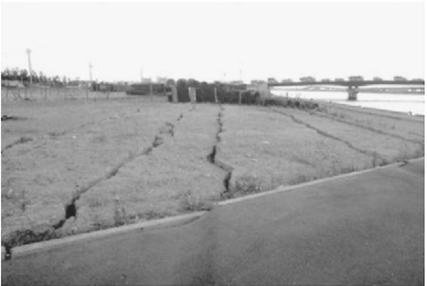
FIGURE 3.27 Ground cracks caused by lateral retaining wall movement due to liquefaction during the Kobe earthquake on January 17, 1995. The site is near Nishinomiya Port and consists of reclaimed land. (Photograph from the Great Hanshin Bridge Collection, EERC, University of California, Berkeley.)
