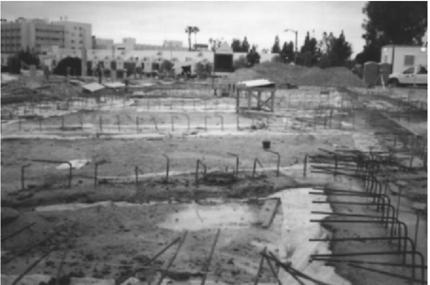
FIGURE 13.14 The concrete for the grade beams has been placed. The steel reinforcement from the grade beams will be attached to the steel reinforcement in the floor slab.
