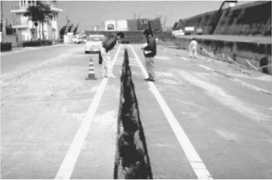
FIGURE 3.33 Damage on Port Island caused by retaining wall movement during the Kobe earthquake on January 17, 1995. (Photograph from the Kobe Geotechnical Collection, EERC, University of California, Berkeley.)
