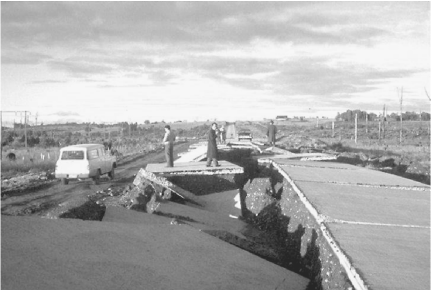
FIGURE 11.6 This picture shows the failure of a concrete surfaced highway due to an earthquake-induced foundation failure. This area was observed to be a marshy region. This main highway is located 6 km north of Perto Montt. The May 1960 Chile earthquake (moment magnitude = 9.5) caused the highway damage. (Photograph from the Steinbrugge Collection, EERC, University of California, Berkeley.)
