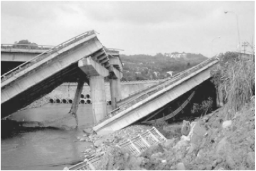
FIGURE 9.38 Earthquake-induced landslide movement that damaged the south abutment of the Shih-Wui Bridge. The landslide was caused by the Chi-chi (Taiwan) earthquake on September 21, 1999. (Photograph from the Taiwan Collection, EERC, University of California, Berkeley.)
