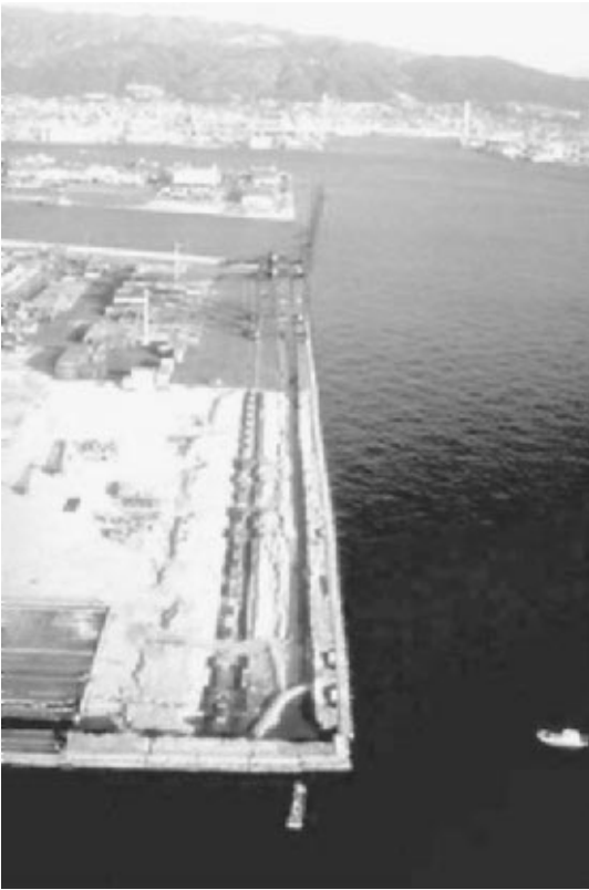
FIGURE 3.32 Retaining wall that moved outward about 2 to 3 m (7 to 10 ft), creating a depression behind the wall that was about 3 m (10 ft) deep. The cause of the retaining wall movement was liquefaction during the Kobe earthquake on January 17, 1995. (Photograph from the Kobe Geotechnical Collection , EERC, University of California, Berkeley.)
