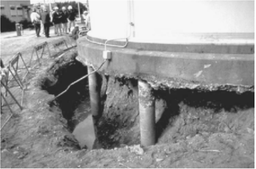
FIGURE 13.5 Storage tank supported by concrete piles. The soil underneath the tank liquefied during the Kobe earthquake on January 17, 1995. The soil around the piles was removed in order to observe the condition of the piles. (Photograph from the Kobe Geotechnical Collection, EERC, University of California, Berkeley.)
