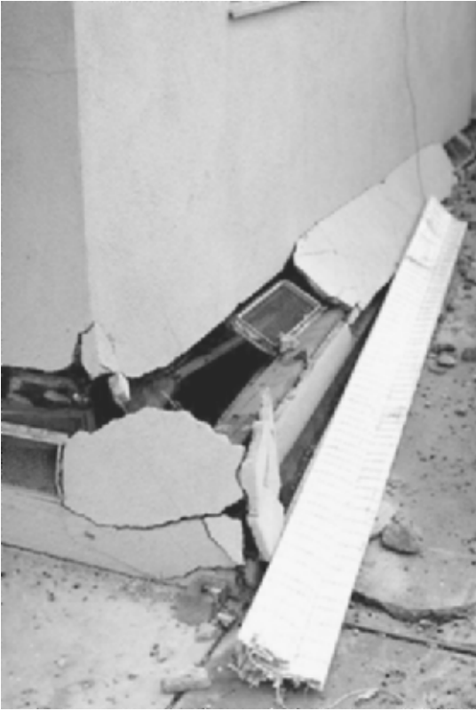
FIGURE 13.37 Sliding of house off the foundation caused by the San Fernando earthquake in California on February 9, 1971. The house is located in the city of San Fernando, near Knox and Grove Streets. (Photograph from the Steinbrugge Collection, EERC, University of California, Berkeley.)
