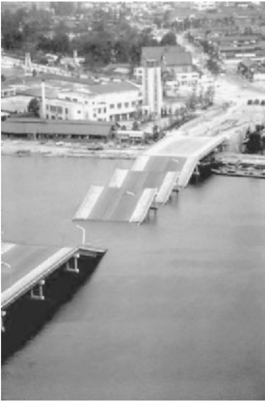
FIGURE 3.25 Collapse of the Showa Bridge during the Niigata earthquake on June 16, 1964. (Photograph from the Godden Collection, EERC, University of California, Berkeley.)
