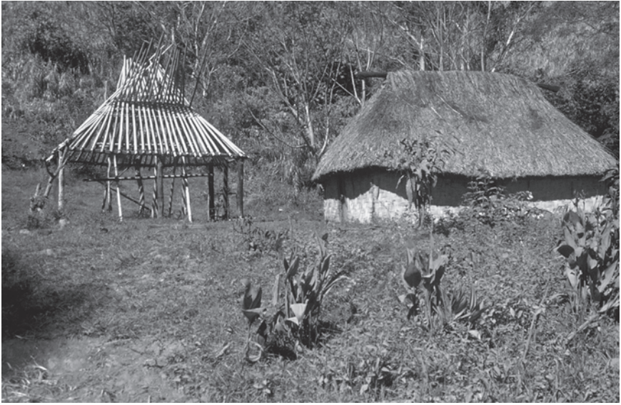
2.5 The vernacular embodying overlapping images of sustainability: House in the Sigatoka Valley on the Pacific island of Fiji under construction in 1979. Unmodified 'natural' materials characterize traditional local building using a technology of tied wood and bamboo frame, woven grass walls and thatched roof (photographer Antony Radford).
