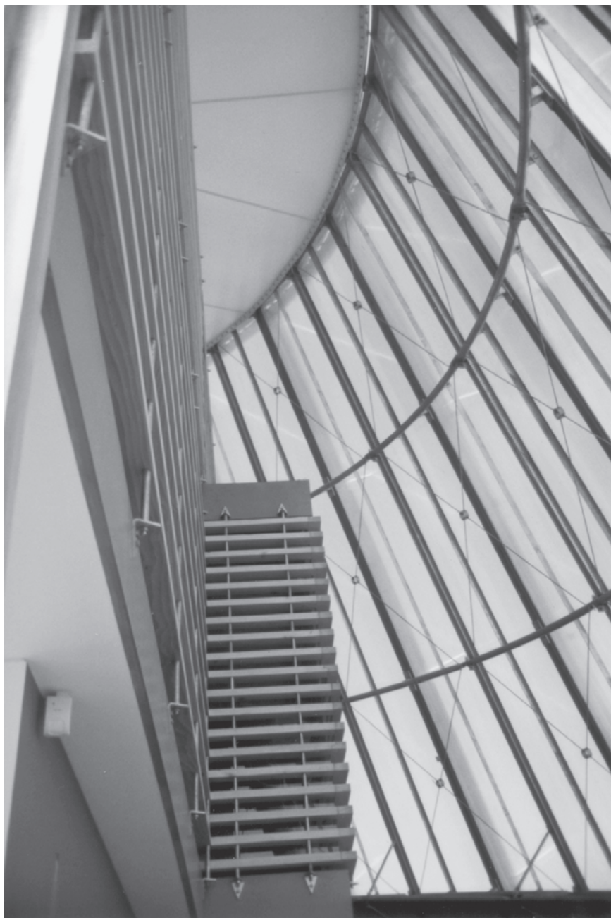
7.1 Seeking cohesion: between the inner and outer skins of the Forest EcoCentre, Scotsdale, Tasmania, 2002 (architects Robert Morris-Nunn and Associates). The brief reflected 'the close links of the community and its industry to the environment and a desire for a sustainable future' (Forest EcoCentre visitor information brochure) (photographer Antony Radford).
