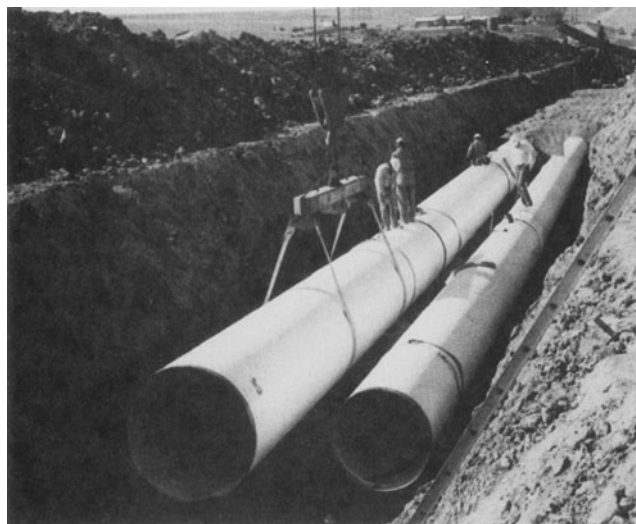
Figure 12.1.4 Parallel 60-in and 42-in diameter steel water transmission lines being installed in Aurora, Colorado. Lightweight polyethylene tape coating and O-ring bell and spigot joints helped speed installation. (Courtesy of Northwest Pipe Company.)
