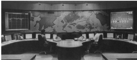
Figure 11.4.6 CAP control room. The CAP's operating features—pumping plants, check structures and turnouts—are remotely operated from the project's headquarters in north Phoenix by a computer assisted control and communications system. Cables buried along the aqueduct carry operating commands from the Control Center's computer to check structures and turnouts. The commands raise or lower gates in these structures so water can be moved through the system or delivered to users. A microwave system is used for communicating with the pumping plants. Commands are sent from the Control Center through the microwave system to pump units at the plants, starting and stopping them as needed. The communications systems also carry information from the operating features back to operators at the Control Center. The operators, who plan system operations, also monitor the system's performance and adjust it as necessary, correcting problems that may occur. The microwave and cable systems can be used interchangeably to operate the project features. If this remote operations capability is temporarily lost, each individual operating feature can be operated locally. (Courtesy of Central Arizona Project.)
