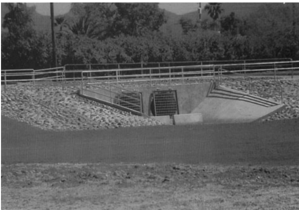
Figure 17.2.18 Culvert spillway for a detention basin in Scottsdale, Arizona. (Photograph by L. W. Mays.)
