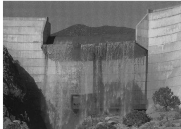
Figure 17.2.16 Spillway on Santa Cruz Lake Dam on the Rio Frijoles in New Mexico. (Photograph by L. W. Mays.)
