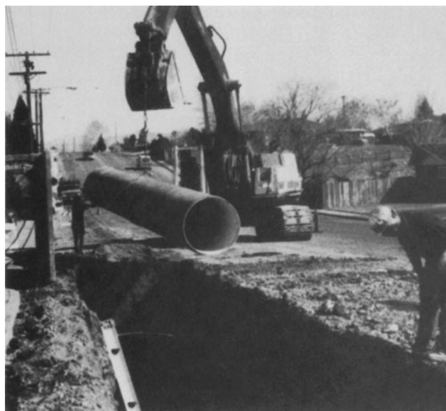
Figure 12.1.3 Cement-lined and coated steel pipe (42-in diameter) being transported to trench. (Courtesy of Northwest Pipe Company.)
