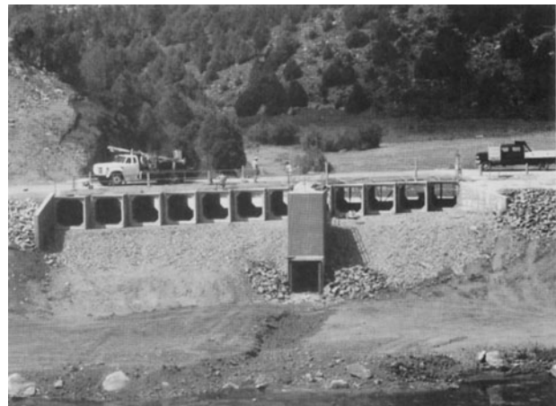
Figure 17.2.19 Culvert spillway for Dulce Reservoir dam under construction in northern New Mexico. (Photograph by L. W. Mays.)
