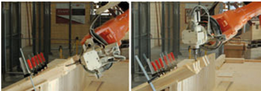
Figure 8 Positioned wooden beams and robot milling head during the production of the two joint parts.
