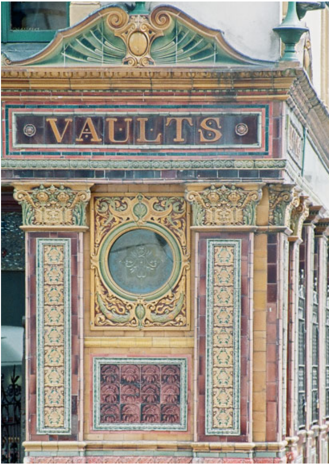
Polychromatic ceramic tiles on the facade make the pub a Belfast landmark.
