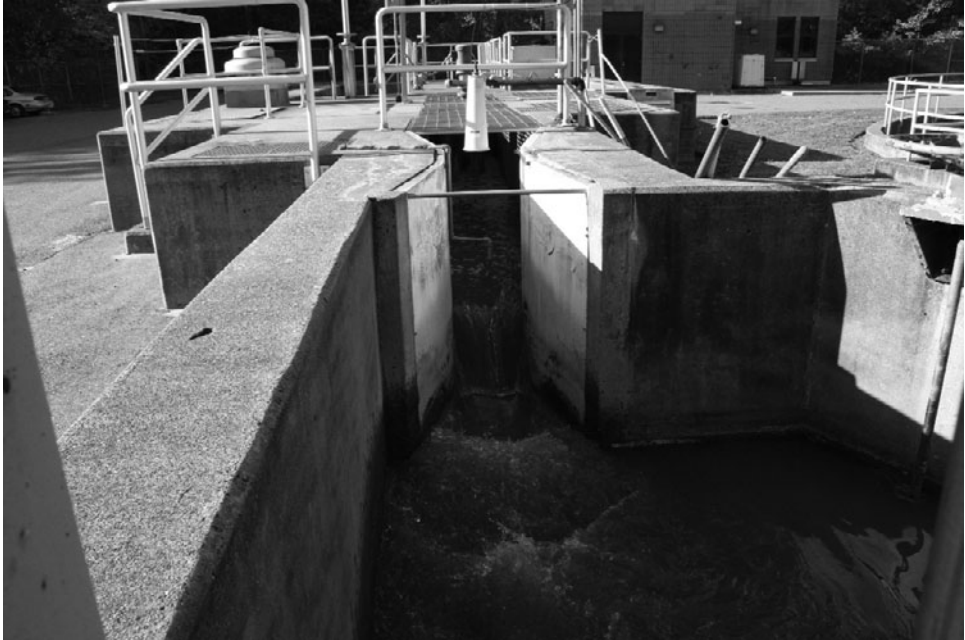
Figure 9-18. Parshall flume in a wastewater treatment system.
