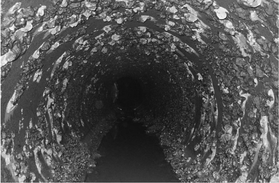
Figure 10-1. Interior of a 48-in. cast-iron water main more than 100 years old. Source: The author gratefully acknowledges Camp Dresser & McKee, Inc., and the City of New Bedford, Massachusetts, for permission to use photographs of the City of New Bedford's water distribution system. © Camp Dresser & McKee Inc. All rights reserved. Used by permission.
