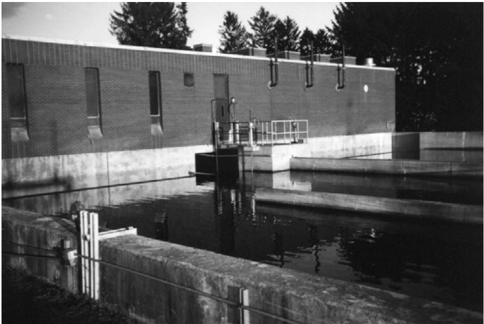
Figure 1-3. Chlorine disinfection contact tanks in a wastewater treatment system. Chlorine is added immediately prior to the tanks, allowed to mix, and then the chlorine contacts the pathogens in the contact tank.
