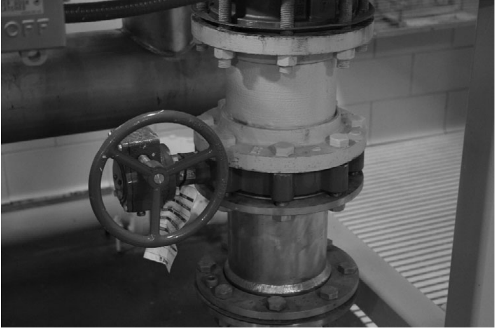
Figure 8-8. Butterfly valve installed in a water treatment system.
