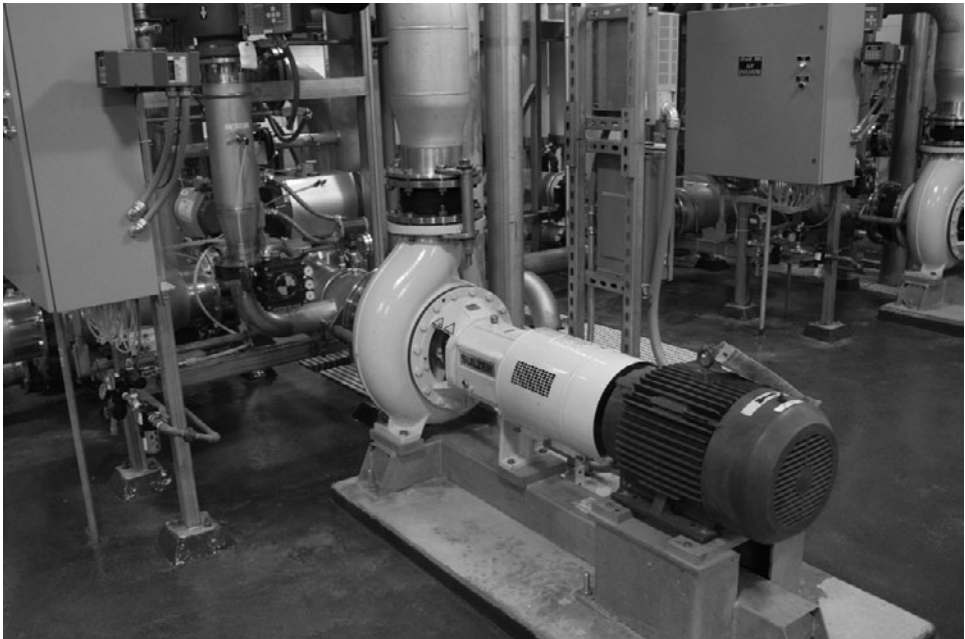
Figure 6-2. Centrifugal pump feeding an ultrafiltration system in a drinking water treatment facility.
