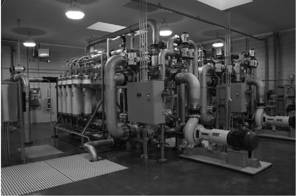
Figure 1-2. Ultrafiltration system at a drinking water treatment facility.
