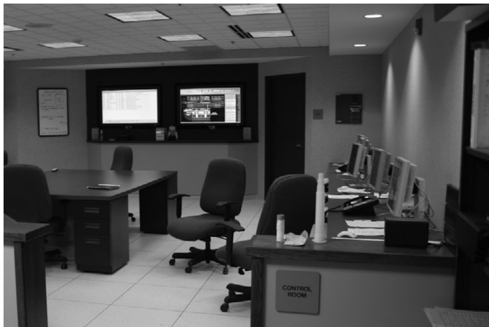
Figure 9-1. Wastewater treatment plant control room.
