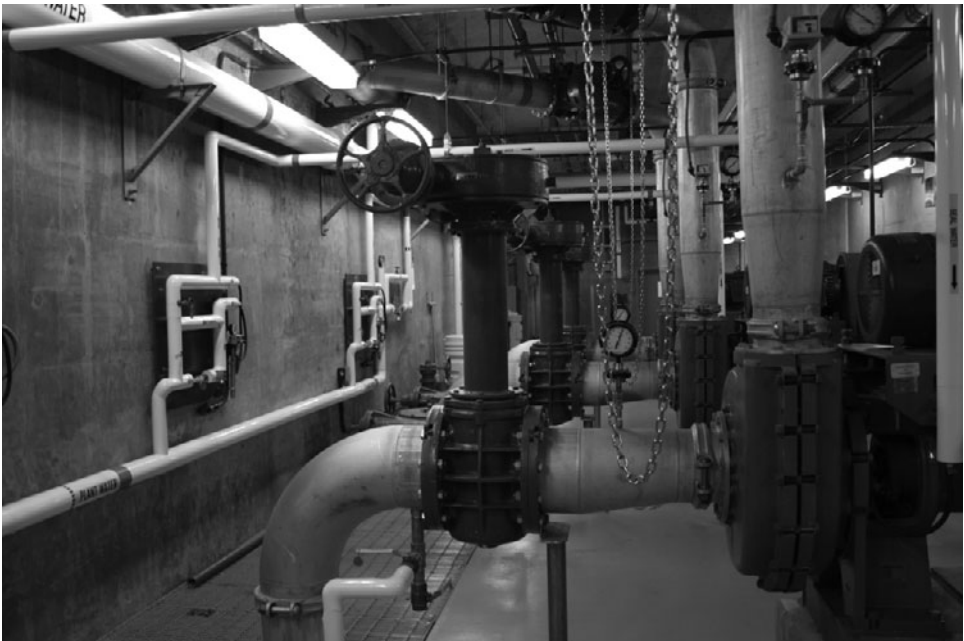
Figure 8-9. Plug valves installed in wastewater sludge pump suction lines.
