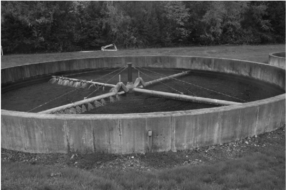
Figure 4-9. Trickling filter showing wastewater distribution arms (Problem 4).
