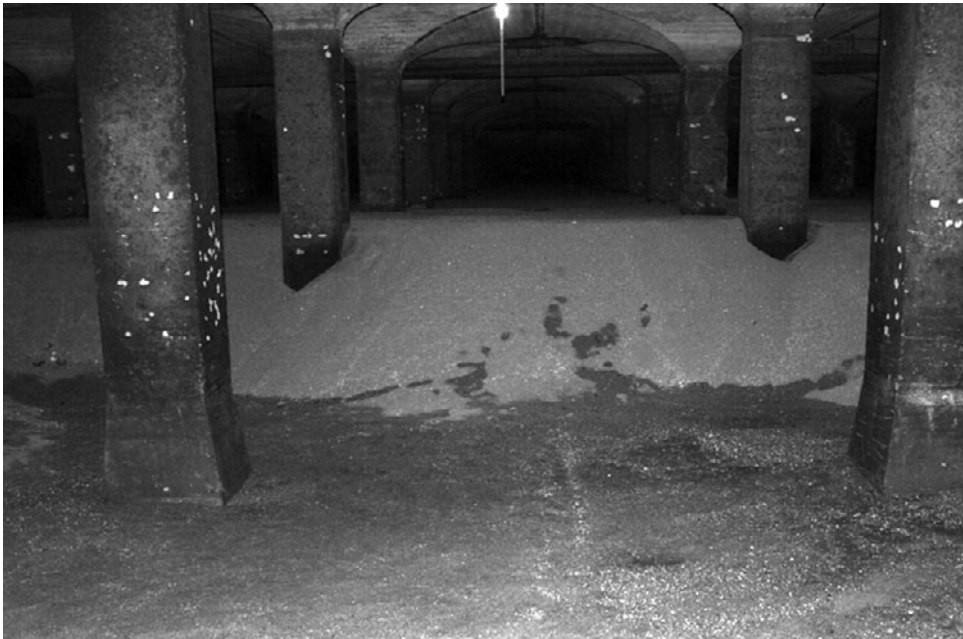
Figure 1-8. Slow sand filter used for drinking water treatment. The filter is under renovation with new sand being spread.
