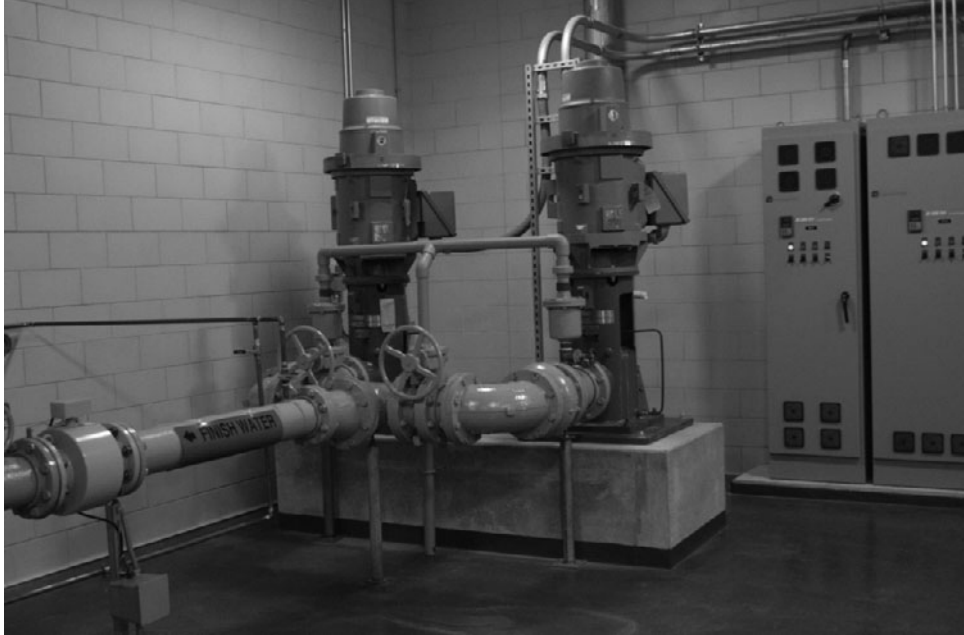
Figure 6-7. Vertical centrifugal pumps.
