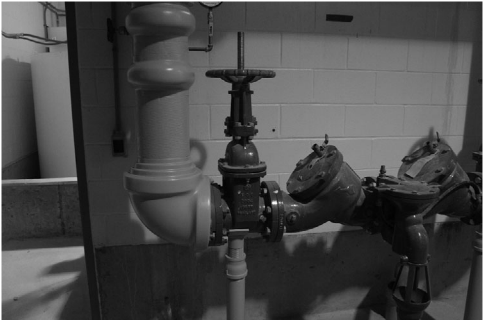
Figure 8-6. Gate valve installed in a water treatment plant.
