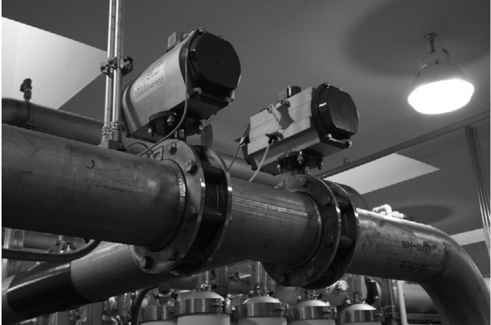
Figure 8-14. Pneumatic actuators installed on butterfly valves.
