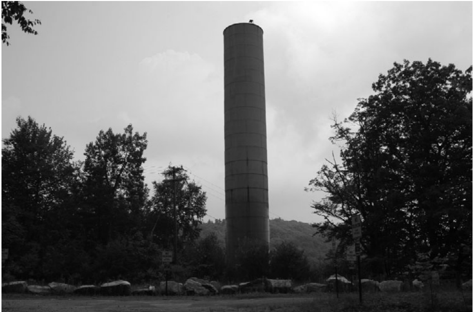
Figure 11-10. A stand pipe used to control surge in a piping system from a reservoir.
