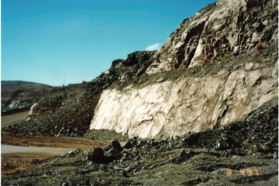
C.19 Extensive slickenside exposed in residual shale overburden of iron ore mine.
