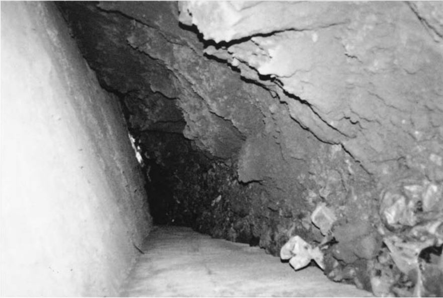
Plate 8.2 (View from right). One of the erosion cavities under spillway of Acton Valley dam.
