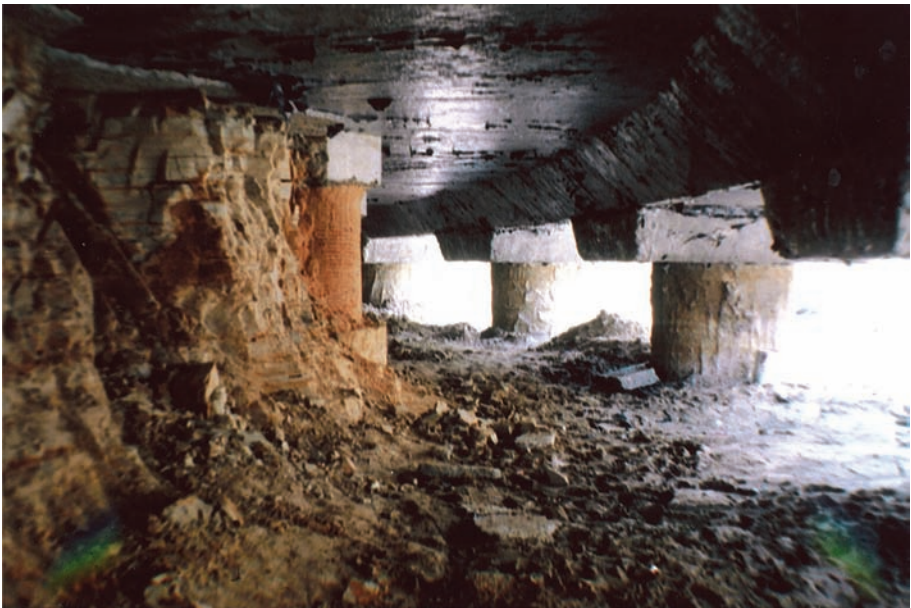
C.26 Post-construction undermining of cooling tower pond floor to relieve uplift by heave of weathered mudstone.
