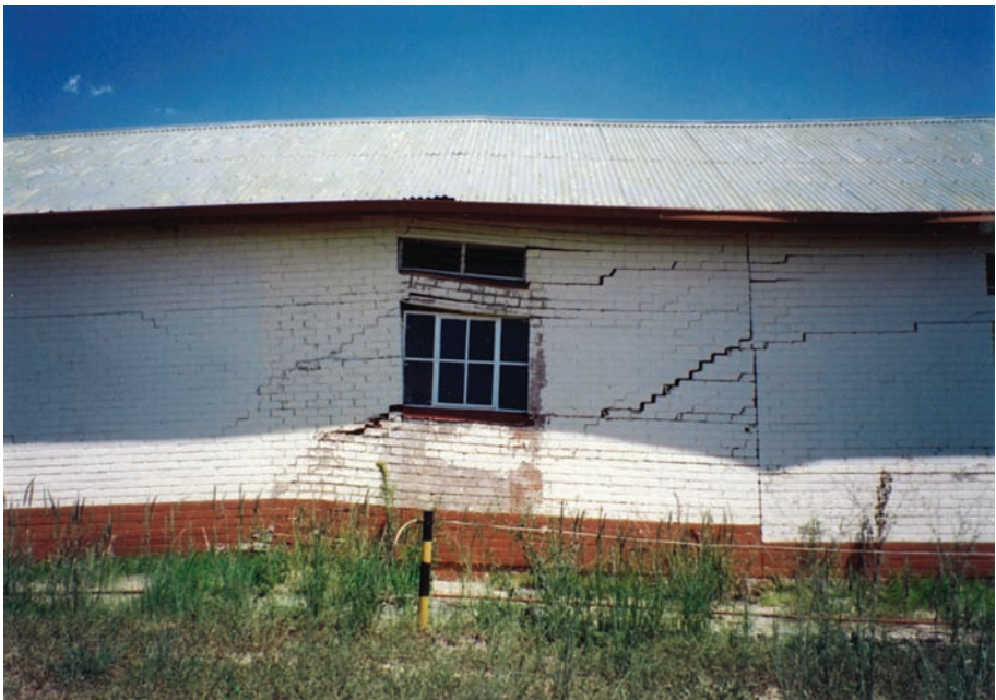
C.16 Damaged building constructed over differentially weathered dolomite.
