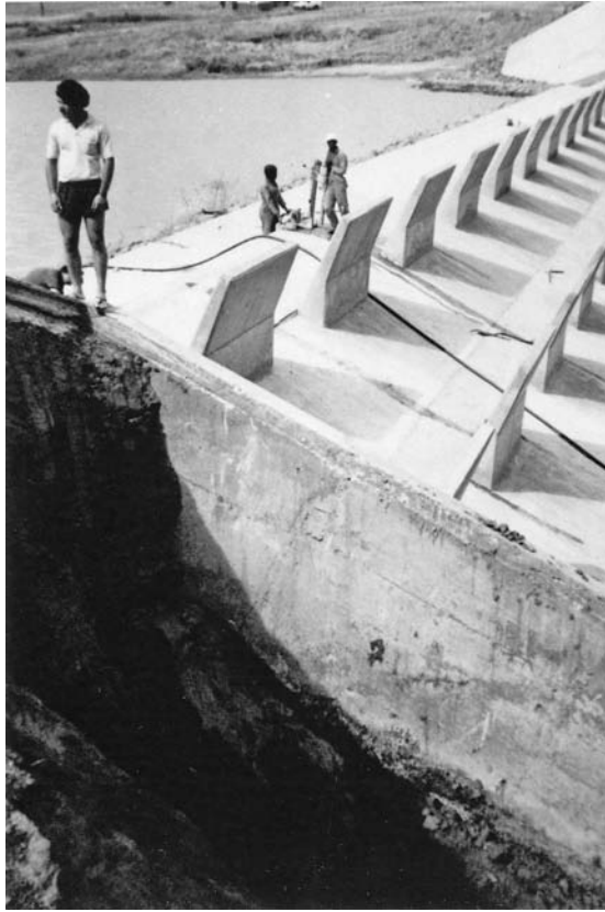
Plate 8.1 Entry points of erosion pipes in Acton Valley dam.
