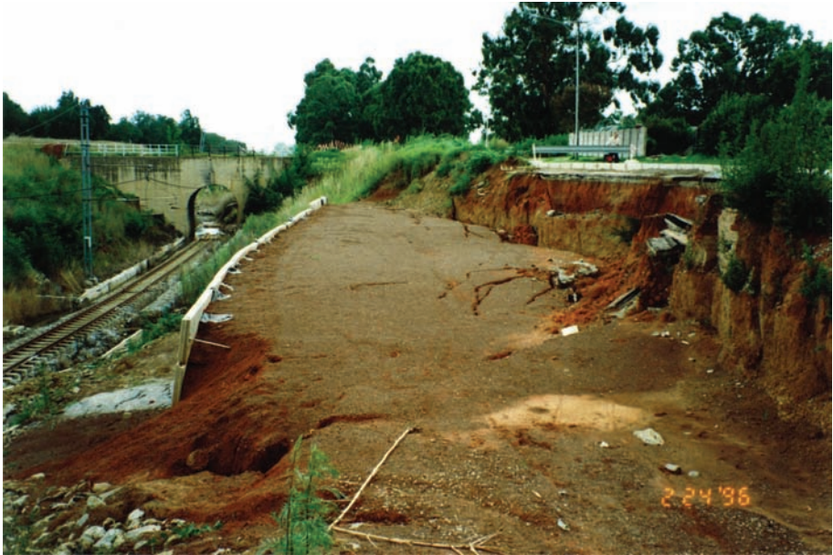
C.31 Abortive attempt to remediate failure of cut in residual andesite.
