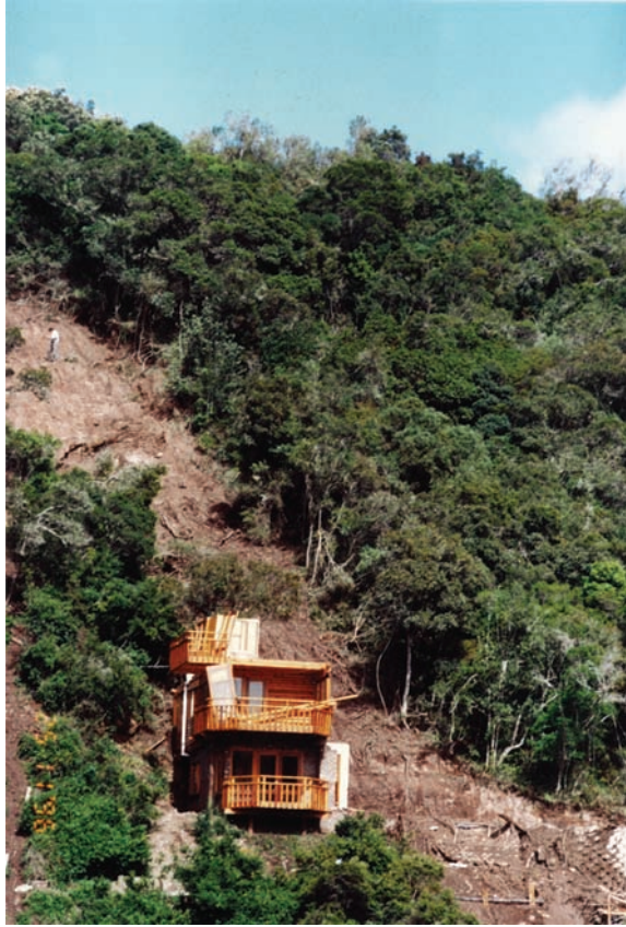
C.27 Shallow slide in residual shale slope cut into to found house.
