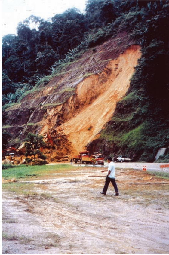
C.29 Failure of slope cut in residual granite in Malaysia.
