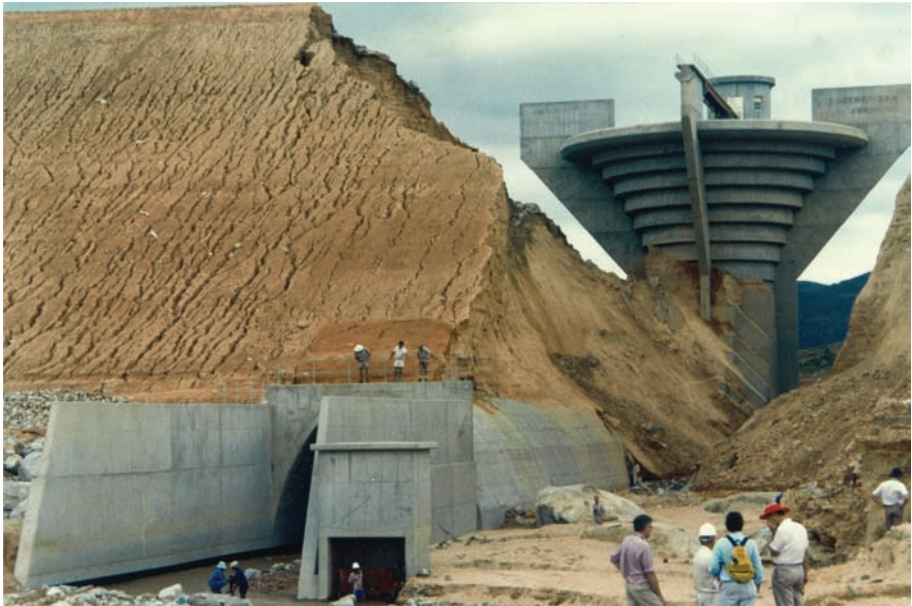
C.18 Piping failure on first filling of rolled earthfill dam.
