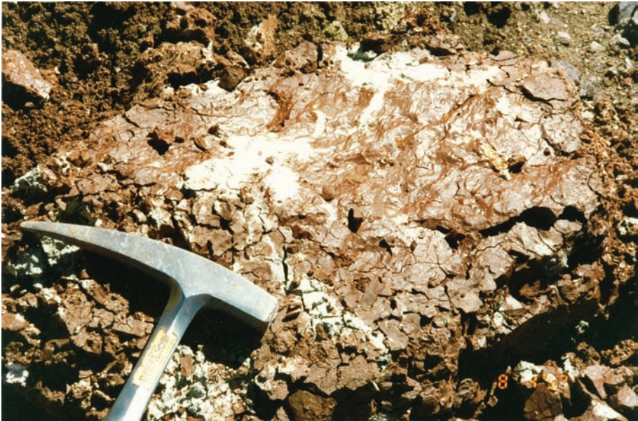
C.20 Slickenside forming part of failure surface in road cutting.
