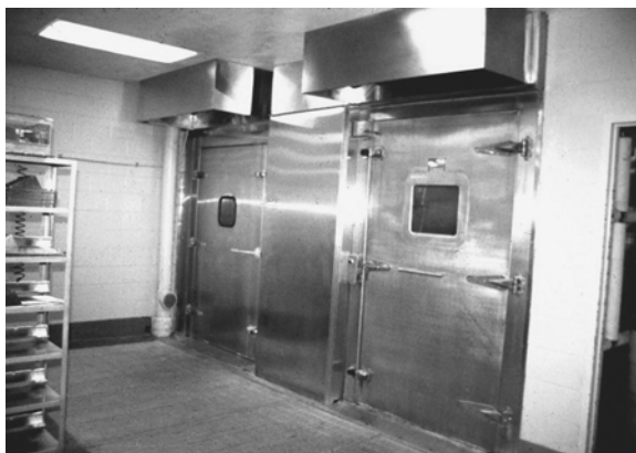
Figure 8.20 A view of a pair of batch-type cage and rack washers from the clean side of the cage sanitation area that are pit mounted to make the washer floor level with the room floor. Note the exhaust fume hoods at the ceiling and the grate-covered pit in front of the washers.
