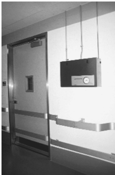
Figure 8.15 A corridor in an animal facility showing extruded solid aluminum bumper guardrails at two levels to protect the walls and the door. If only one guardrail is to be used, the lower one may provide the most protection from the widest variety of mobile equipment. Note that the rail extends further out from the wall in one location to protect wall-mounted equipment that protrudes further from the wall than the typical rail mounting of 3 in from the wall.
