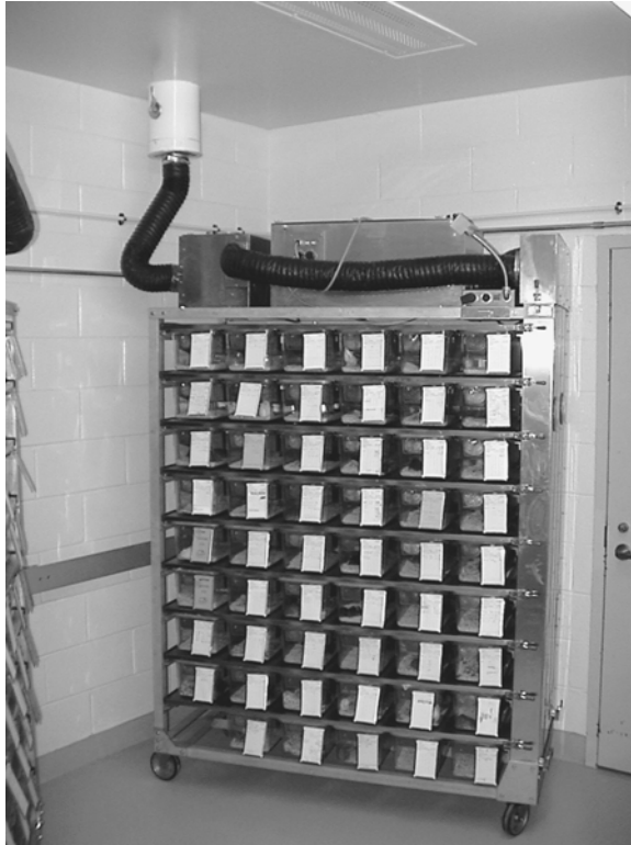
Figure 8.16 An individually ventilated microisolation cage rack with the cage exhaust filter and fan unit connected directly to the room exhaust at the ceiling, which minimizes odors in the room. The supply and exhaust fan and filter units are situated on the top of the rack. Note the extruded aluminum rail protecting the wall at the left side of the photo.
