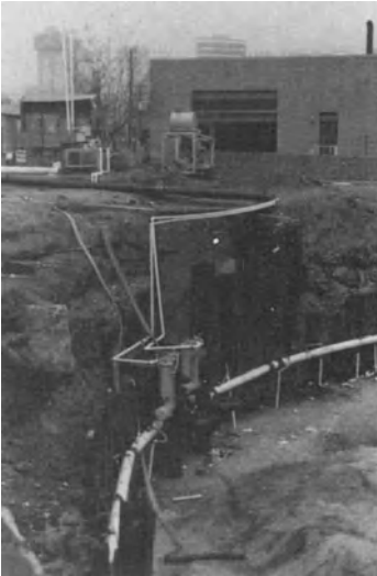
Figure 12-5g Manifold System Connected to Vacuum Chamber.
