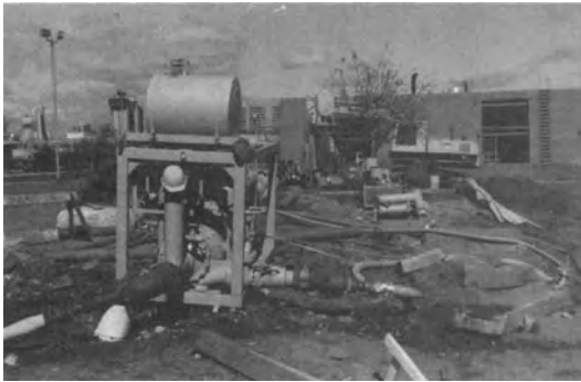
Figure 12-5h Gasoline-Driven High-Pressure Water Pump.
