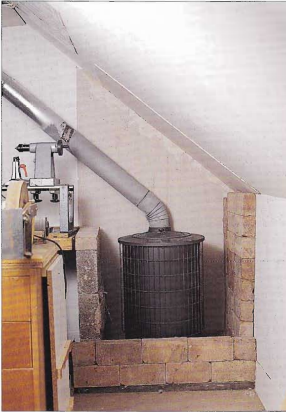
ABOVE! A heating solution that not only keeps the workshop warm, it keeps it tidy
