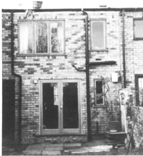
Fig. 12.15. View of the garden-facing facade of a renovated terraced house in Cambridge.
