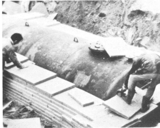
Fig. 7.2. Insulation of the Danish Zero Energy House thermal store.
