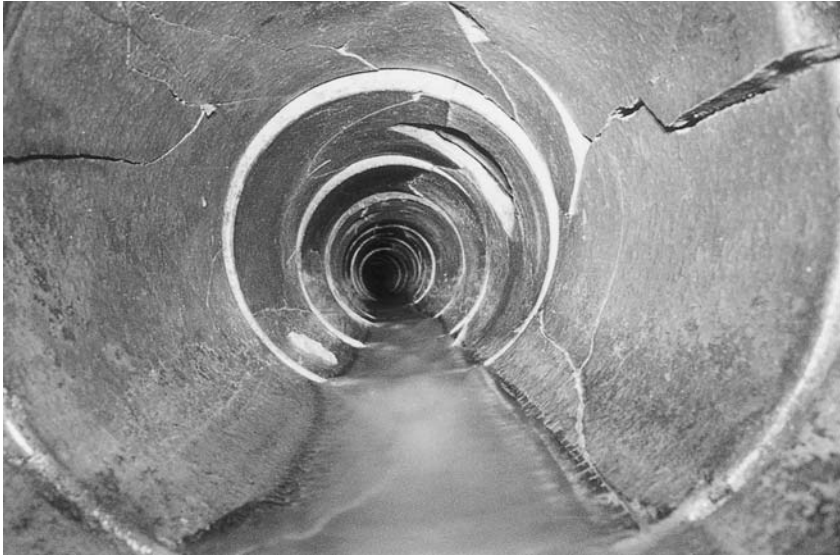
Fig. 18.2 CCTV image of a sewer in poor condition (courtesy of Telespec Ltd, Guildford)
