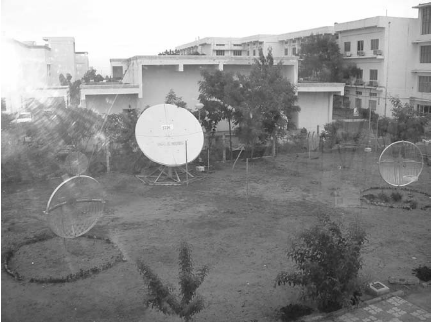
Figure 5.3 Software Technology Park of India (STPI) earth station.
