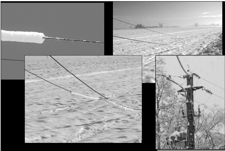
Figure 1. Damages on electric line due to wet-snow accretion on wires.
