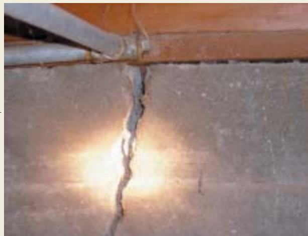
Foundation cracks like this one, caused by expansive soils, can cause serious damage to buildings that is expensive to repair.
