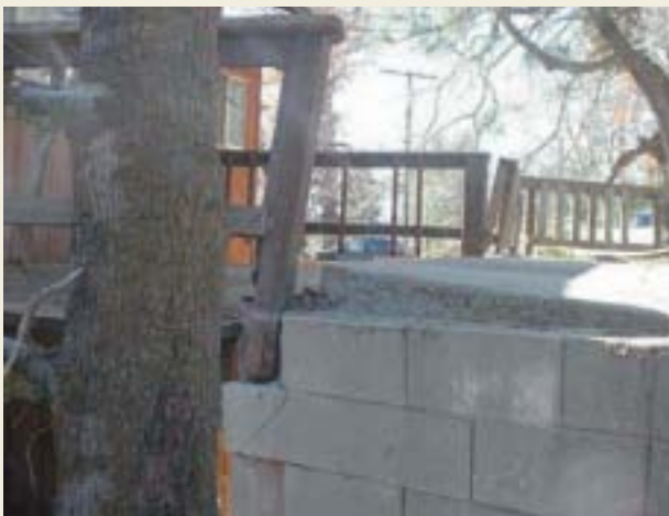
The concrete driveway slab here has been heaved upward by expansive soils, also causing damage to the adjacent railing and retaining wall.
