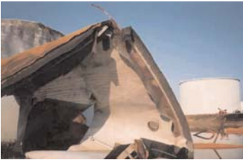
Example of a damaged pontoon after an internal explosion. This is why every means of fighting rimseal fires from the wind girder with portable equipment or from the ground, via fixed or semi-fixed systems, should be in place. Firefighting from the ground level using monitors should not be used due to the possibility of tilting the roof.
