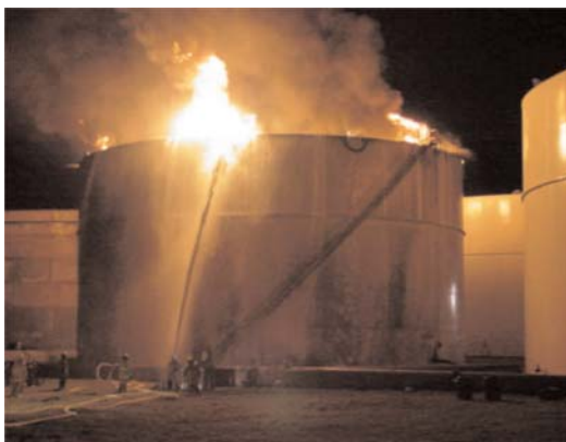
Fires at the vents are very difficult to tackle. This 95 ft (29 m) gasoline tank fire was extinguished by using foam and three of the vents were 'shot out' utilizing dry chemical (Hydro-Chem™ type).
