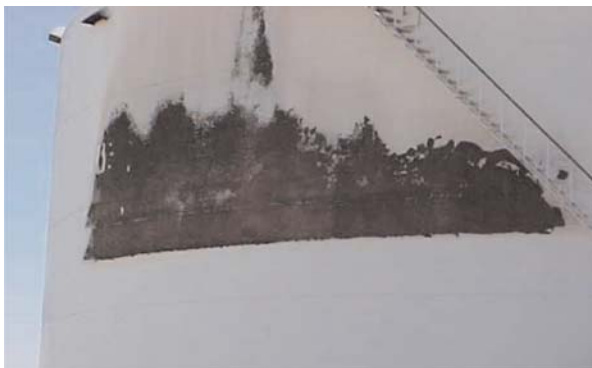
Signs of an internal rimseal fire that ignited after this tank was exposed to radiant heat from another tank fire.
