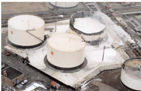
Example of partial fold-in of a tank shell. The liquid level is well visible as the product kept the paint cool and intact.
