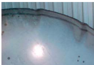
Damaged tank compartment joint
