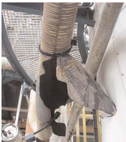
Pipe ruptured due to overpressure.
