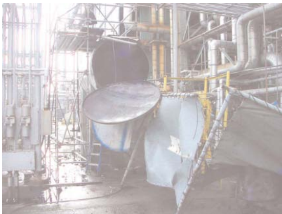
The insulated flat-head horizontal cylinder failed due to overpressure.
