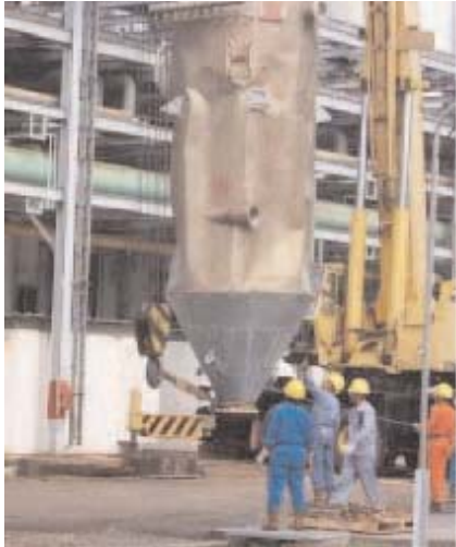
Damaged cyclofilter being removed for repairs.
