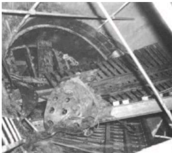
Figure 13 This picture was taken through the manway of a large vacuum tower. The trays had been upset during a shutdown of the vacuum section of this crude unit. Pump difficulties delayed pumping out the vacuum tower bottoms. Hot primary tower bottoms were inadvertently leaking into the vacuum tower during this period. At the same time, the furnace was being steam purged into the vacuum tower. Condensate from this purge contacted the hot oil in the tower and flashed into steam, causing the serious internal damage.
