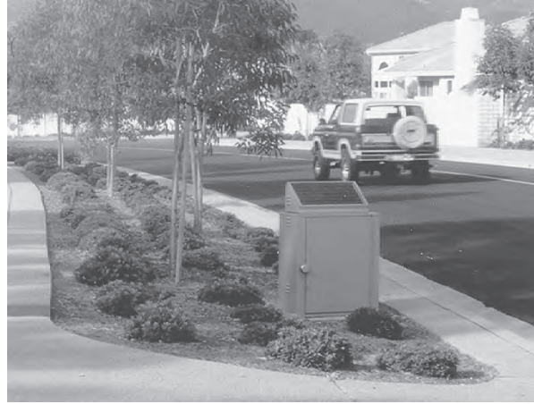
Figure 4.28 An early solar irrigation controller with an inverter to provide 110V AC power to standard valves. (Photo: Photocomm/Golden Genesis Co.)
