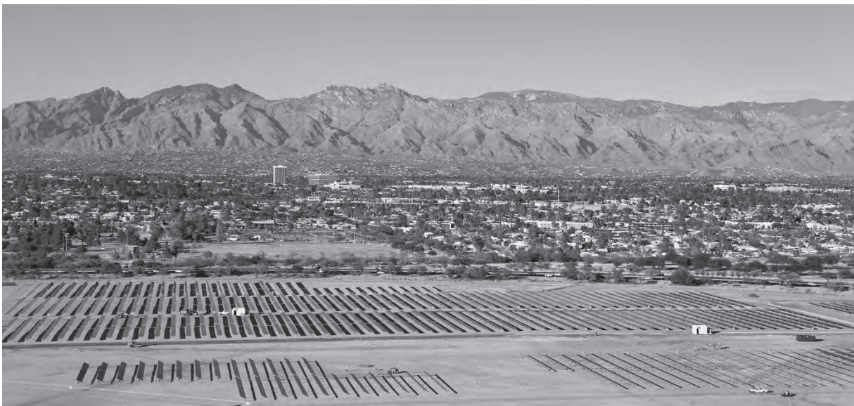
Figure 7.2 PV panels cover 170 acres at Davis-Monthan Air Force Base, Tucson AZ, the largest Department of Defense solar installation. The US military is transitioning to alternative energy far faster than are US politicians. Siting a huge “energy farm” next to a dense user community is the only time such vast centralized features make sense—and in most places, it would likely be opposed by the adjacent residents. (US Air Force photo: 1st Lt. Sarah Ruckriegle.)
