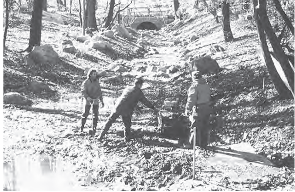
Figure 4.14 Tons of accumulated sediment were removed from Sweet Brook and used to fertilize the restored banks. (Project: New York City Department of Environmental Protection. Photo: Dean Cavallaro.)
