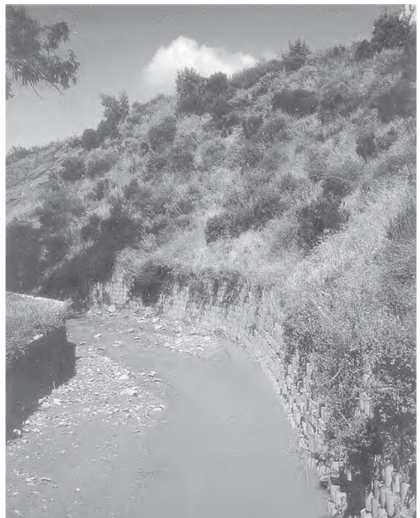
Figure 3.12a, b Greenwalls can reduce the “footprint” or horizontal extent of a high bank by steepening it. This approach protects Crystal Cove State Park (CA) from increased upstream runoff—shown during (a) and after construction (b). (Project: California State Parks, Steve Musillami. Photo: Alan Tang.)
