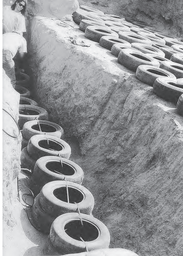
Figure 6.16 Check dams reuse waste tires to stabilize an arroyo in Arizona. Tires in the trench form a footing for the dam at the upper level. (Project and Photo: Stuart Hoenig and Joshua Minyard.)
