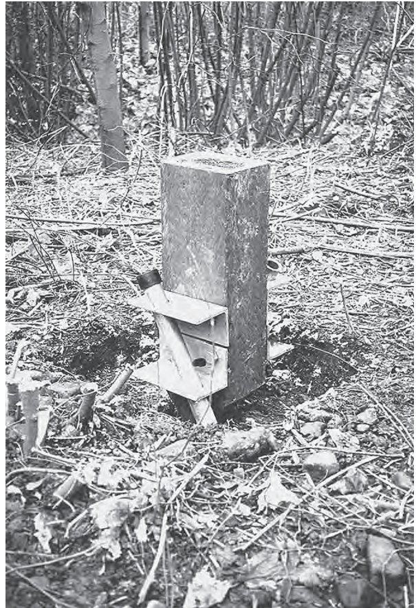
Figure 6.18 Recycled plastic lumber piers support decks along the Upper Charles River near Boston. Metal “pinned foundations” cause almost no site disruption and can be removed or adjusted easily. (Project and Photo: Carol R. Johnson and Associates.)
