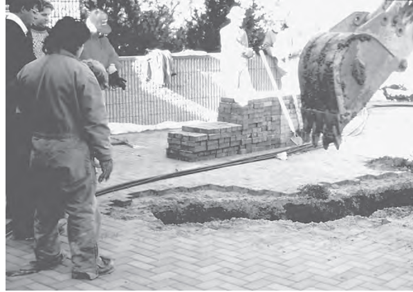
Figure I.9 Interlocking pavers set on sand are easily removed and replaced for utility access, saving energy, cost, and waste. Some pavers also permit water infiltration. (Photo: Courtesy of Interlocking Concrete Pavement Inst. / David R. Smith.)
