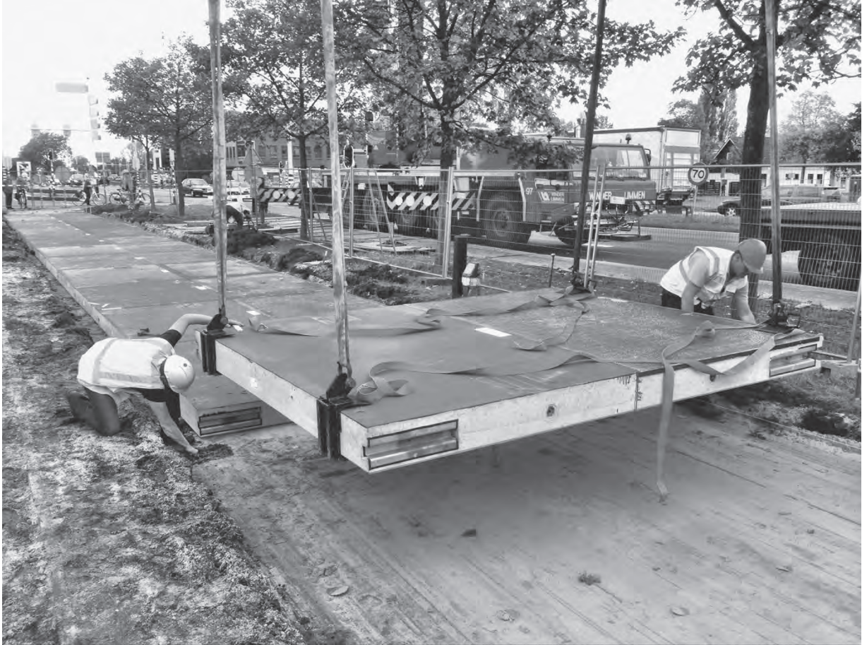
Figure 7.5 Large modular PV panels are placed for a bike and walking path that generates energy in Holland. (Product and Photo: SolaRoad Netherlands [courtesy photo].)
