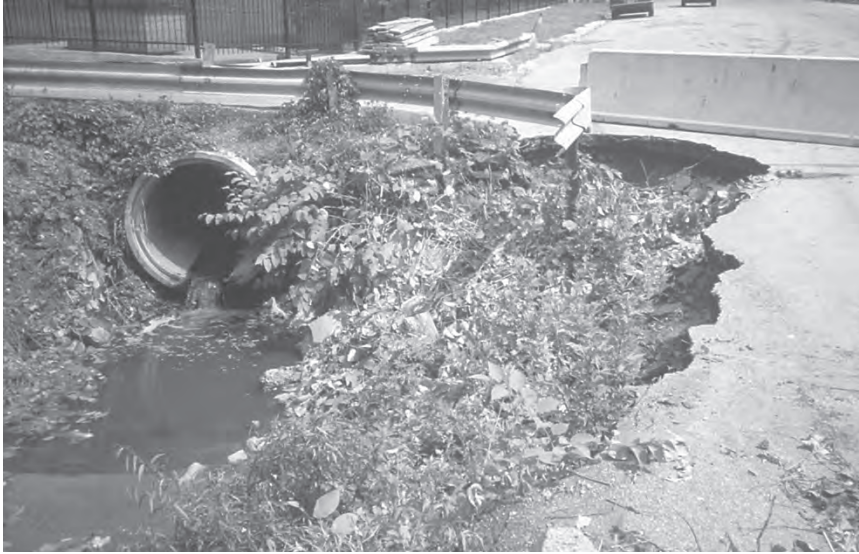
Figure 4.16 Erosion undercut pavement at Maguire Avenue and prevented plants from re-establishing. (Project: New York City Department of Environmental Protection. Photo: Dean Cavallaro.)
