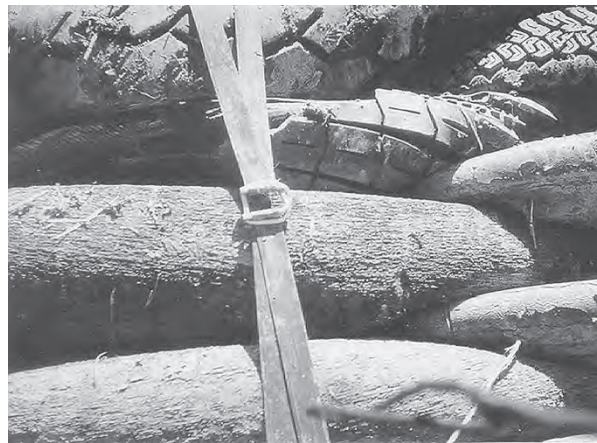
Figure 6.17 Strapped in place, tires form a strong, flexible structure that traps sediment and eventually supports plants. Some systems incorporate live staking. (Project and Photo: Stuart Hoenig and Joshua Minyard.)
