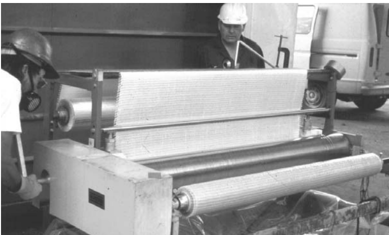
Fig. 20 Use of automated saturators is the preferred method for wet lay-up repair process. (Courtesy of Fyfe Co. LLC)
