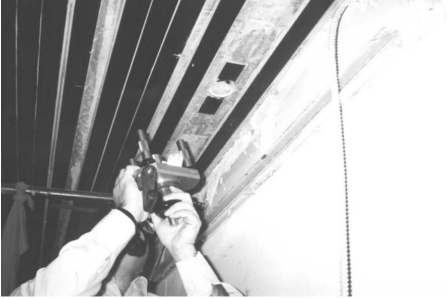
Fig. 22 Prefabricated composite laminate R/C slab applications and on-site bondline strength test. [Courtesy of Structural Composites Construction Inc. (SCCI)]
