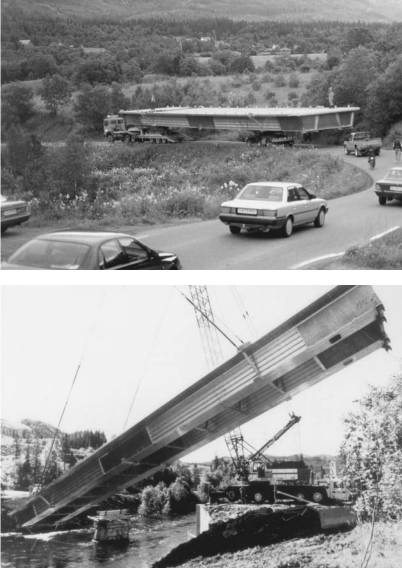
Fig. 9 The Foresmo bridge in northern Norway is an excellent example of the use of Al-Mg alloys for built-up girder systems; these photos illustrates a major advantage of replacement aluminum bridges: the ability to prefabricate the spans, (a) transport them, and (b) erect them in place quickly, minimizing the disruption to traffic.
