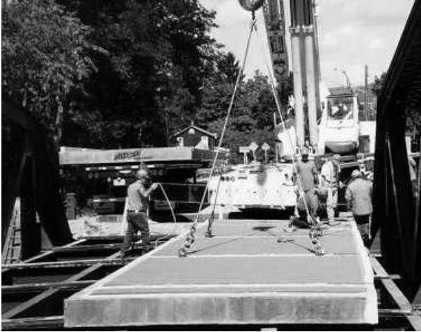
Fig. 51 Installation of all-composite bridge deck of NY 367 over Bentley Creek, Chemung County, New York (2000). (Courtesy of New York DOT, Region 6, Hornell, NY)
