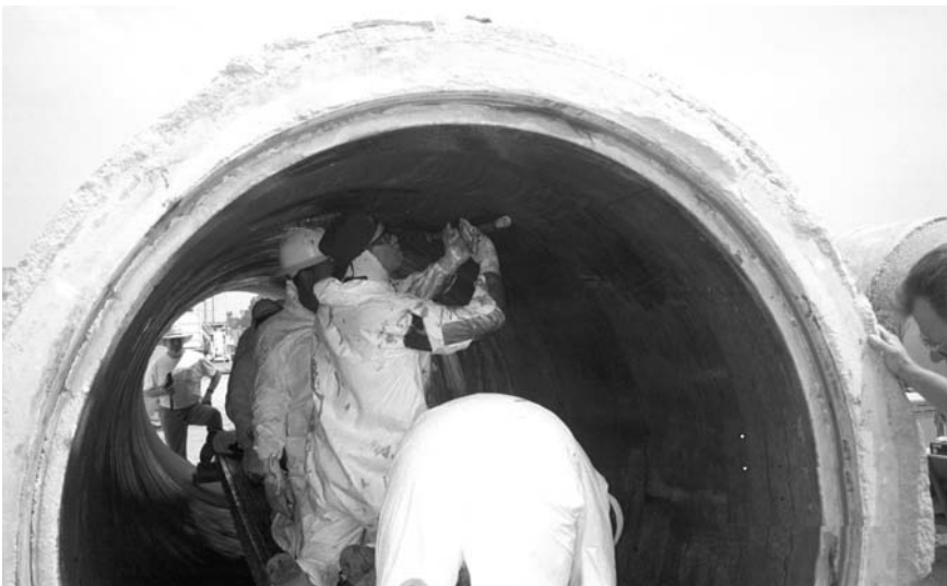
Fig. 12 Strengthening of reinforced concrete pipes using polymer composites. [Courtesy of Structural Composites Construction Inc. (SCCI)]
