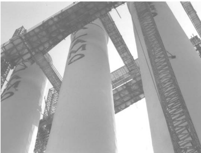
Fig. 9 Structural strengthening of chimneys using polymer composites. (Courtesy of Fyfe Co. LLC)
