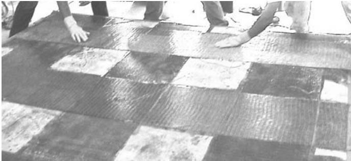
Fig. 11 Structural strengthening of unreinforced concrete slab-on-grade using polymer composites. [Courtesy of Structural Composites Construction Inc. (SCCI)]
