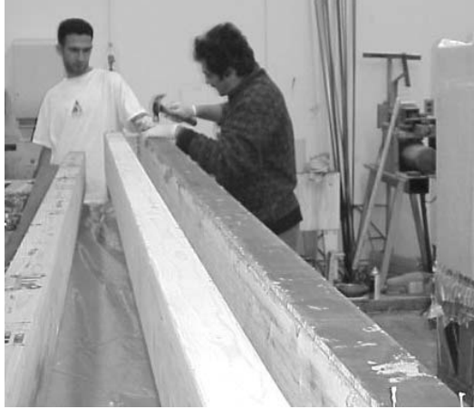
Fig. 15 Structural strengthening of glue-lam wooden beams using carbon/epoxy sandwich composites. (Courtesy of Sigma Composites, LLC)
