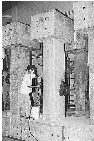
Fig. 27 Minimum radius of 0.75 in. (20 mm) for noncircular columns is required before the application of FRP composites. (Courtesy of Professor M. Haroun, University of California, Irvine)
