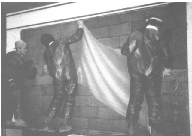
Fig. 16 Strengthening of unreinforced masonry walls using polymer composites. (Courtesy of Fyfe Co. LLC)
