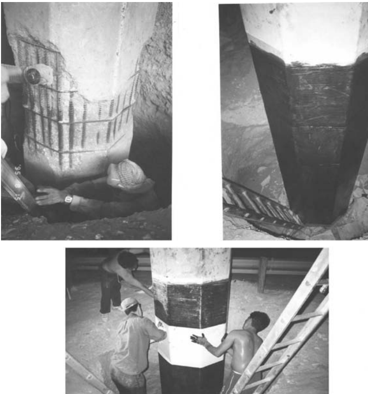
Fig. 2 Reinforced concrete corroded column repair applications using composites. (Courtesy of Sigma Composites, LLC)
