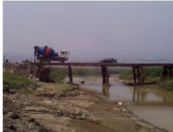
Figure 3. A bridge site that suffered liquefaction induced lateral spreading during 921 Ji-Ji earthquake
