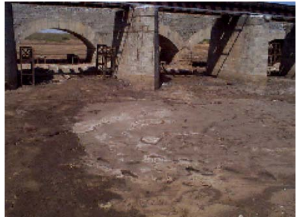
Figure 6. Liquefaction induced sand boils at the bridge site
