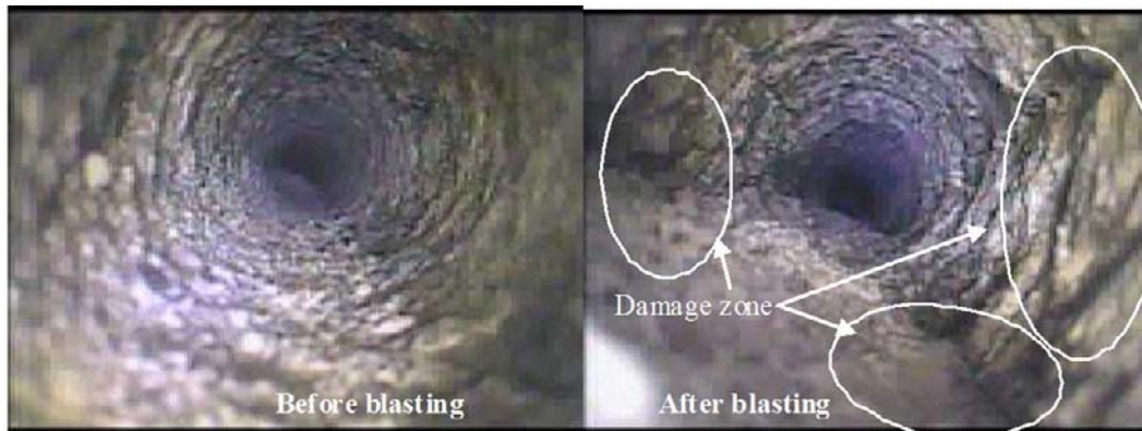
Figure 12. Images of pre-blast and post-blast inspection surveys of rock mass with acute joint orientations captured by borehole camera
