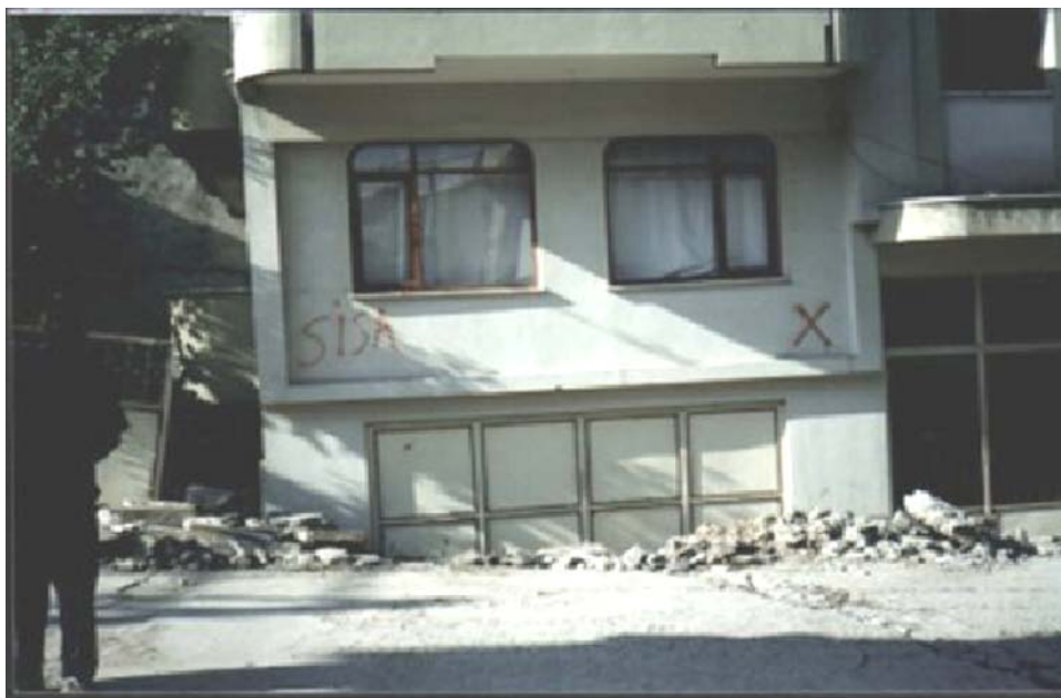
Figure 1. Punch failure of foundations
