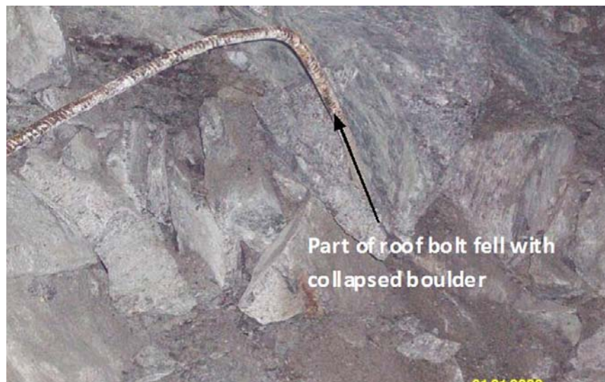
Figure 20. Roof failure due to extension of fractures beyond 3m due to repeated blast induced damage
