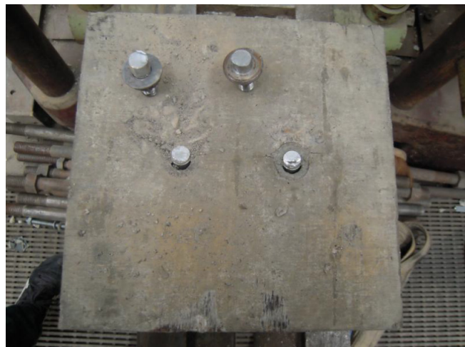
Figure 5. Shear connector fracture
