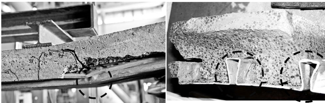
Figure 5. Buckling of the web at the starting point of the inclined bending crack.
