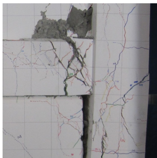
Figure 6. Damage of specimen CWPS at drift angle of -0.03rad
