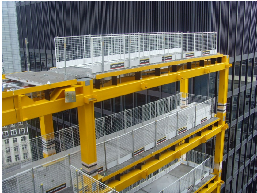
Fig. 15 - North core module, delivered as one unit (steel table, precast planks, horizontal services and edge protection)
