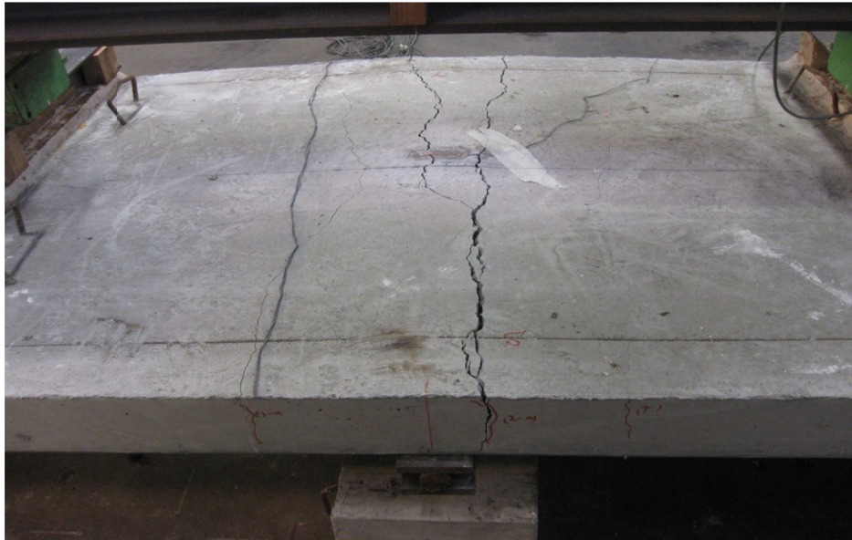
Figure 11. Excessive cracking in concrete surface at interior support in slab S1.
