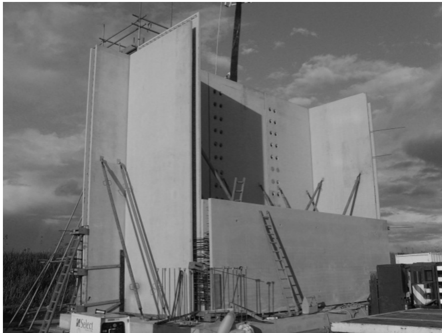
Figure 3 – Construction of ‘trial’ twinwall water-retaining tank at Laing O’Rourke’s manufacturing facility near Worksop
