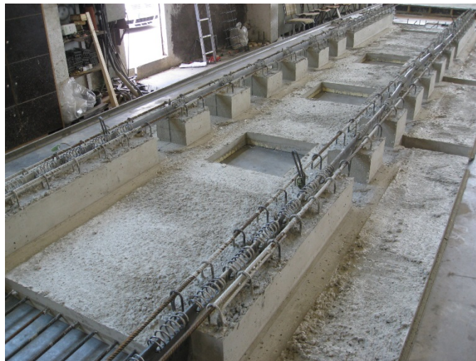
Figure 12. Manufacture of the hollow slabs with the webs reinforced with metal plate and the helically reinforced connector
