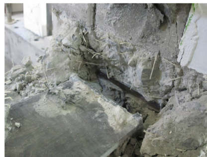
Figure 7. Fracture of steel beam of specimen CWPS (Observation after test)
