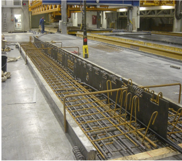
Figure 10. Manufacture of the experimental girder with web plate and the helically reinforced connector including prestressing reinforcement
