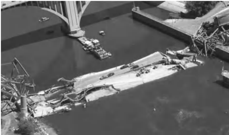
Figure 10.7 NTSB PHOTO: Collapsed Bridge Center Section (Looking Southeast)
