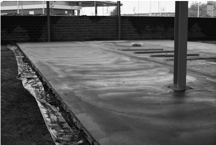
Fig. 5.33. The effect of power trowelling is to create a smooth and durable surface. There must be just the correct amount of surface laitance. Too little and the surface will remain open; too much and a thin layer may eventually spall at the surface
