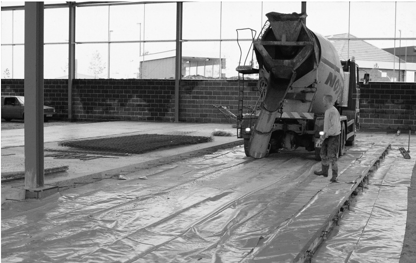
Fig. 5.23. A slip membrane has been laid and formwork has been fixed prior to concreting. The concrete truck reverses along the strip to the discharge position. Care has to be taken to avoid rutting the sub-base and disturbing the slip membrane. The mesh reinforcement cannot be installed prior to concreting as it would interfere with access
