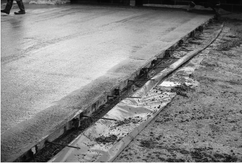
Figure 5.30. The concrete is left to set. Note the excess slip membrane material and the tie bars. Because the roof sheets are fixed and the weather is cool, there is no need to take special measures to reduce moisture loss from the upper surface of the concrete
