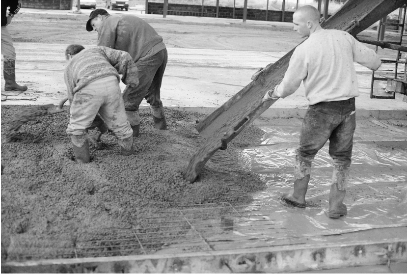
Fig. 5.24. The concrete is discharged between the formwork and, in this case, a previously constructed strip. A piece of mesh reinforcement has been installed. The concrete is discharged as close as possible to its required position and is moved by hand as required
