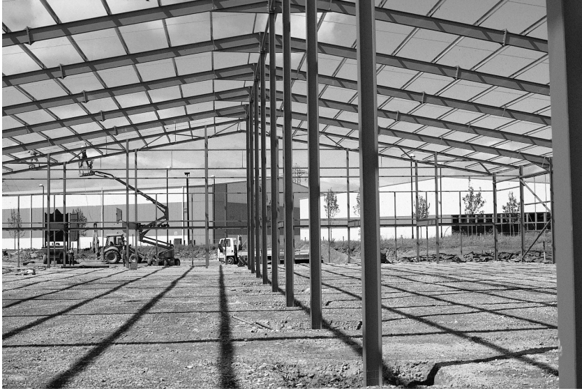
Fig. 5.19. The propped portal frame has been completed and the sub-base has been laid. Floor construction cannot start until the roof sheets have been fixed otherwise the sun could lead to rapid moisture loss from the concrete. This in turn could cause plastic cracking in the floor
