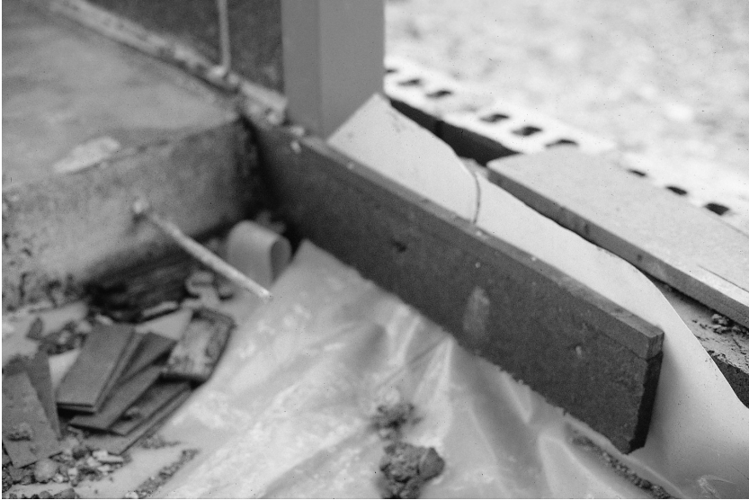
Fig. 5.35. An isolation joint is formed at the building perimeter using the compressible material shown. In this case, the floor slab is constructed right up to the internal wall without a perimeter strip. The slip membrane is brought to the slab surface to contain the moisture in the concrete during curing
