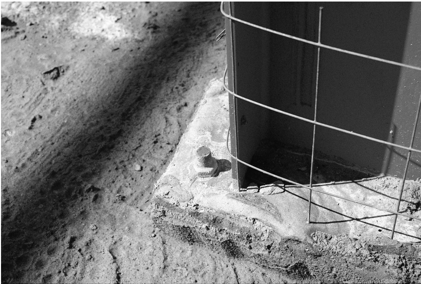
Fig. 5.21. Lightweight steel mesh reinforcement has been fixed around the prop columns through the depth of the floor slab. A baseplate has been welded to the end of the column. The baseplate has been bolted to the foundation. Wind may cause the column to develop tension so it has to be bolted positively to its foundation
