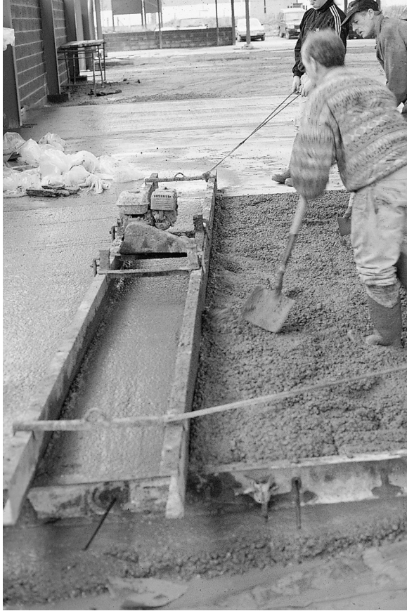
Fig. 5.27. A double vibrating beam is pulled along the formwork to compact the concrete. A member of the team ensures that there is sufficient concrete along the length of the beam. Tie bars have been inserted in holes in the formwork
