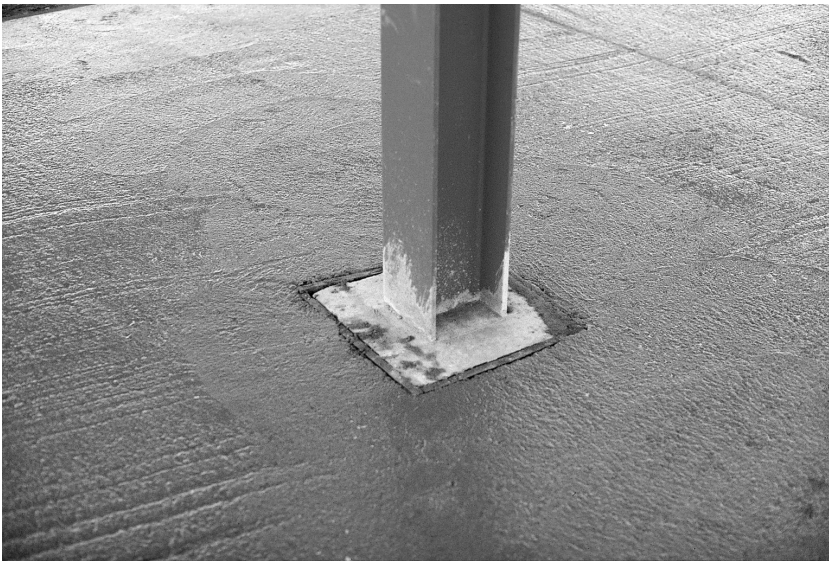
Fig. 5.31. The floor slab has been cast around an internal column. Compressible material has been fixed around the square concrete surrounding the column. The upper part of the compressible material will be replaced by a protective strip
