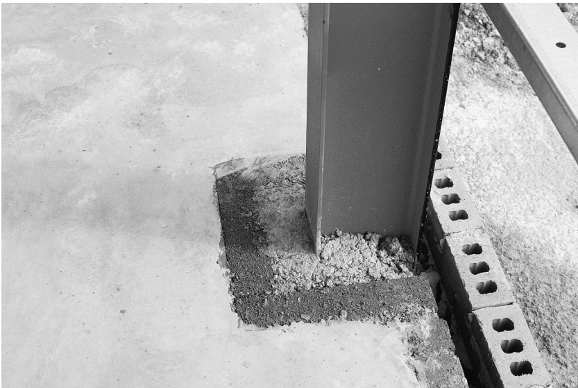
Fig. 5.36. At the external columns, the concrete block internal leaf is constructed round each column and a compressible strip is fixed to the concrete blocks prior to concreting. This isolates the floor from the internal leaf and from the main columns
