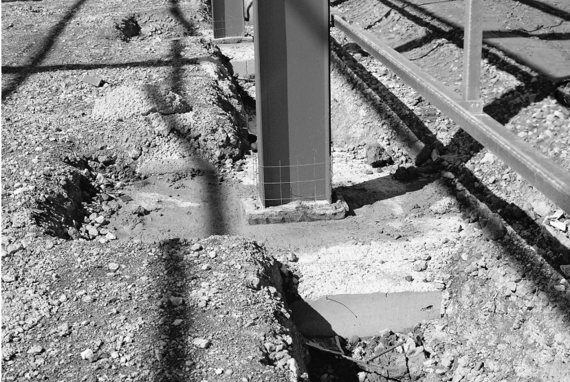
Fig. 5.20. The prop columns along the centre of the building have been bolted to their concrete foundations which are below the level of the underside of the floor slab. The floor slab will surround these columns
