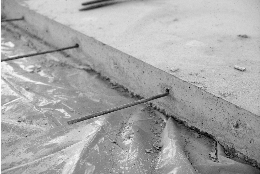
Fig. 5.34. The finished slab with the formwork removed showing the tie bars ready for the neighbouring long strip. This concrete can be used as formwork for the next long strip. Sometimes the alternate strip method is used whereby the initial long strips require formwork at each side and the intermediate strips use the previously cast concrete. In this case, one central long strip was cast using formwork at each side. All of the subsequent strips were cast using one existing concrete long strip and one side of formwork
