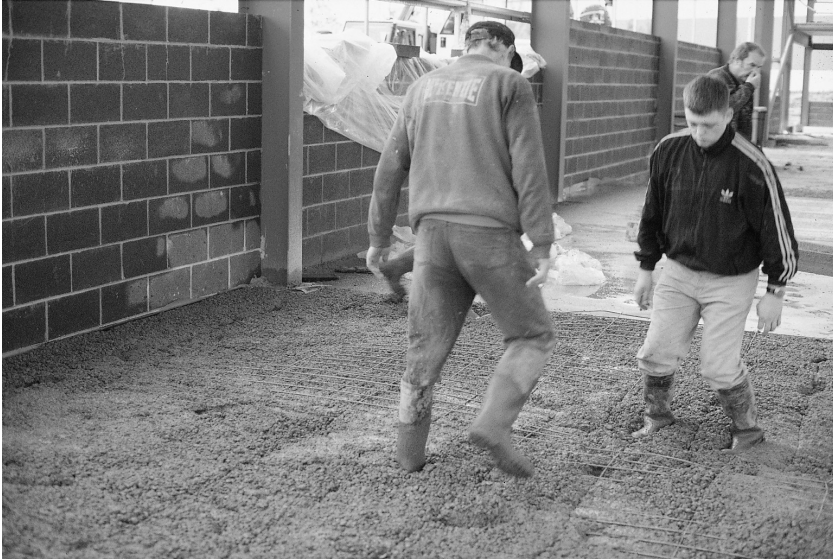
Fig. 5.26. The mesh is pressed into the concrete by members of the concrete gang walking over it. The mesh can be located with a surprising degree of accuracy by a skilled team. Care is taken to ensure sufficient overlap with neighbouring pieces of mesh. A cropping tool is on hand to deal with obstructions
