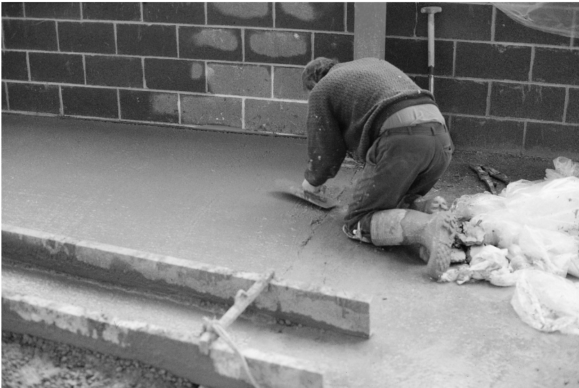
Fig. 5.29. The edges of the slab are trowelled to improve the quality of the longitudinal joint. This trowelling takes place immediately after the concrete has been compacted. Additional concrete may be placed to make up levels
