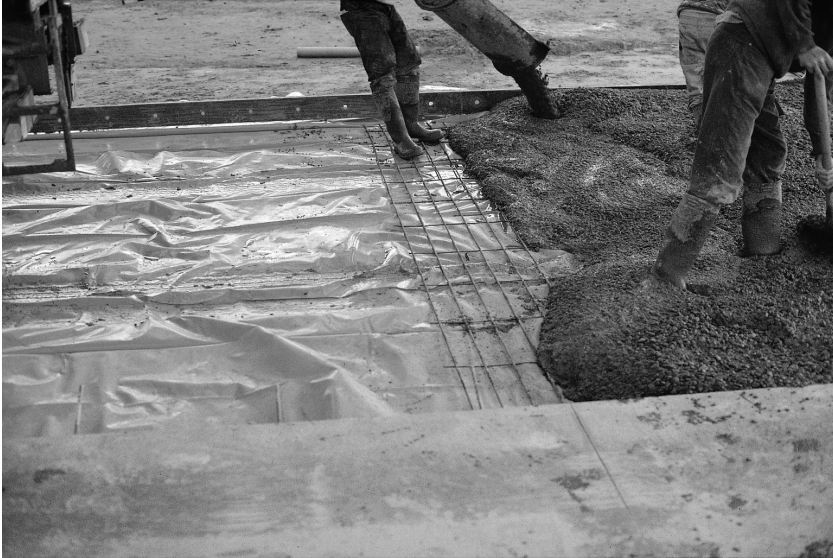
Fig. 5.28. A short length of mesh is placed near the underside of the concrete to act as the tie at a transverse tied joint. The main mesh reinforcement near the upper surface of the concrete is stopped short of the tied joint. Note that the main reinforcement runs normal to the longitudinal long strip direction. A transverse groove has already been cut in the neighbouring bay to complete the tied joint
