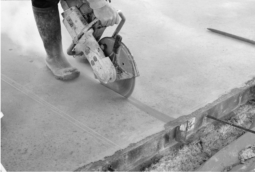
Fig. 5.37. A 3 mm wide by 40 mm deep groove is cut into the concrete using a hand held saw. Care has to be exercised to ensure a straight cut. The reduction in cross-sectional area and second moment of area ensures that cracking occurs here. Note that the main mesh is stopped here and a shorter piece having its main bars running along the line of the cut contributes to the weakening at such joints
