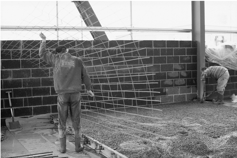
Fig. 5.25. A standard size (4.8m × 2.4m) piece of mesh is ready to be placed in the fresh concrete. The mesh is orientated so the main reinforcement is in the longitudinal direction. The mesh is positioned vertically, then allowed to rotate onto the surface of the concrete
