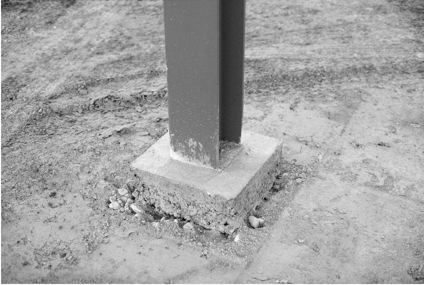
Fig. 5.22. Concrete has been cast around the column through the depth of the floor slab. A strip of compressible material will be fixed around the perimeter of this concrete to the full depth of the floor to ensure that the floor and the structural frame can move independently of each other
