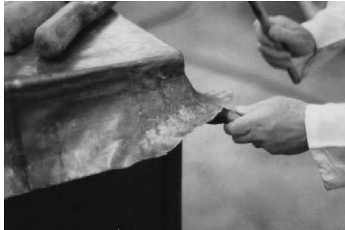
Figure 4.18 Sheet lead work (Reproduced with the kind permission of the Lead Sheet Association)
