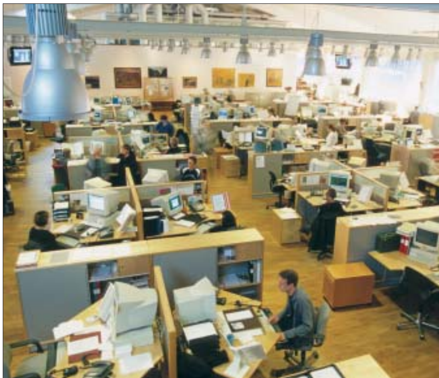
Figure 21 Industrial style luminaires used in high office space
